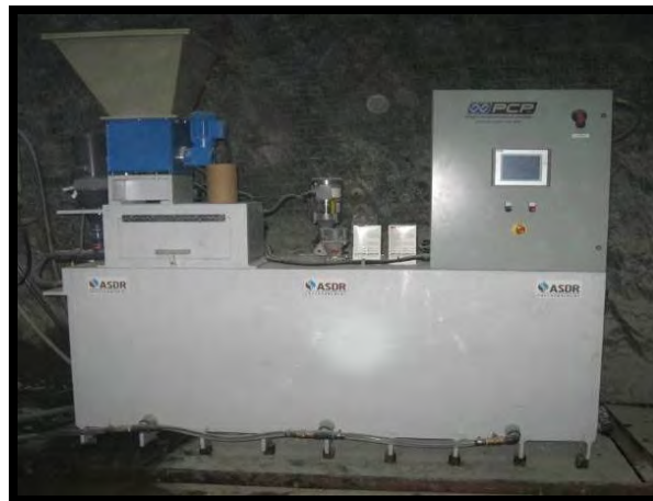
Picture 9: Polymer preparation unit
