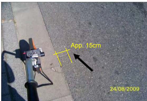
Figure 4. Lateral crack at the edge
