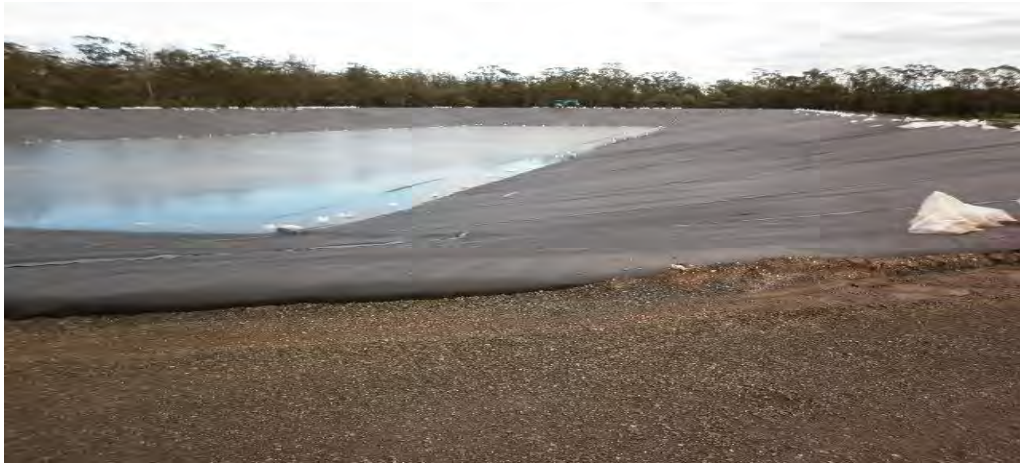
Fig 2. Typical HDPE lined CSG water pond
