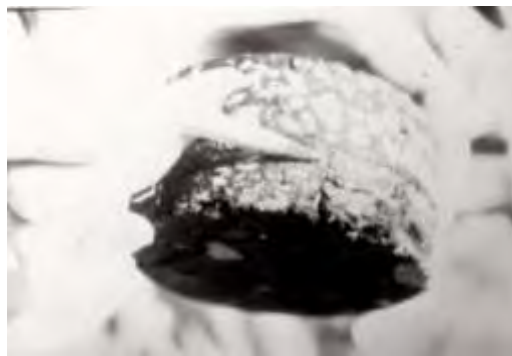
(e) Asphalt pavement core showing the crack-arresting feature offered by the geotextile with the new overlay placed above
