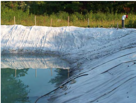
Figure 14. The GCL isn't working. No cover soil ! GCL left exposed for weeks/months. Incredible ! Last item in procedure, "place cover", not done.
