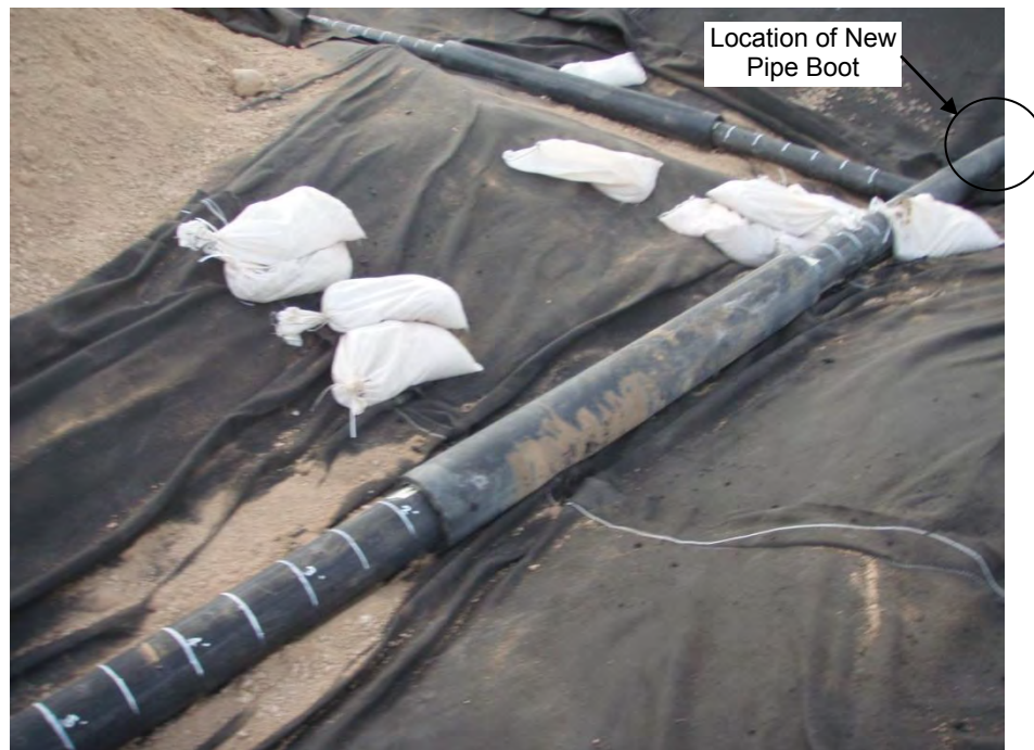
Figure 7. Leachate pipes and pipe sleeves configuration prior to geotextile wrap, pipe boot welding and local trench backfilling.
