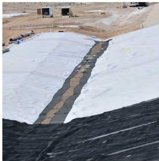
Figure 5. Photo of secondary 60-mil conductive white-surfaced HDPE geomembrane with LCRS piping and gravel drain. Geonet drainage layer (black) is installed over the piping.
