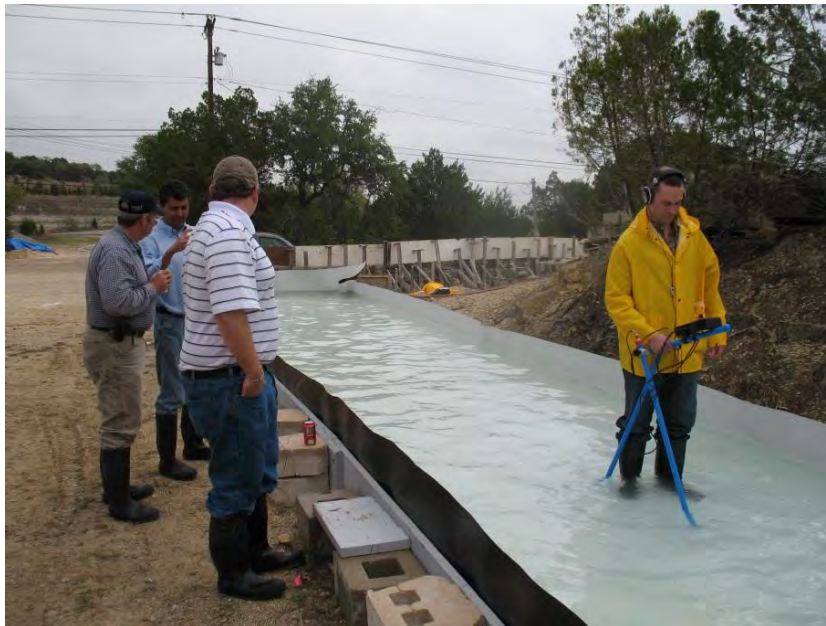
Figure 1. Water-covered liner test cell.
