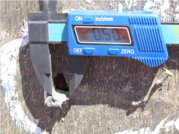
Figure 4. Leak #30 (Smaller leak signal.)
