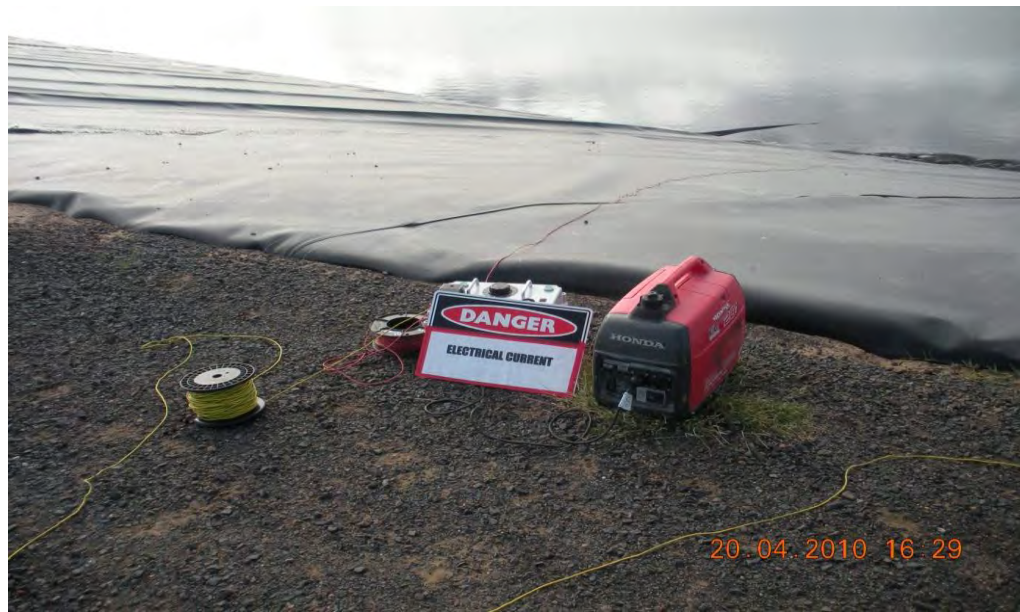
Fig 3. DC Generator and leads for applying electrical potential to the pond
