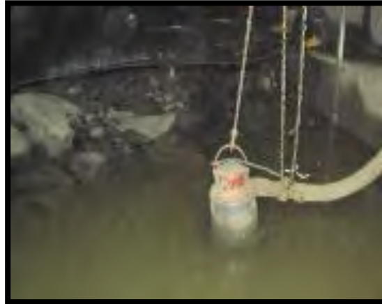
Picture 3: Sump pump
