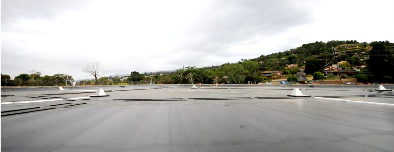
Figure 5: Cross view of completed floating cover showing tensioning of the cover and surface apparatus
