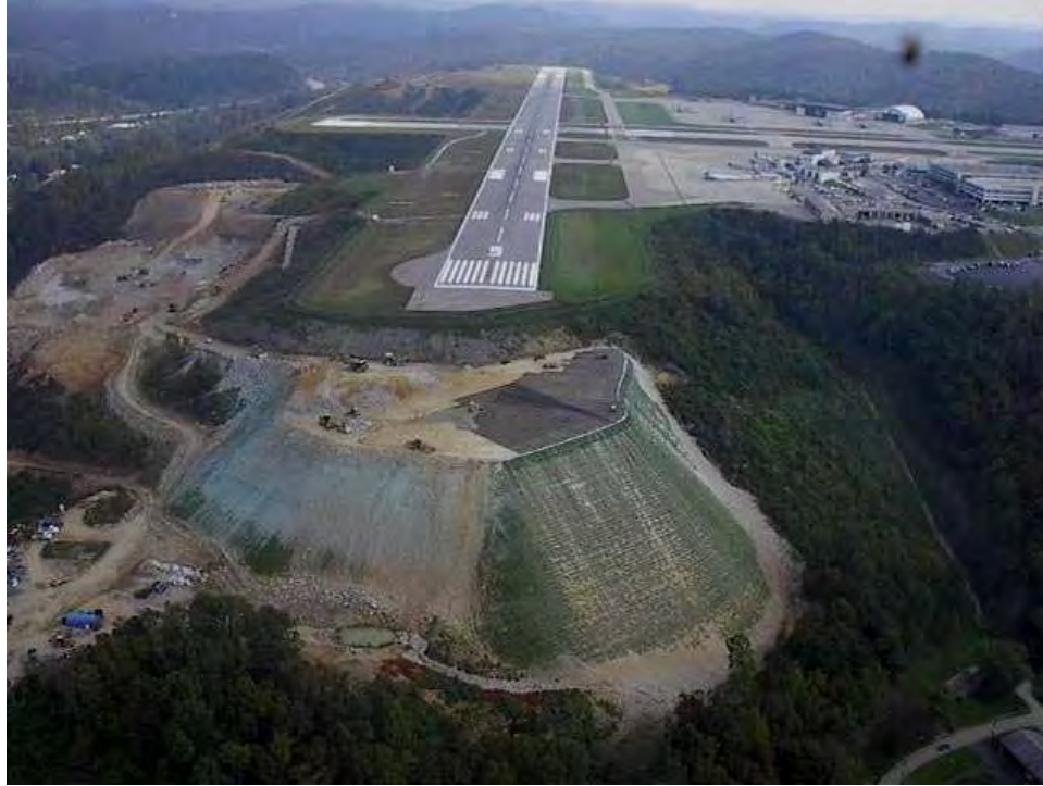
Figure 10. 242 ft (74 m) High 1H:1V Reinforced Soil Slope for Airport Runway Extension (Lostumbo, 2009)
