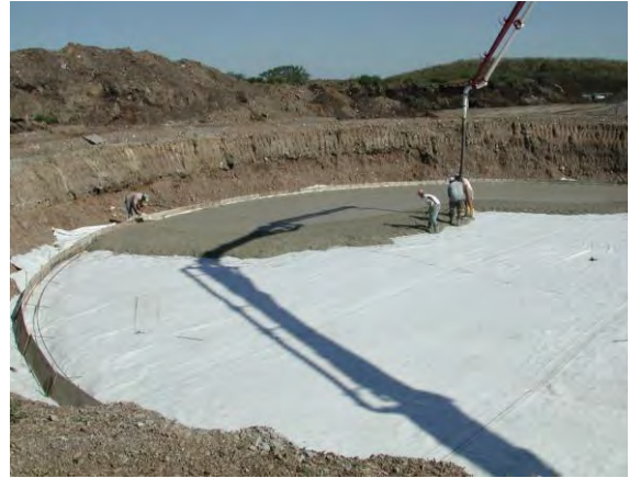
Figure 9. Concrete being poured over a GCL for a new concrete clarifier (Farming industry).
