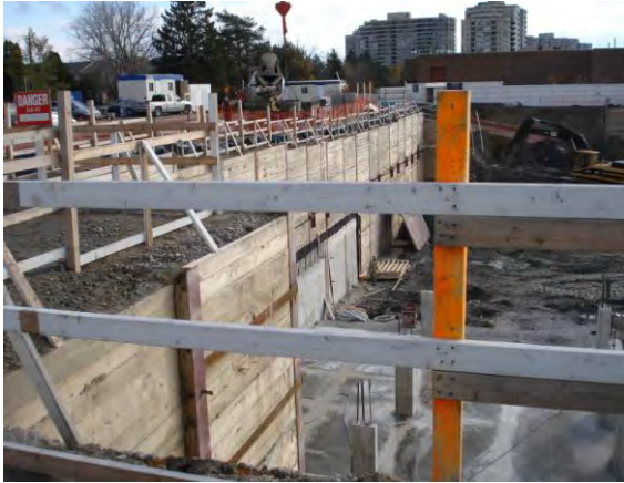
Figure 8. GCL used as a component in a waterproofing lining system for a new condominium building.
