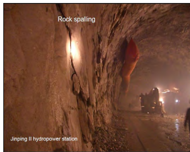
Figure 3: Higher vertical stress, UHE – Jinping II, Sichuan - China (Hudson, 2009).
