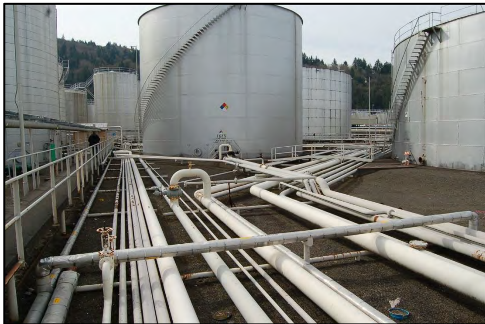
Figure 2: Pipes across Terminal
