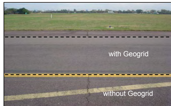
Figure 7. Joints of the concrete slabs reflect in the area where no reinforcement was used
