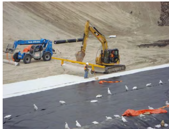
Figure 2. Landfill Base Liner (HDPE over GCL). GCL being used in a composite liner design used in lieu of a CCL component.
