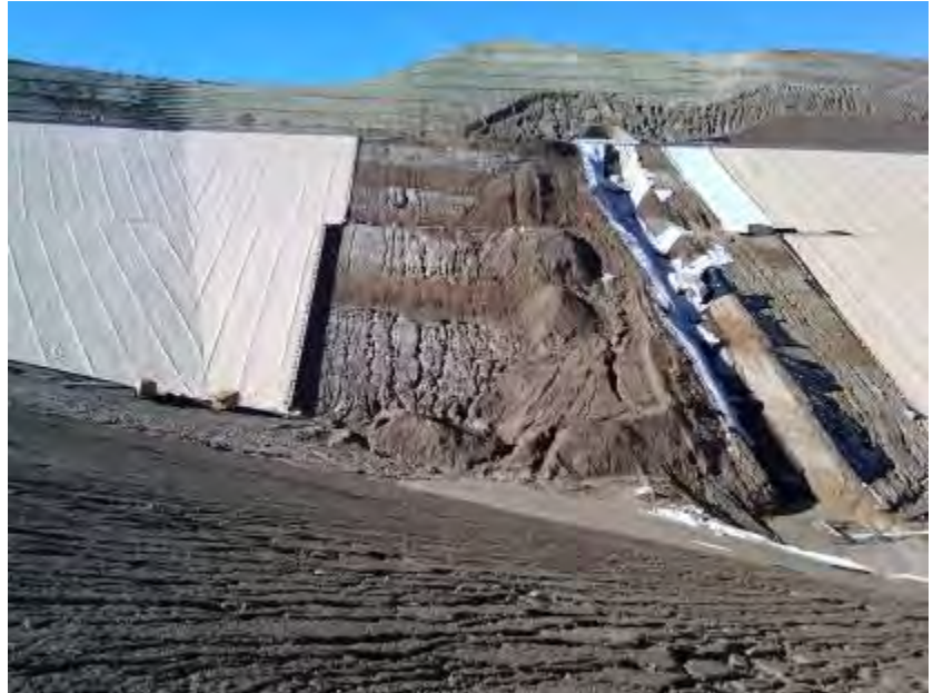
Figure 6: Subgrade damage after a significant rainfall event.
