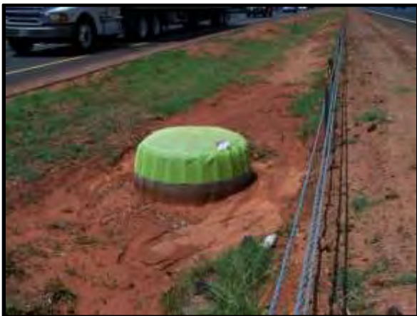
Figure 11 – SRD Protecting Inlet
