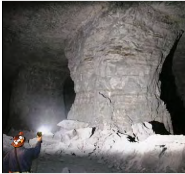
Figure 4: Partially benched pillar failing under elevated stress at the edge of bench mining (Esterhuizen, G.S. et al. 2011).
