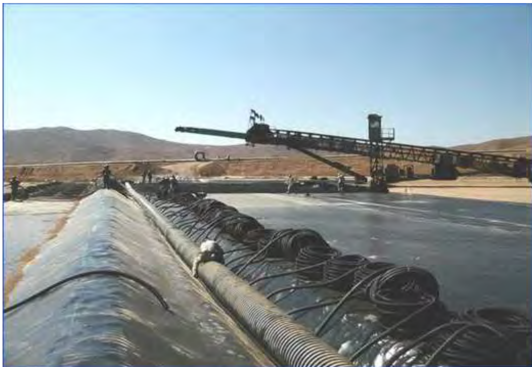
Figure 8. Solution collection system ready to be deployed in advance of ore stacking.
