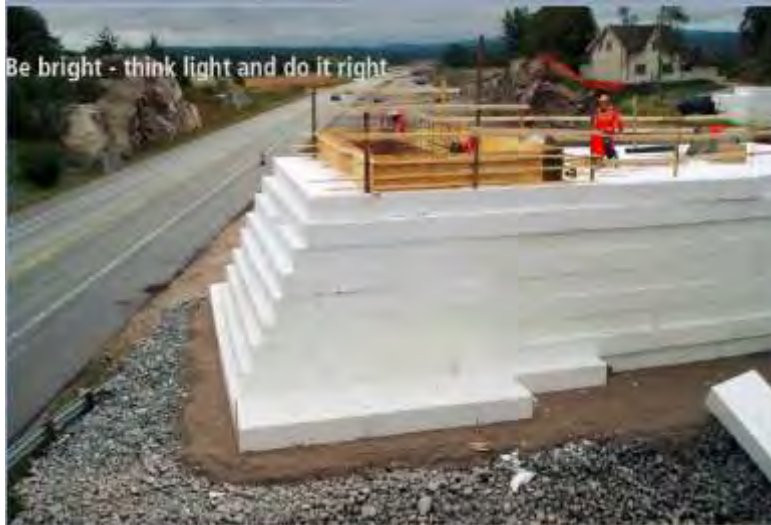
Figure 7a – Temporary bridge abutment over quick-clay (Courtesy of Norwegian Public Roads Administration).
