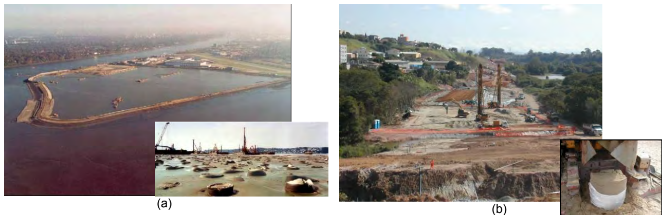
FIGURE 1 – (a) polder construction for EADS Industry enlargement in Germany (Source: Huesker); (b) first GEC Brazilian work – connection between SP-99 Rodovia dos Tamoios and BR-116 Rodovia Presidente Dutra. In details, installed columns.
