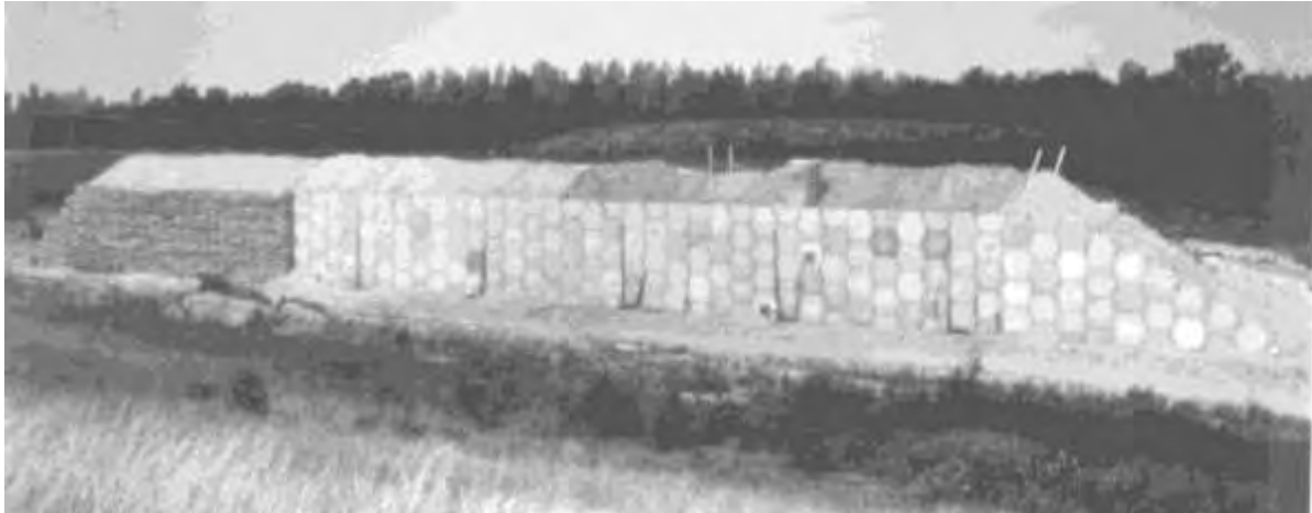
Figure 2. FHWA-Study, Instrumented walls constructed in Algonquin, Illinois by STS Consultants (from Christopher, 1993)
