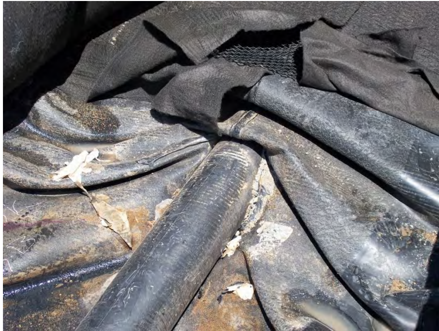
Figure 4. Containment system geomembrane and geomembrane apron around downgradient non-containment side of pipe boot upon discovery of ponded fluid.
