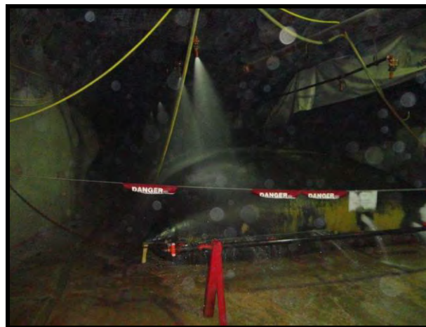
Picture 11: Sprinkler System
