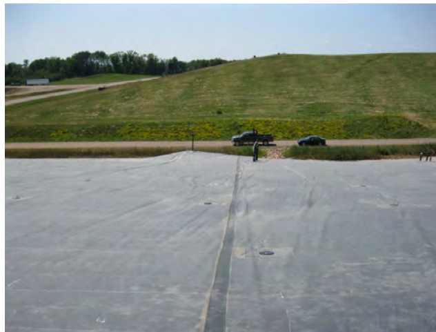
Figure 4. 45-mil EPDM exposed cover installed in northern Midwest, with Phase I completed in November 2011 and Phase II in June 2012.
