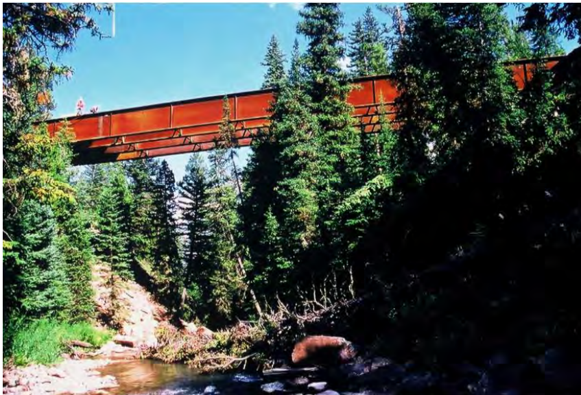
Figure 7. Big E-Z bridge. At 191 feet, the longest GRS-IBS structure in the world.
