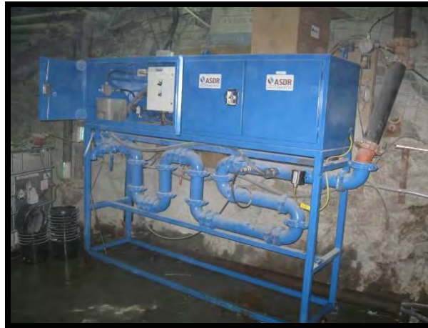
Picture 10 : Chemical dosing and mixing unit
