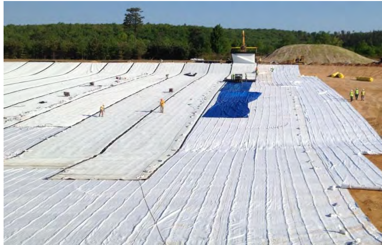
Figure 3. Photograph of the installation of an exposed, 1.5 mm (60 mil) HDPE liner underlain by a draitube geocomposite.
