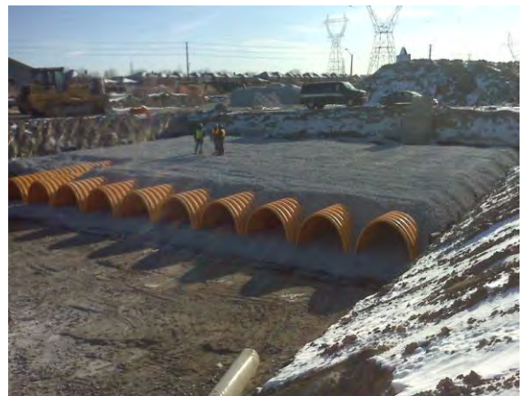
Figure 13. GCL being used instead of a PVC liner under Storm Chambers due to winter temperatures.
