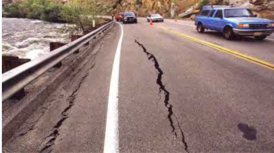
Figure 14. Major longitudinal cracking causing traffic diversion.
