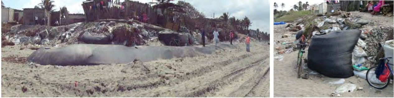
Figure 5. After 3 years Geotextile tubes installed in 2008 withstood the force of strong waves, by these Geotube® Technology were proposed as the best method to protect the coastal line.
