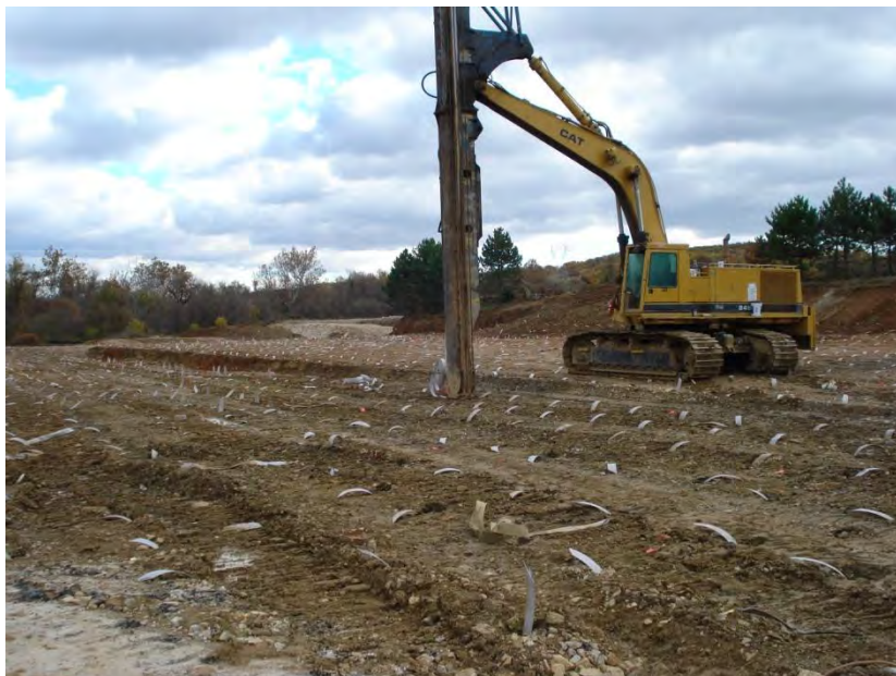
Figure 4- Installation of wick drains in the northern portion of the town center.
