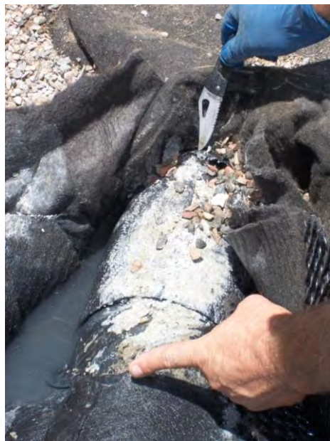
Figure 5. Observed displacement between original pipe boot weld location and final post-failure weld location (the knife and the finger are pointing to the two sides of the original weld).
