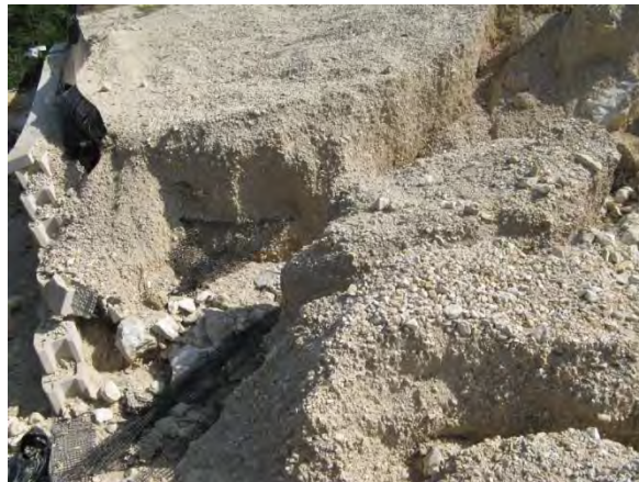
3.3(c) A Photo of the Wall Failure
