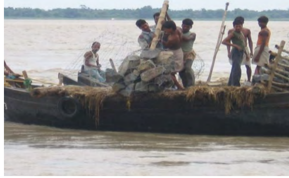
Laying of two layers of boulder filled wire crates on the Geotextile-Tarza mat composite
