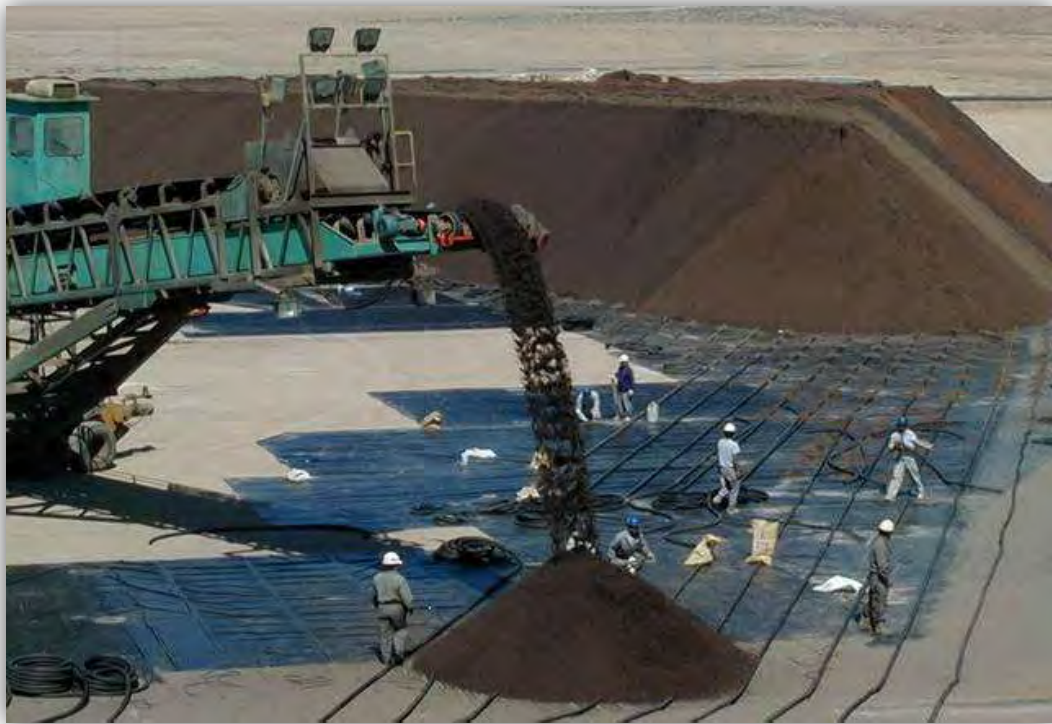
Figure 7. Mantoverde-style liner deployment showing ore being stacked soon after liner is placed.
