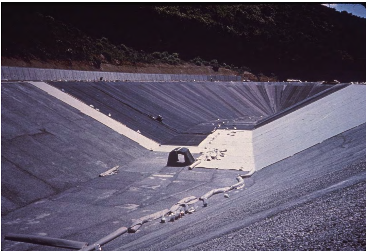
Figure 1. Butyl rubber geomembrane bituminous geomembrane double liner constructed in 1974. (Photo courtesy J.P. Giroud)
