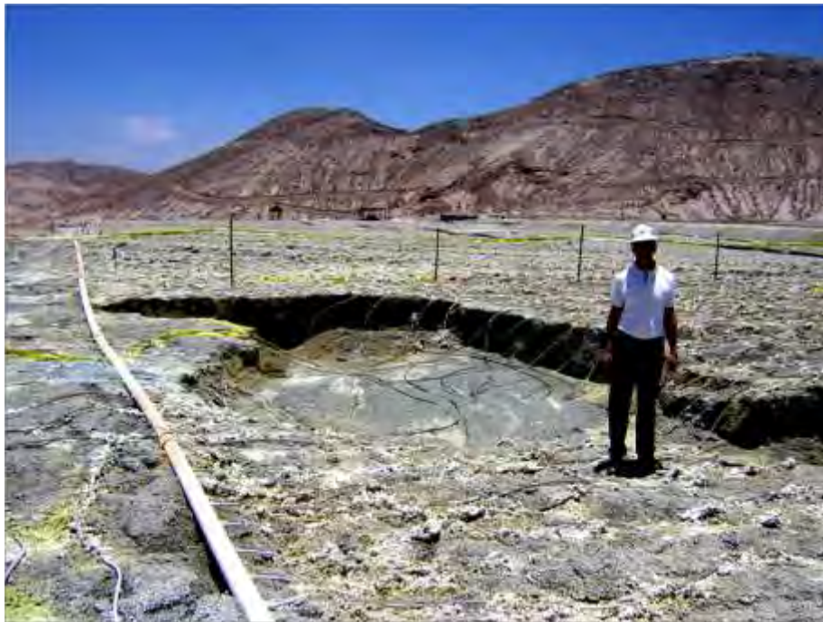
Figure 2. Sink hole on top of the heap at the Cerro Verde copper mine, Central Peru, which developed directly over a collapsed drainage pipe. In part because of failures like this, the Cerro Verde heap has experienced dramatic increases in the water level, to over 20 m above the liner, and some local liquefaction failures (see Figure 3).
