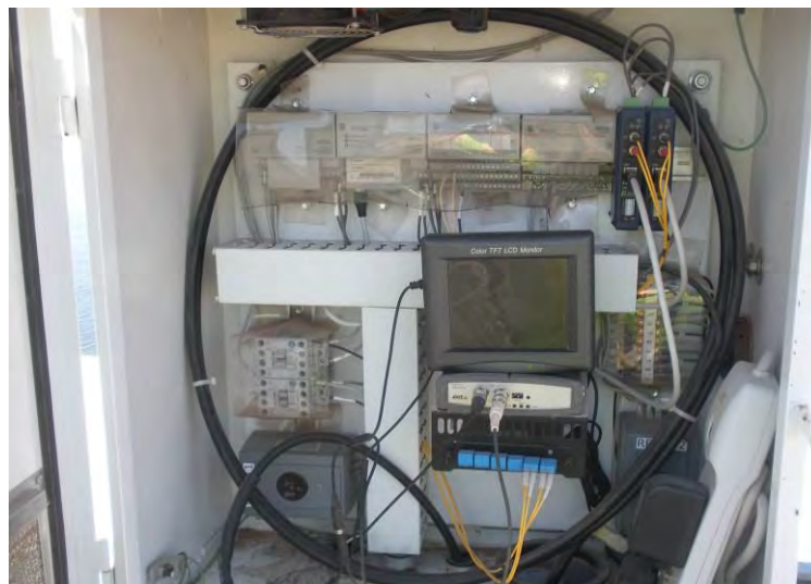
Figure 6. Leak detection monitoring equipment
