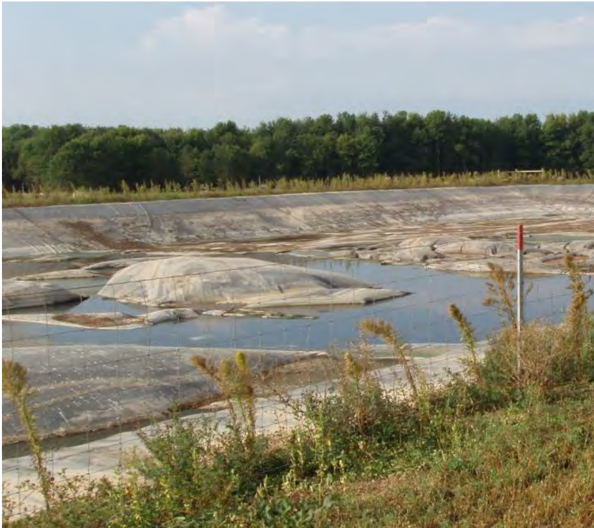
Figure 4. Large bubbles under liner visible after emptying (Case History No. 4).
