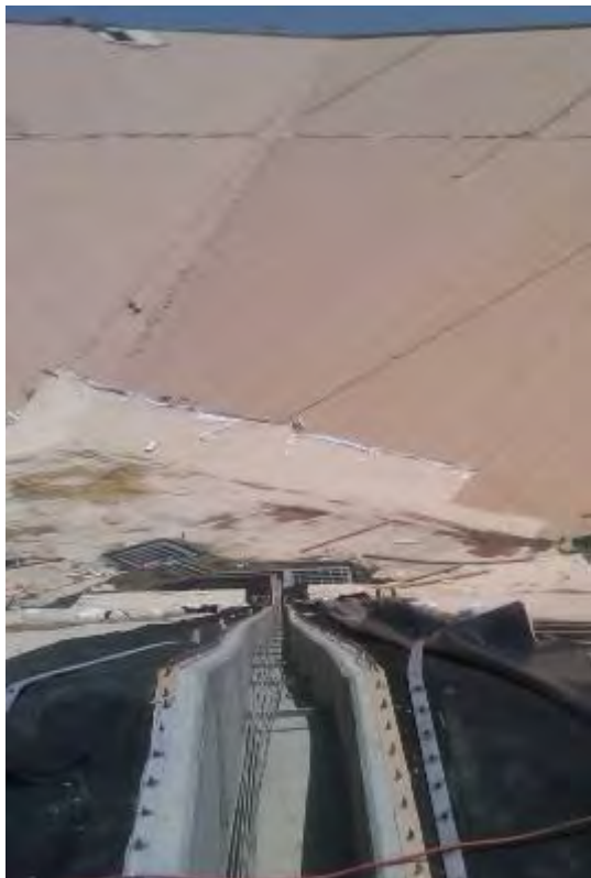
Figure 7: Pneumatic tubing in concrete trough
