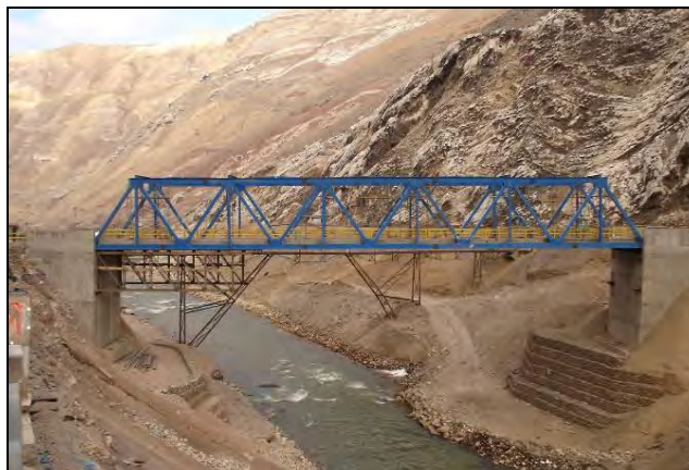
Figure 10. DTSW mesh/ Geosynthetic reinforcement System platform bridge abutment Doe Run mine (Peru)
