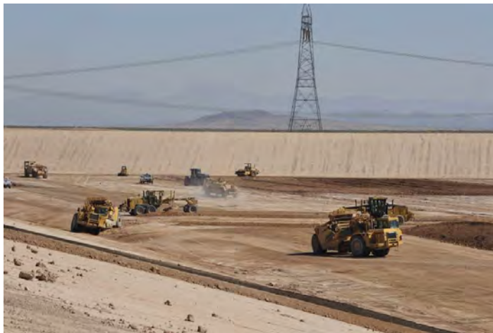
Figure 8. Regrading of pond floor subgrade in Pond 2. The subgrade elevations isolate identifiable areas and sumps.
