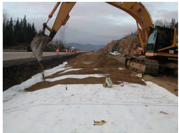
Figure 11. GCL being used to line underneath a highway – groundwater protection against road salt – GCL containing a polymer.
