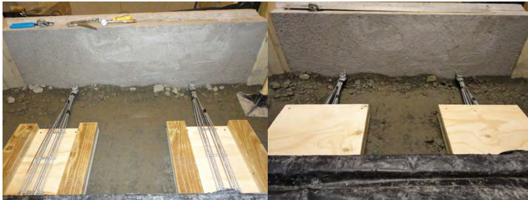
Figure 5. Photos of DPS-TAB connections and discrete-strip with sleeve enclosure.
