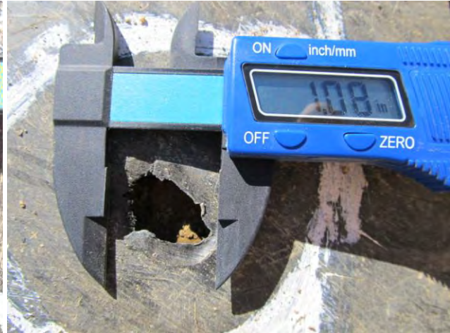
Figure 5. Leak #31 (Larger leak signal.)
