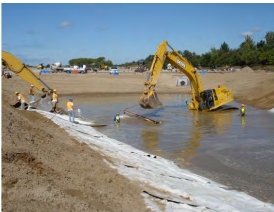
Figure 12. Can you use a GCL in this application? Every project engineer has his/her needs. GCL being deployed in a SWM Pond containing a high water level. Bizarre situation but required by project engineer who had wanted a liner without dewatering the site.
