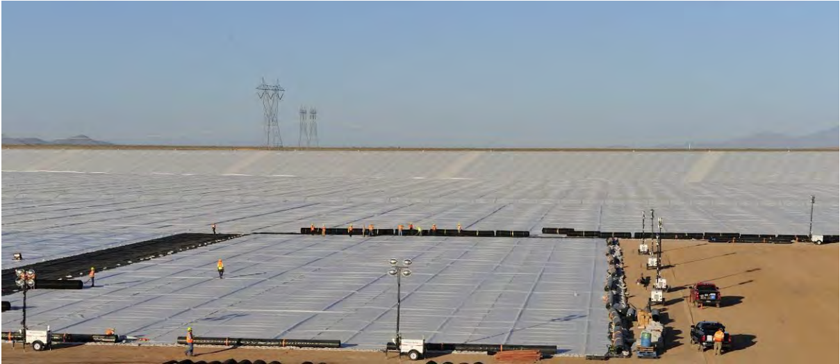
Figure 9. Photo of installed primary geomembrane layer and deployment of geonet drainage layer over installed secondary geomembrane.
