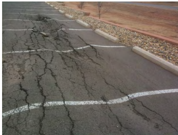
2.2(c) – A Photo of Pavement Failure
