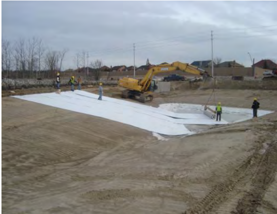
Figure 4. GCL being deployed for a SWM Pond in winter conditions. Note the ice (30cm thickness), ie. stubborn water (water table). Overlap increased from 30cm to 90cm over the ice.
