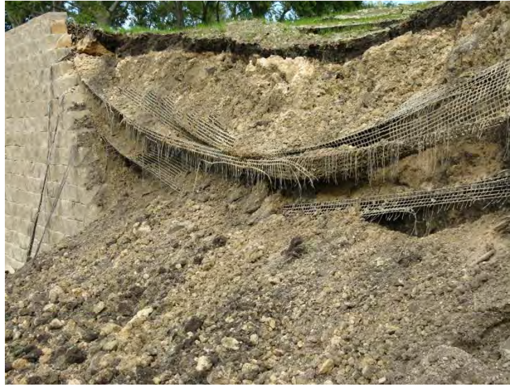
(c) A Photo of the Failure
