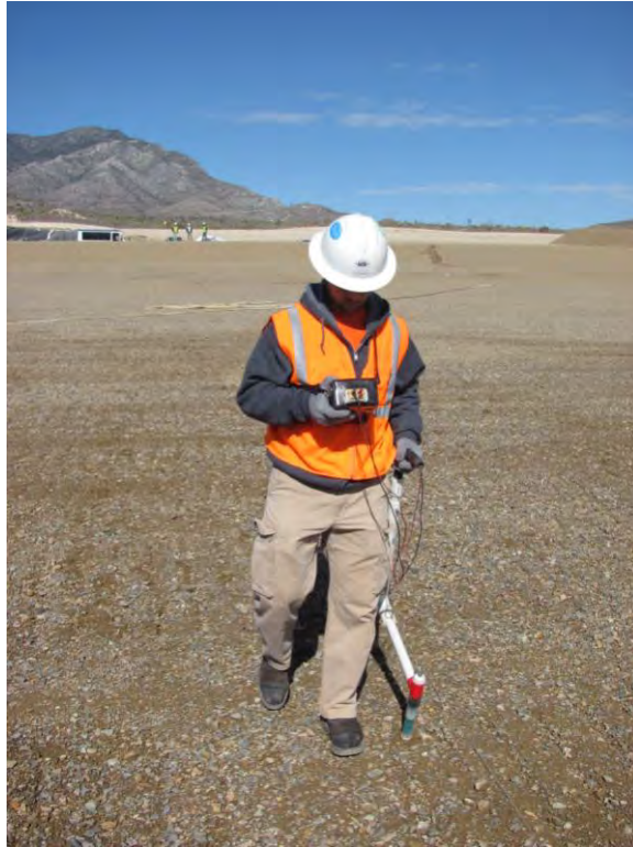
Figure 1. Leak location survey being performed on soil-covered geomembrane using a digital data acquisition system.
