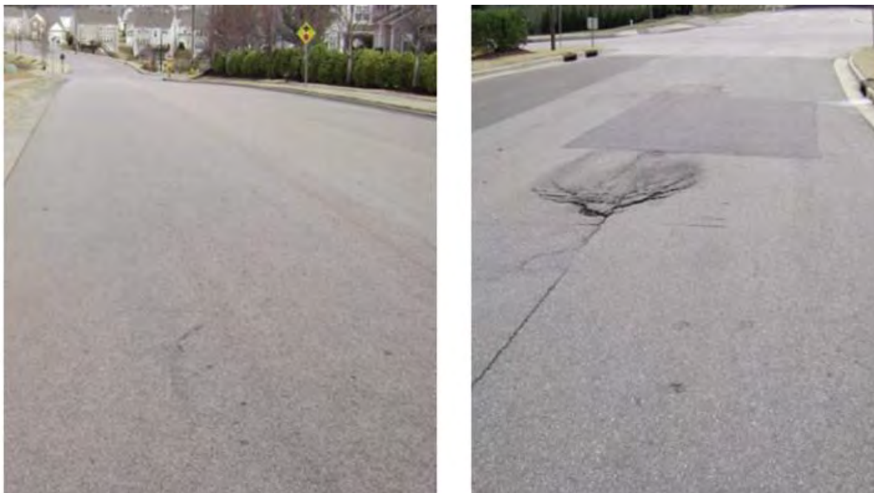
Figure 3. Conditions in 2011 on Country Trail with reinforcement geotextile and Parkstone Drive without geosynthetics.
