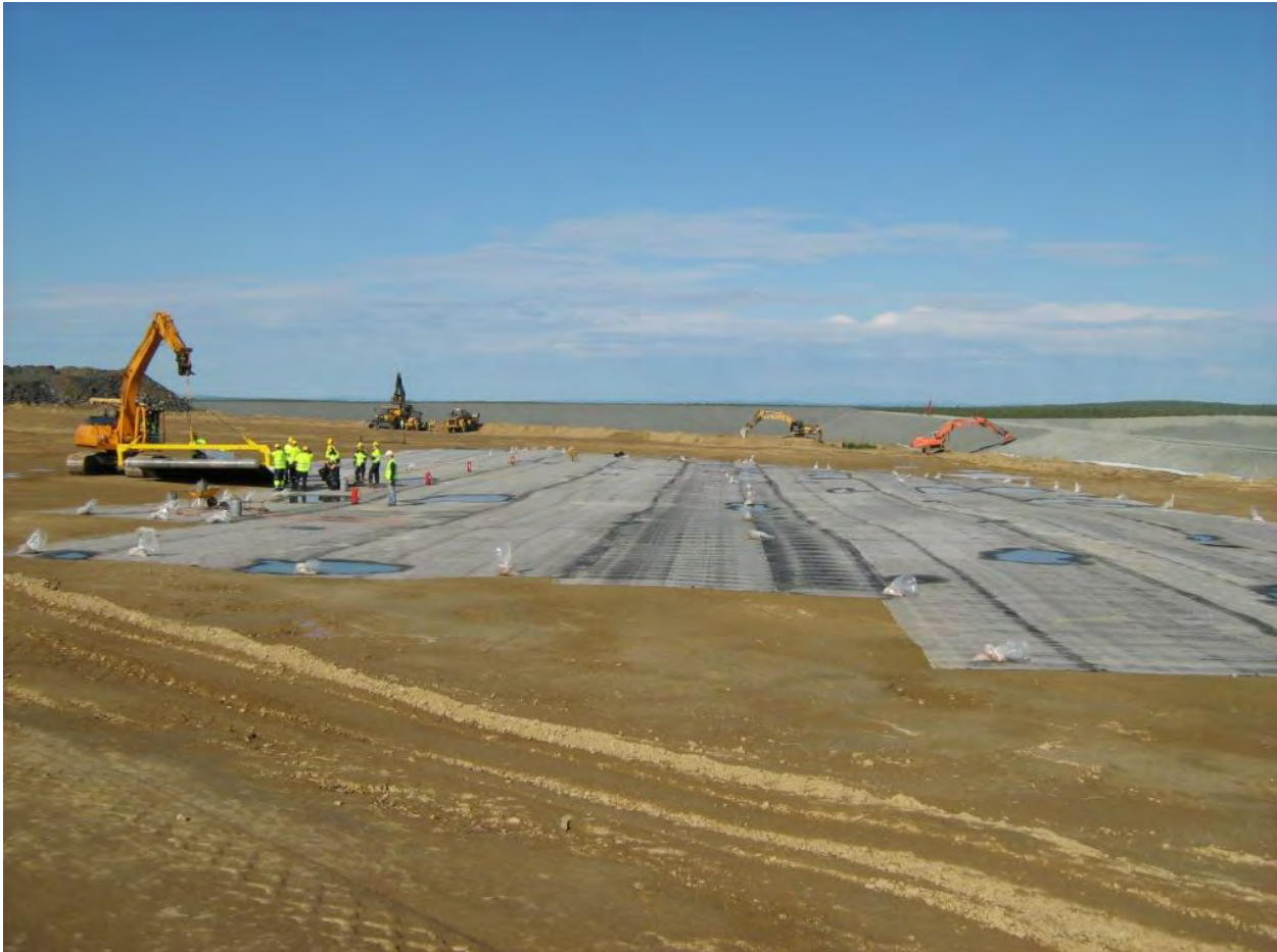
Figure 6: Liner on bottom of pond – note absence of wrinkles
