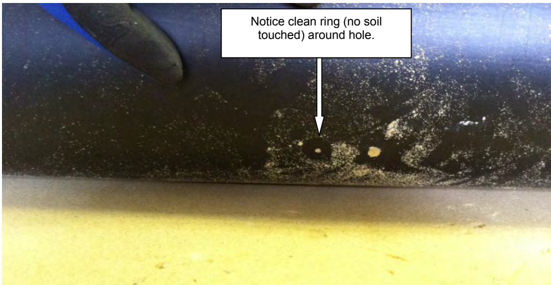
Figure 3. Hole Over Depression in Subgrade.
