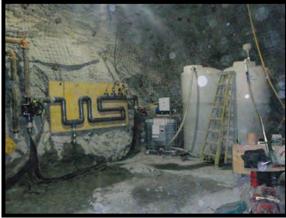
Picture 6: Chemical conditioning unit
