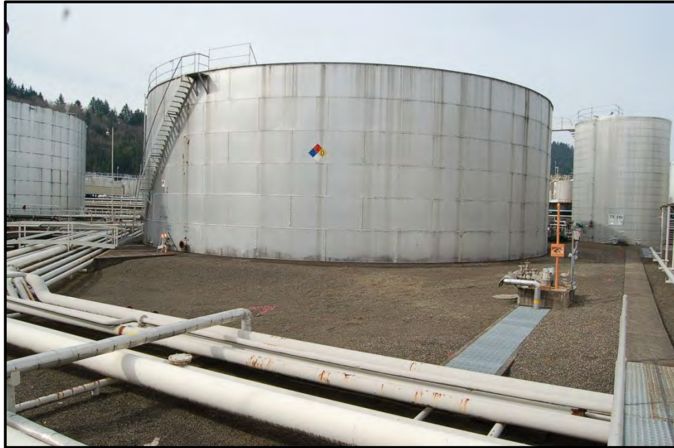
Figure 1: Tank 2 in foreground and Tank 141 in background prior to demolition – note Tank 2 is a riveted tank
