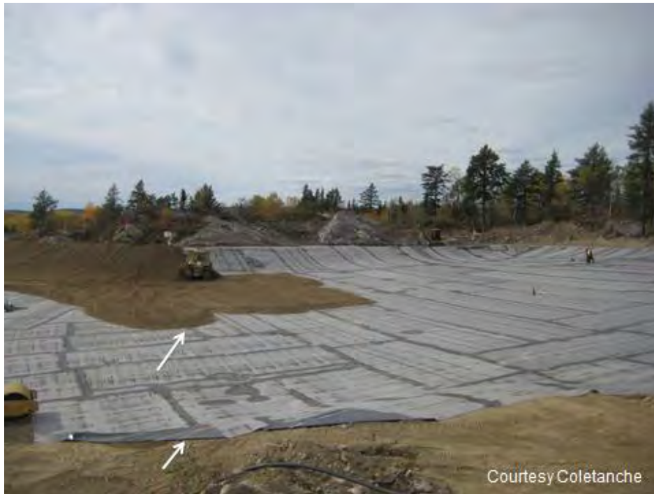
Figure 2. Bituminous geomembrane. No wrinkles (top arrow). No creasing at fold (bottom arrow).
