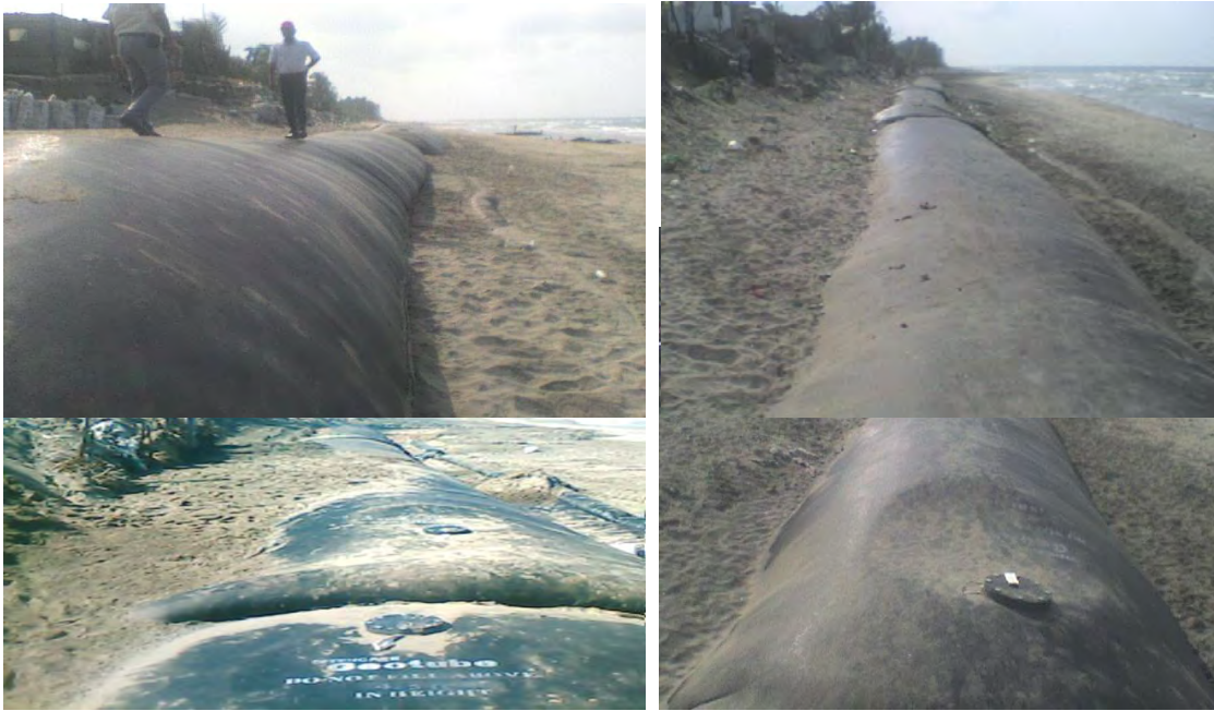
Figure 3. The units were covered with sand (from a nearby mine) to protect them against the traffic of villagers and visitors over them and vandalism.
