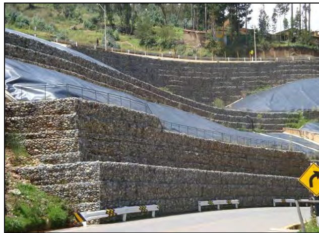
Figure 9. DTSW mesh/ Geosynthetic reinforcement System for access road to the "Antamina" mine (Peru)
