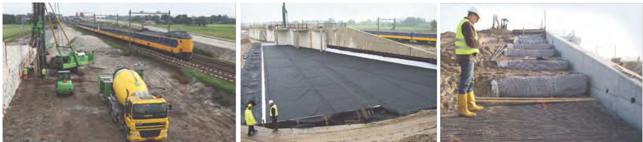
Figure 9: Hanzelijn pile installation (left), bottom grid (middle) and layered soil reinforcement (right)
