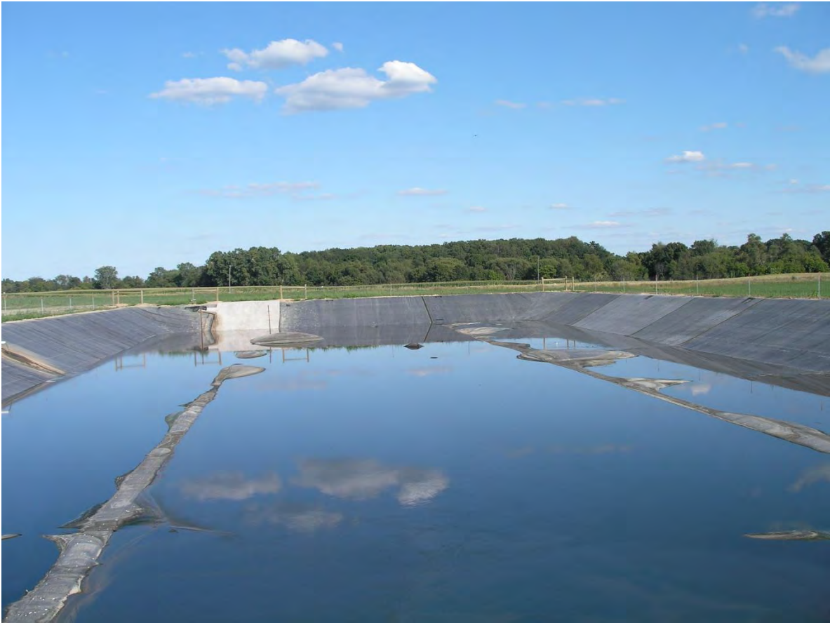
Figure 3. Gas accumulation in venting system (Case History No. 4).
