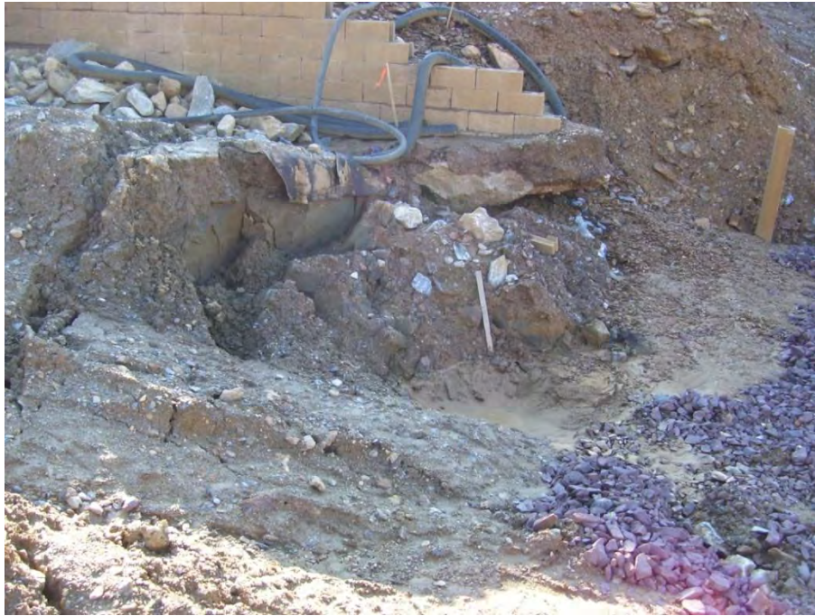
Figure 6- Loss of foundation due to mini-pile installation.
