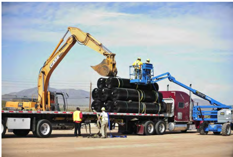
Figure 11 – Unloading of geonet drainage material using man-lift for attachment of roll straps to excavator.
