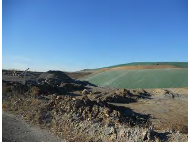
Figure 1. The 40-mil textured high-density polyethylene (HDPE) exposed cap on the first use of the trenchless ballast approach in the United States used a green-tinted membrane to help the cap blend into the surrounding environment.
