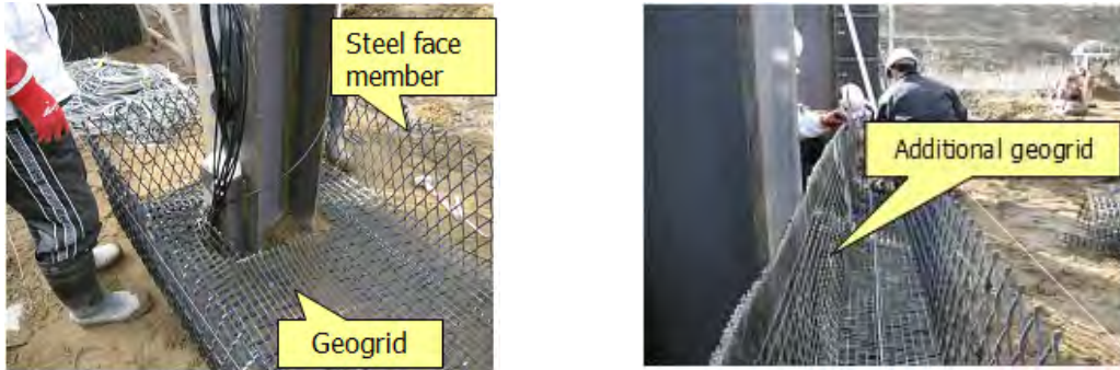
a) Installing of steel face member and geogrid b) Installing of longitudinal additional geogrid
