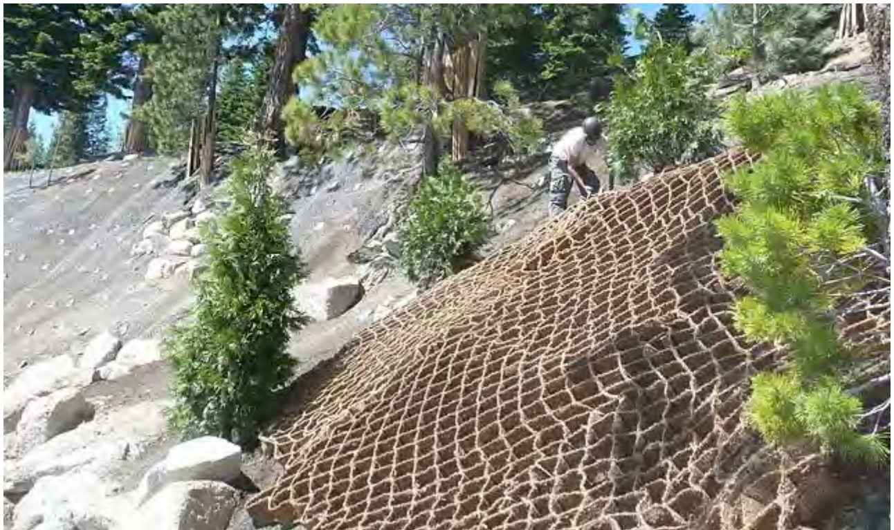
Figure 4 - Cedars and pines planted through keyholes in cellular confinement and steel mesh.
