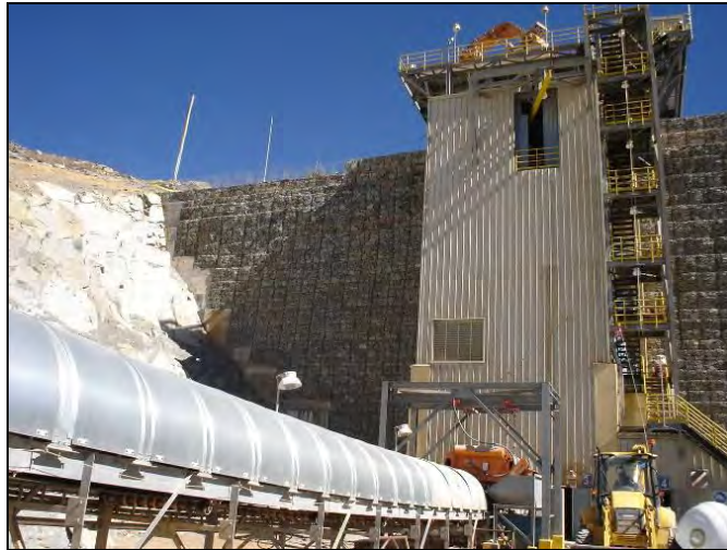
Figure 12. DTSW mesh/ Geosynthetic reinforcement System for walls for access to the primary crusher Alto Chicama ( h_{\max} = 23.50\text{m} - Peru).
