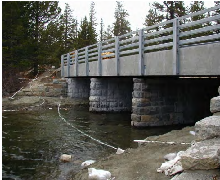
Figure 6. Mammoth Lakes bridge. Note that the deck clears the historic piers by approximately 4 inches.
