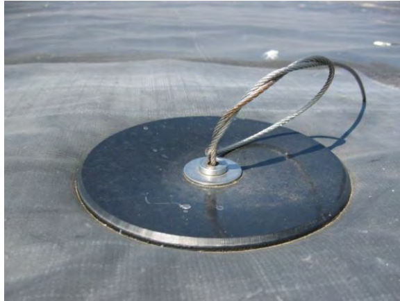
Figure 5. Percussion anchor installed on 45-mil EPDM exposed cap. An additional reinforced scrim patch is installed over the non-reinforced geomembrane to provide a significantly stronger attachment and pull-through resistance of the anchor to the geomembrane.
