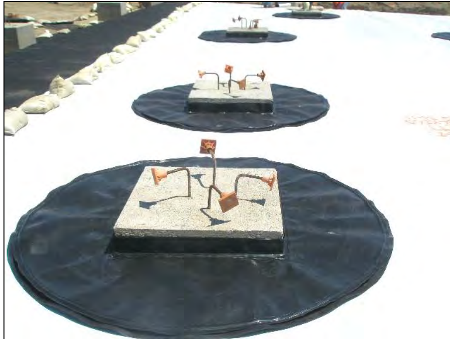
Figure 10: Boot-Ring system at first building on the site (boot welded to white geomembrane below)
