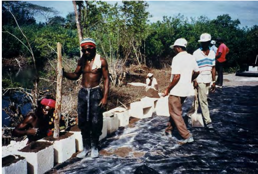
Figure 4. Green Island bridge under construction. The construction was nearly all completed using local unskilled labor and hand tools.
