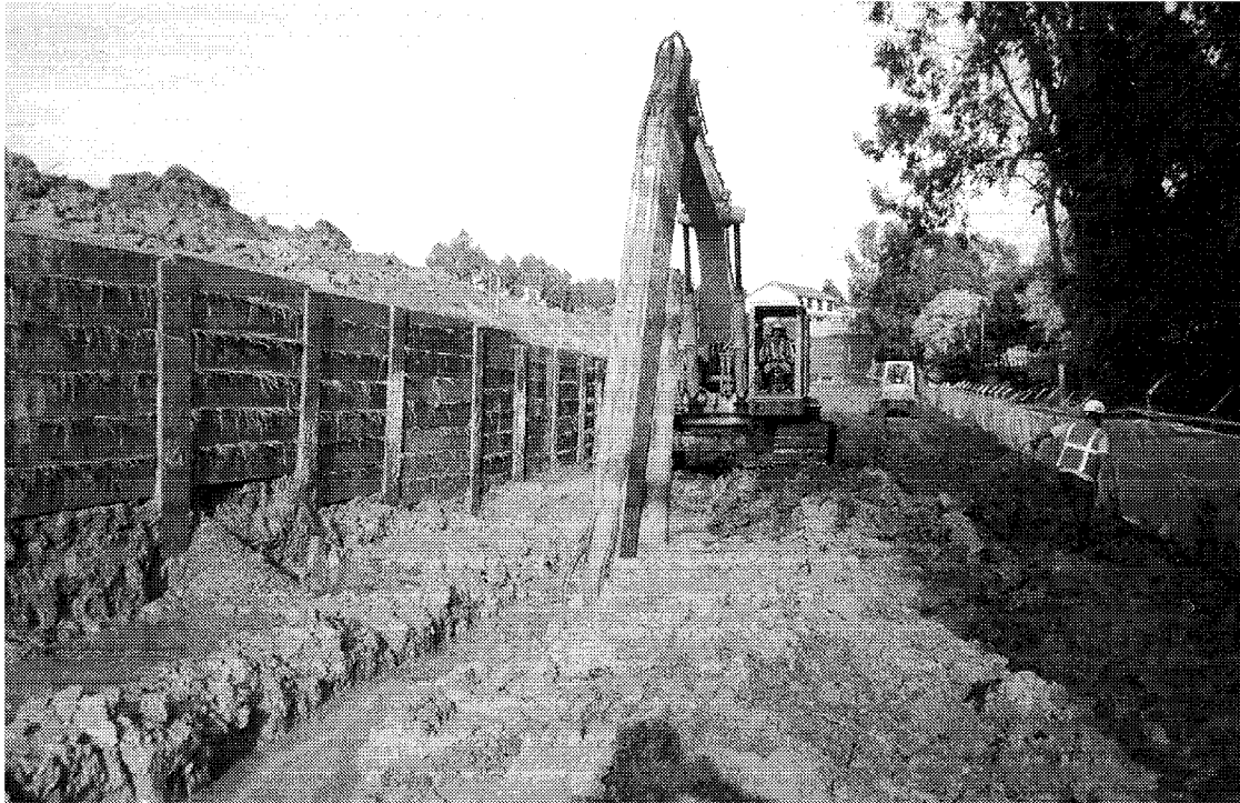
Figure 4. Soldier Pile Wall and Working Pad for Excavation of the Low Permeability Soil Cut-Off Wall
