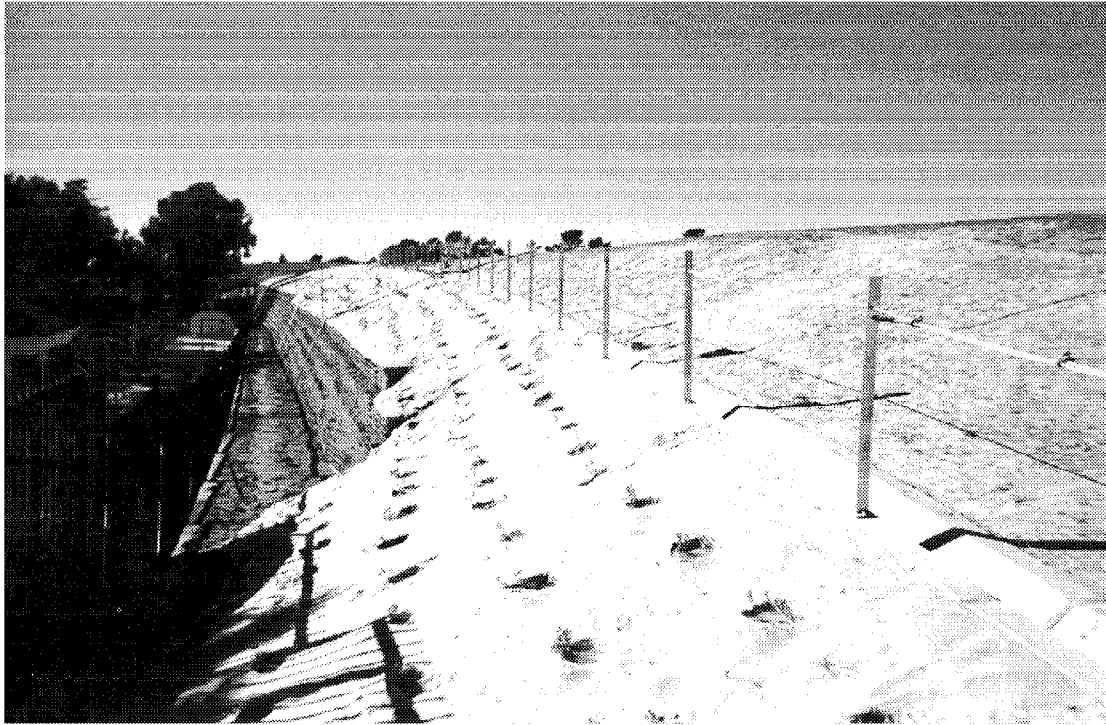
Figure 6. Completed Reinforced Earth Structure over the Liner System, Cut-Off Wall, and Soldier Pile Wall
