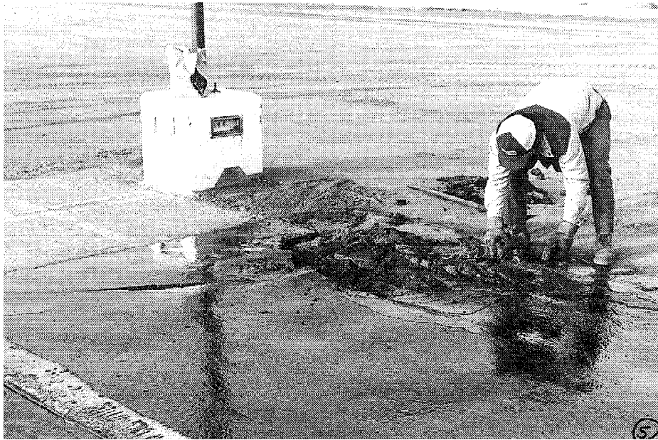
Figure 8 - This broken pavement was left in place under the paving fabric.
