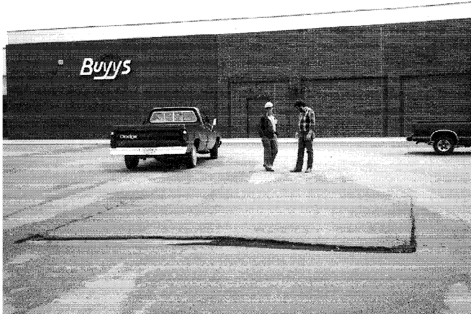
Figure 4 - Delamination of overlay in a parking lot in Indiana
