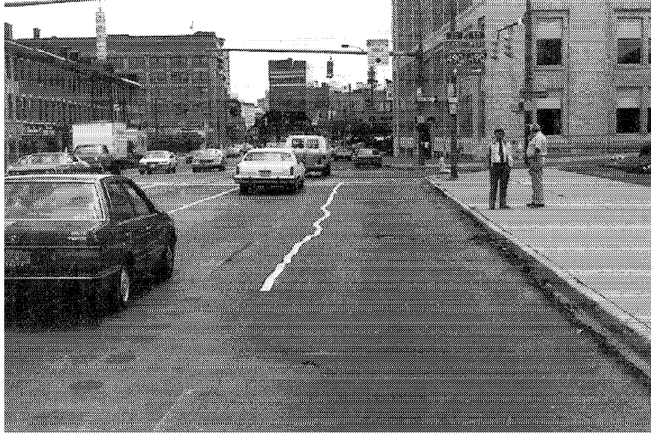
Figure 3 - Shoving of overlay on a city street in New York.
