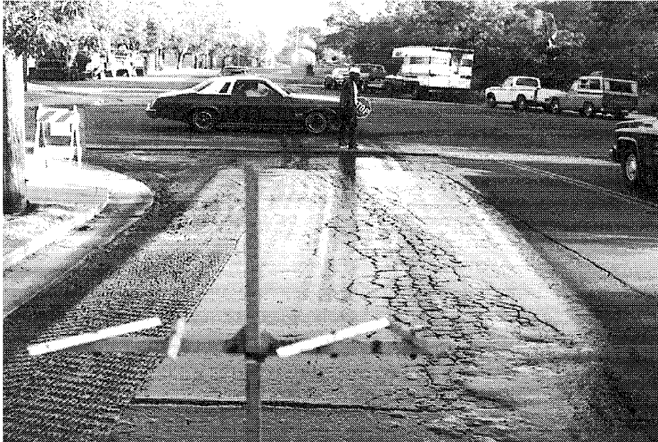
Figure 9 - Area of unstable base material left under the paving fabric
