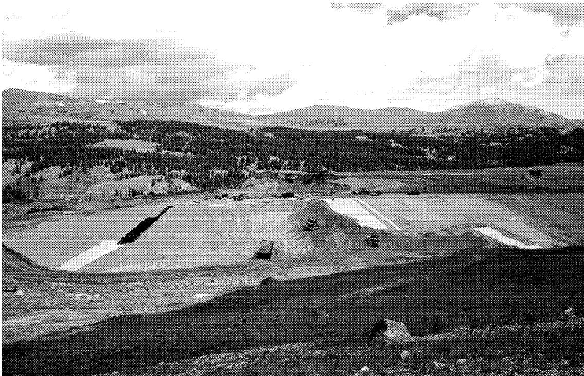
Photograph 1. The Summitville Mine Superfund Site heap leach pad capping system under construction.
