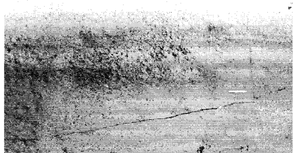
Figure 23- Contraction cracks in side walls
