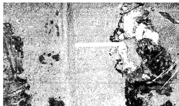
Figure 27- Blisters formed on old tar
