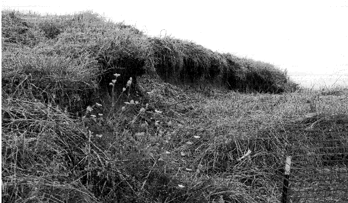
Figure 5. Serious Surface Cracking Prior to Repairs
