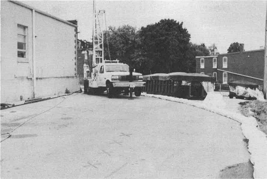
Figure 5. Truck mounted drill rig with mast extended. Barrier wall alignment in foreground.
