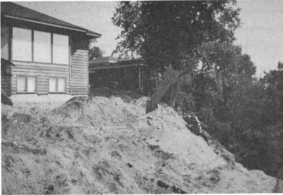
Figure 7. View of the collapsed wall; the sand pail (see arrow) is where the owner's 4-year old daughter was playing when the wall collapsed.
