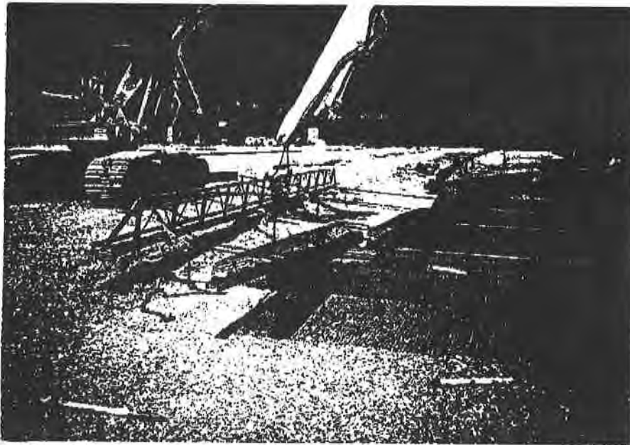
Figure (2): Unit with arrangement for prestressing of the reinforcement and subsequently covering with gravel
