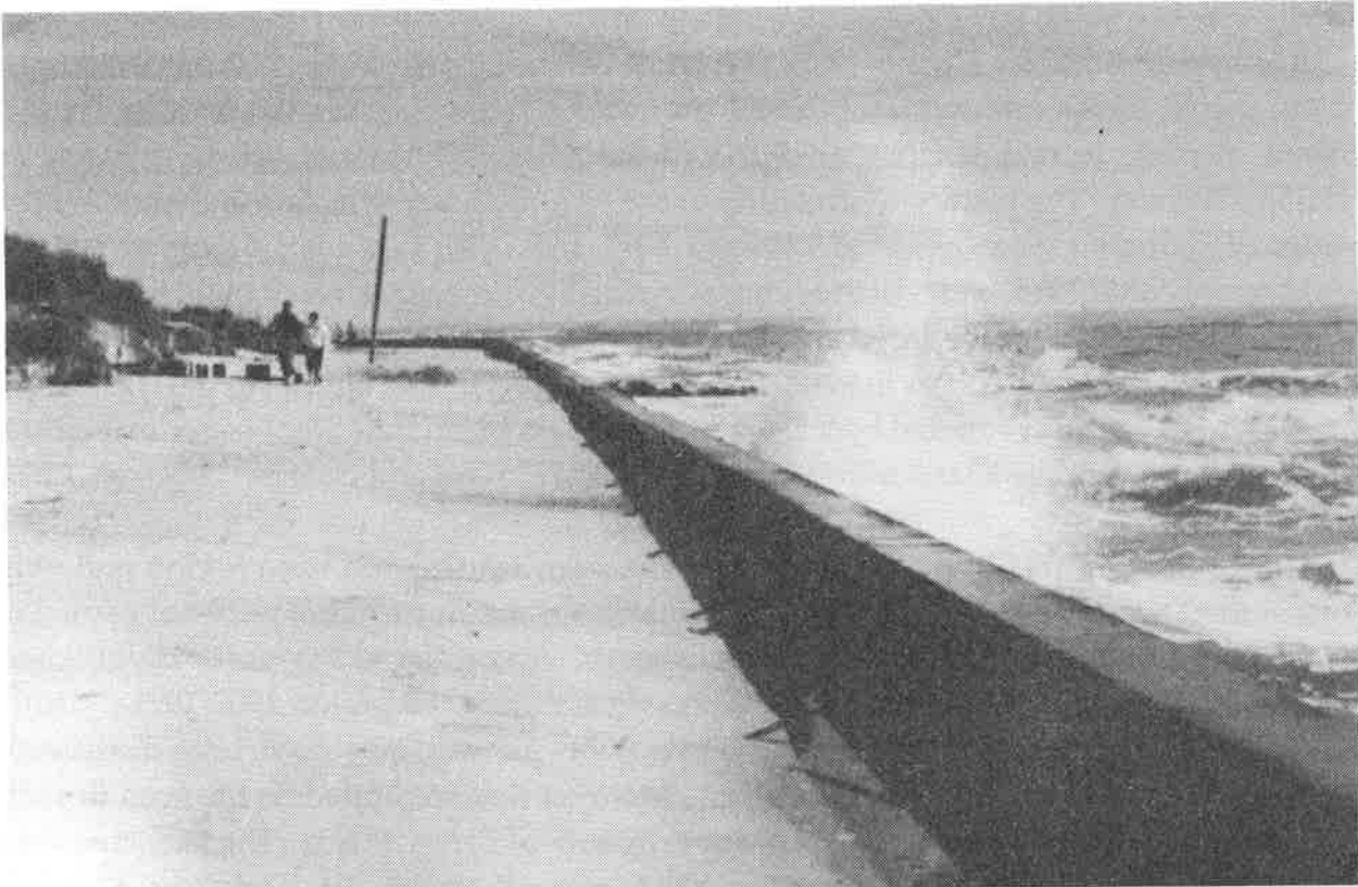
Figure 3 Pre-Project Seawall Conditions (Looking East)
