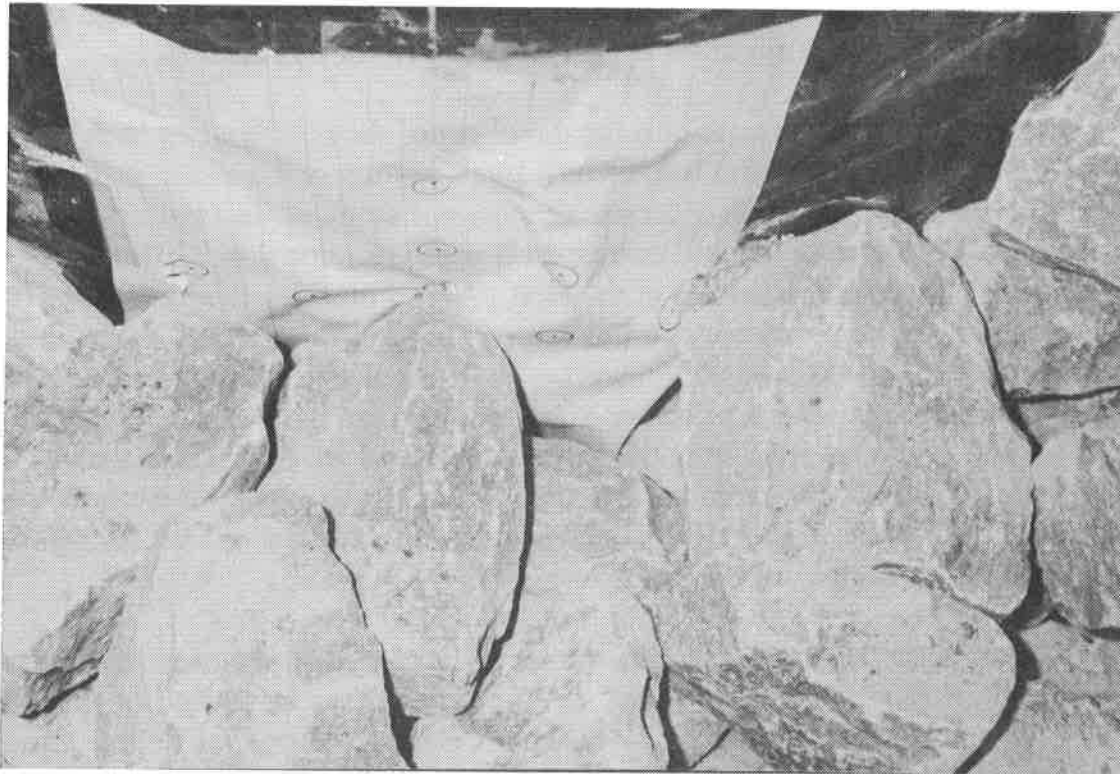
Figure 5. Discontinuous support provided to pipe by 50 mm stone
