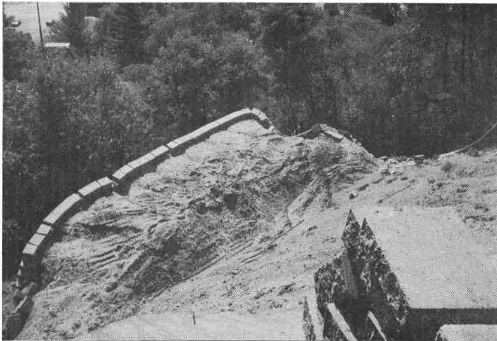
Figure 9. View of the collapsed wall, looking downslope.
