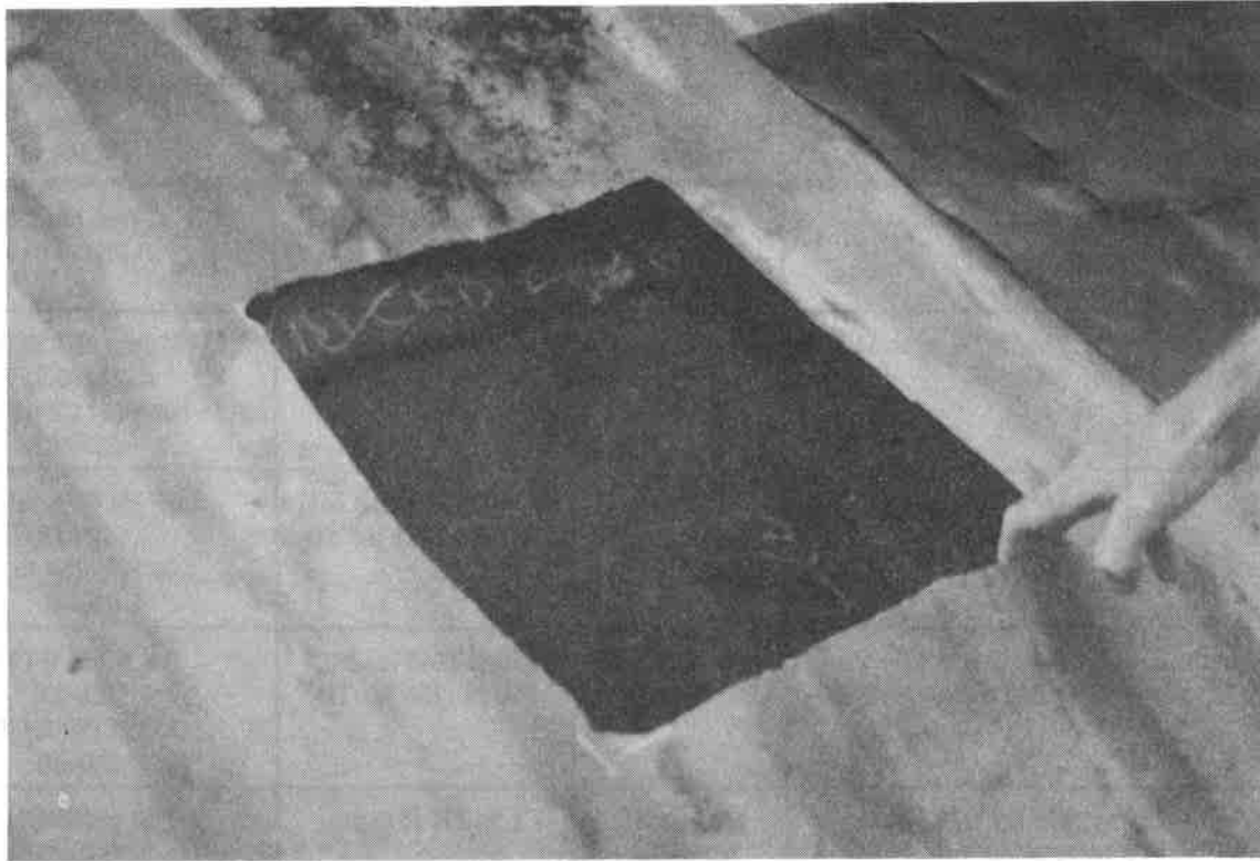
Figure 4. Author's initials from the 1977 installation, visible on the bottom lining.
