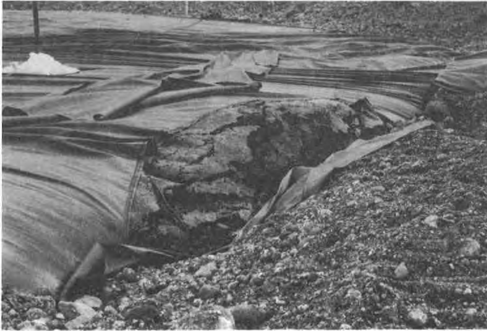
Figure 8. Failure of Type 1 seam during test section.
