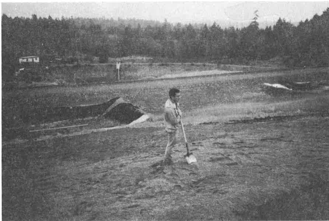
Figure 3. Three Stage Geotextile Lined Infiltration Pond
