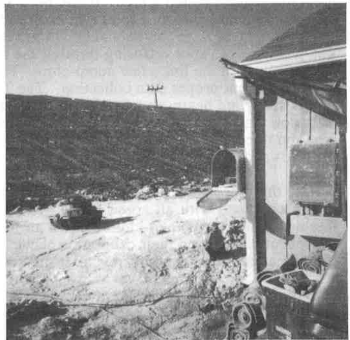
(d) The Control Panel and Data Acquisition Station
