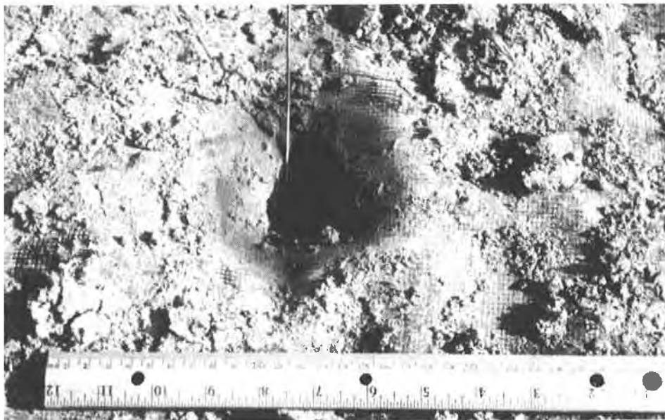
FIGURE 7. FIVE CENTIMETER HOLE IN LINER DETECTED UNDER SOIL COVER
