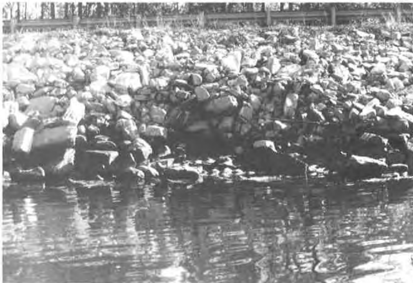
Photo 1: Example of Erosion Control Structural Problem Caused by Failure of Geotextile Underlying Rip Rap
