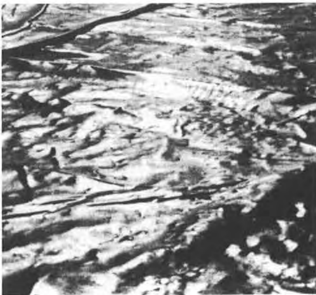
Figure 12. Stones protruding against underside of secondary liner.
