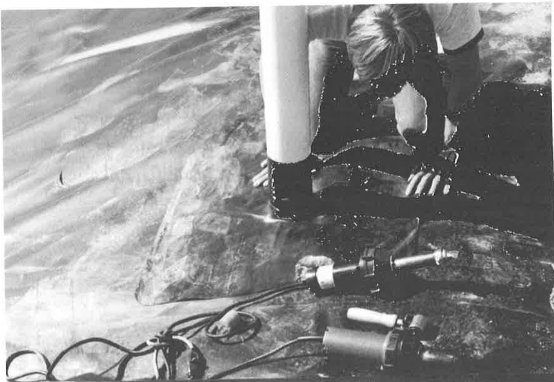
Figure 8. Field fabrication of boots and thermal seaming around penetration by hot air methods.
