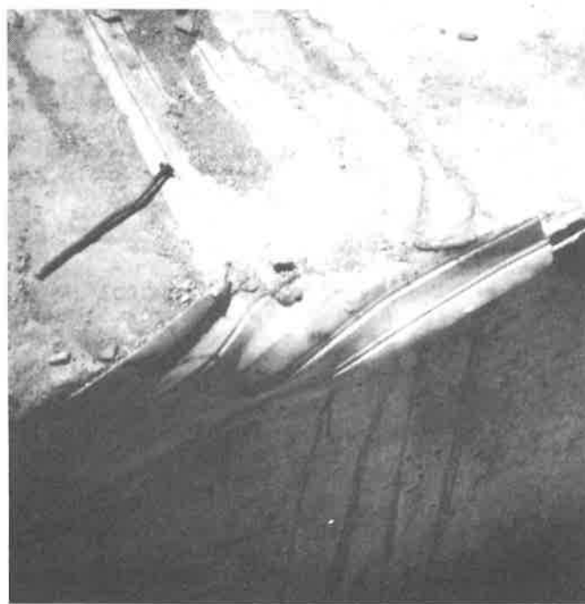
Figure 5: A geosynthetic anchor strip, compound bend at right side of inlet structure.
