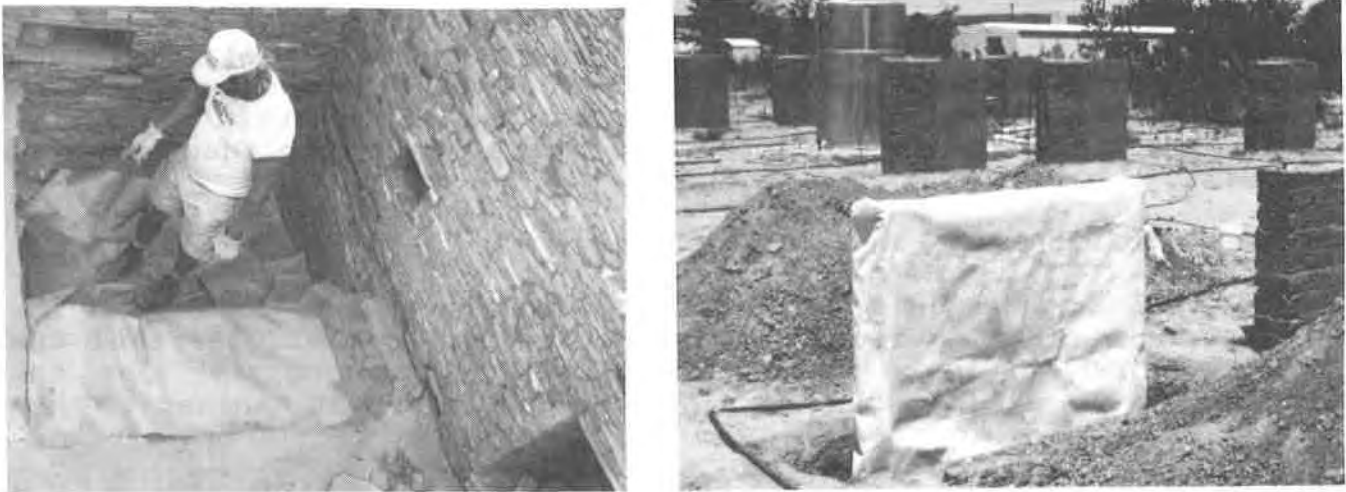
Fig. 11. The use of geotextiles in a reburial operation (left) and to protect adobe test walls at Fort Selden (right).
