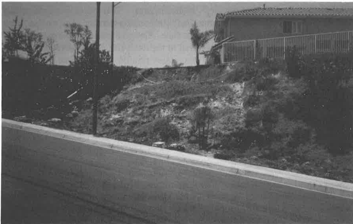
Figure 2. SURFICIAL SLOPE FAILURE
