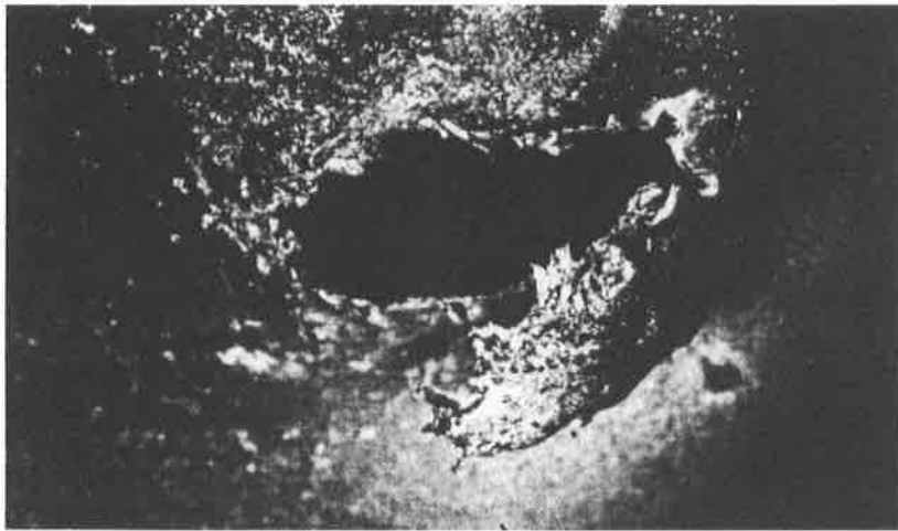
Figure 16. Stone puncture hole in secondary liner.
