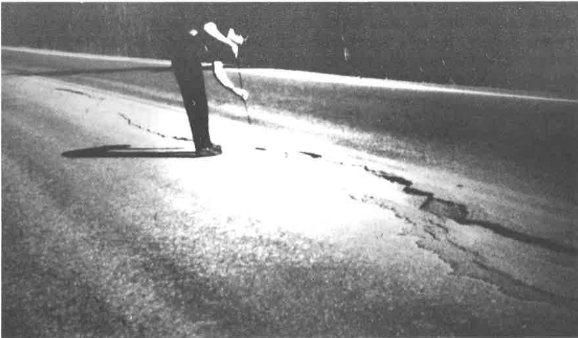
Photograph 1 - Longitudinal Cracking on Farmers Loop Road
