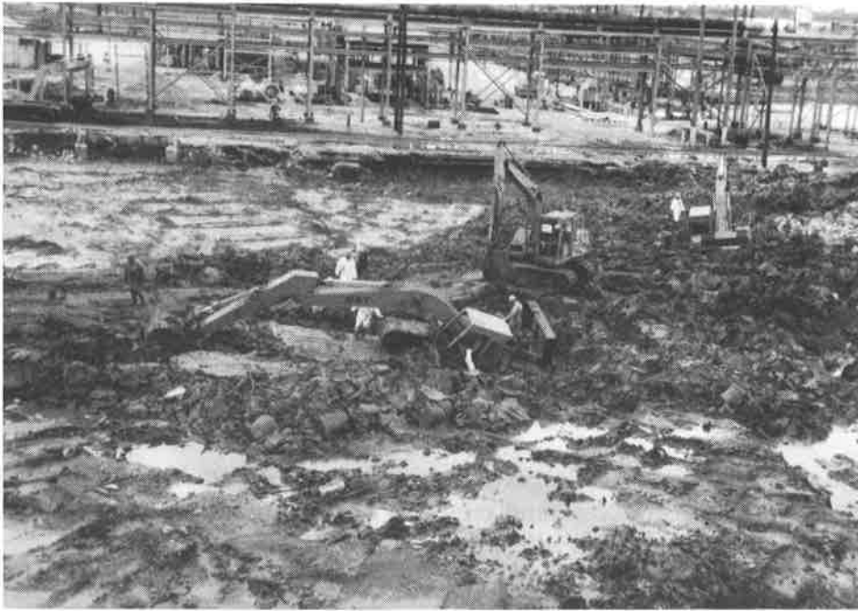
PHOTO 1: Hydrotreater Unit site during initial excavation. Photo shows excavation equipment that had sunk into the soft soils and was being extracted by a third piece of equipment.
