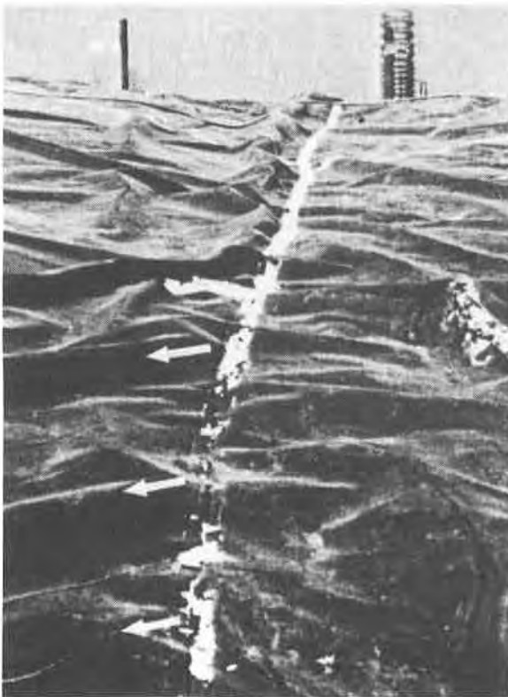
Figure 3. Epoxy paint peeling off a seam. Note flow marks (arrowed) on left panel; smooth surface on right panel.
