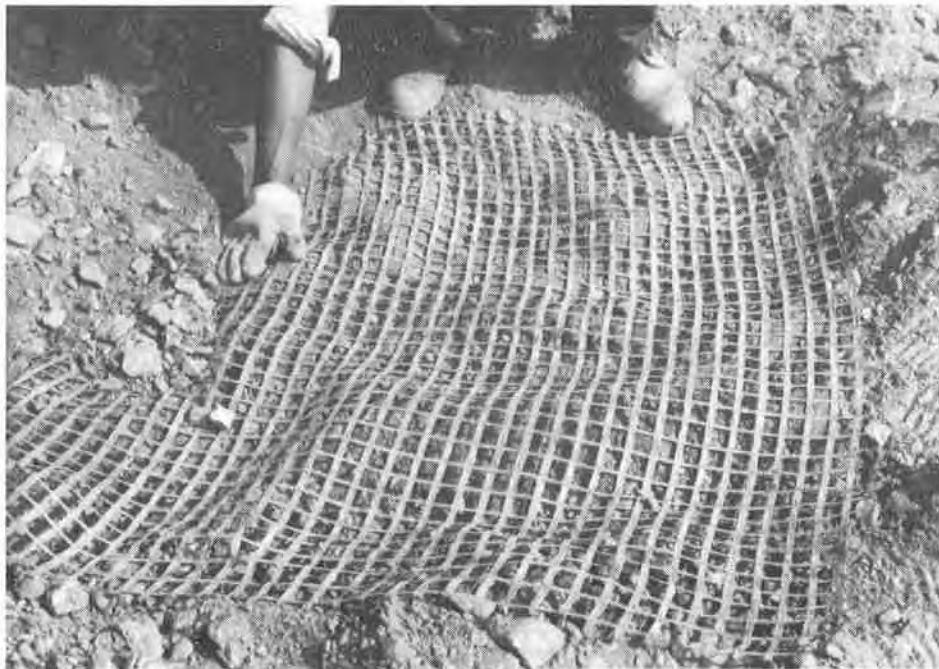
Figure 8. Partially Exhumed Geogrid Sample. Note Minor Distortion of Geogrid and Apparent Conformance to Underlying Sheepsfoot Cleat Marks in Subgrade.
