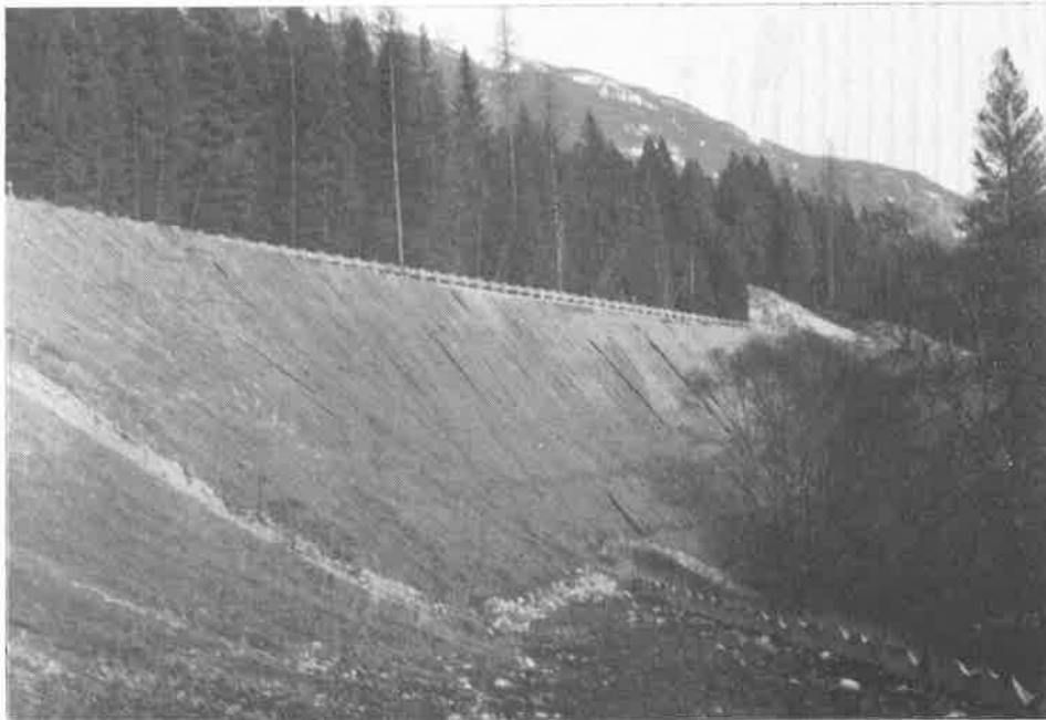
FIGURE NO. 6 - COMPLETED 1:1 GEOGRID REINFORCED EMBANKMENT WITH EROSION CONTROL FABRIC FACING - DICKEY LAKE PROJECT
