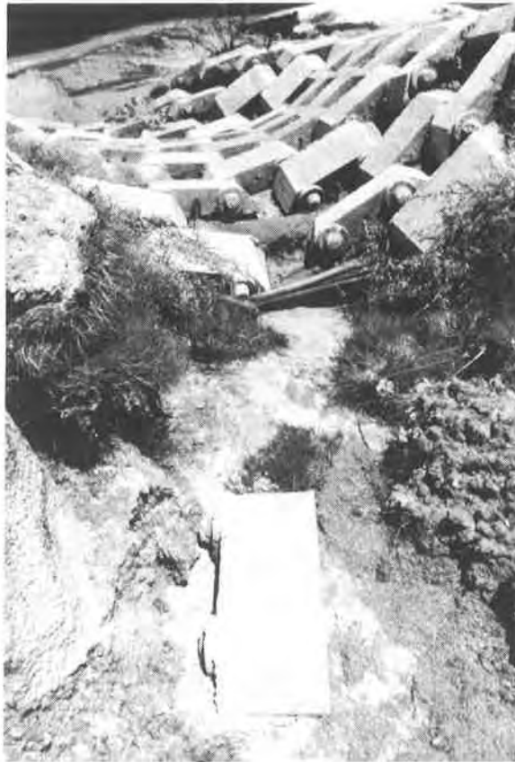
Photo 4: Example of Erosion Control Structural Problem Caused by Failure of Geotextile Underlying Interlocking Concrete Erosion Control Blocks
