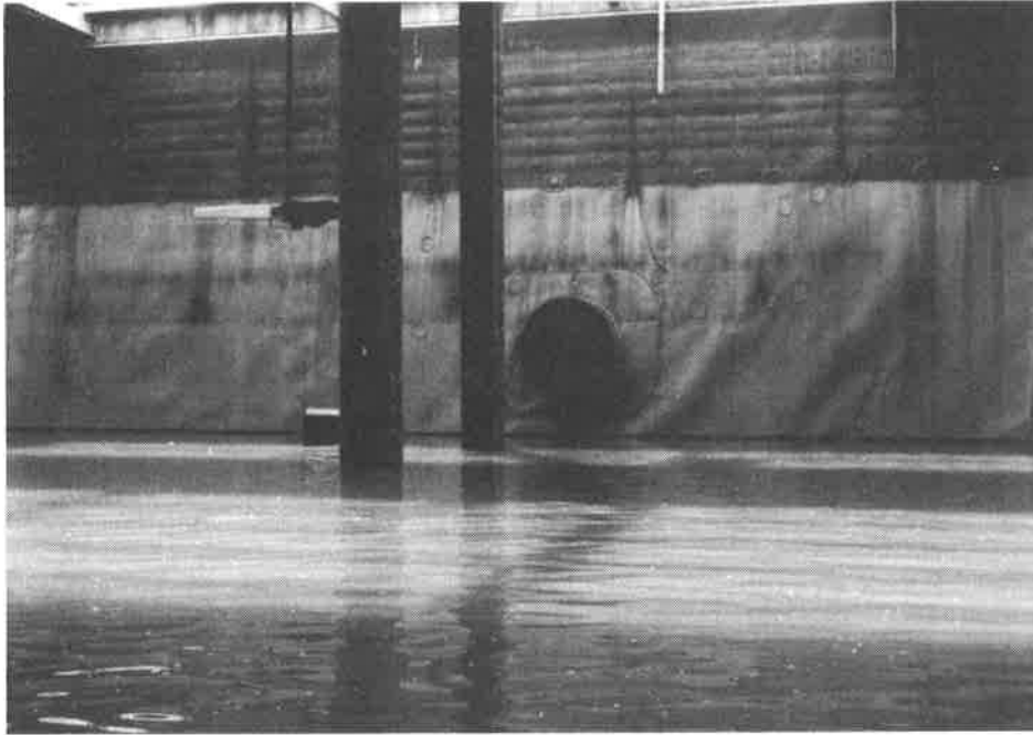
Figure 1. Geomembrane-lined basin. Agitator paddle, 2 columns, and large diameter outlet pipe are shown.
