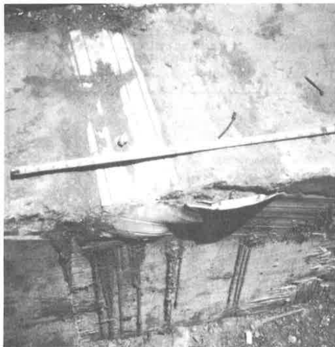
Figure 4: A geosynthetic anchor strip, compound bend at left side of inlet structure.
