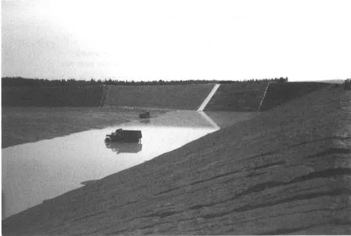
Figure 3 Water ponded at the lower end of the impoundment. Liner deployment had commenced on the northern embankment.
