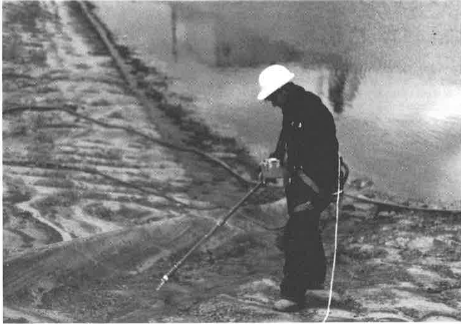
Figure 5. Searching for leaks with the water lance.
