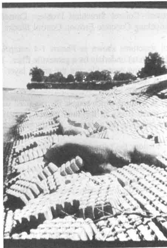
Photo 3: Example of Erosion Control Structural Problem Caused by Failure of Geotextile Underlying Concrete Erosion Control Block
