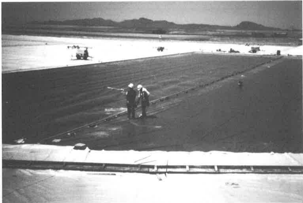
Figure 2: A section of PVC liner in the BMOR invert prior to placement of concrete cover.
