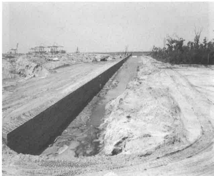
FIGURE 10. The 1,775 Feet Long Modular Block Wall Section Shown Under Construction Along the Project's Southern Boundary
