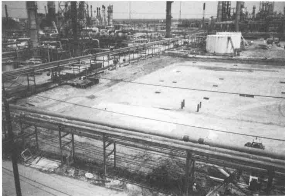
PHOTO 4: Sulphur Block Unit Site with geosynthetic reinforced crushed concrete load distribution mat in place. Ready for concrete unit paving.
