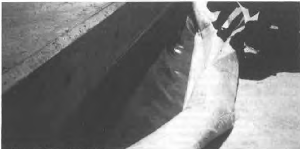
Figure 10: Geomembrane attachment to emergency spillway. An area where the installation did not have enough slack thus the geomembrane was tented.
