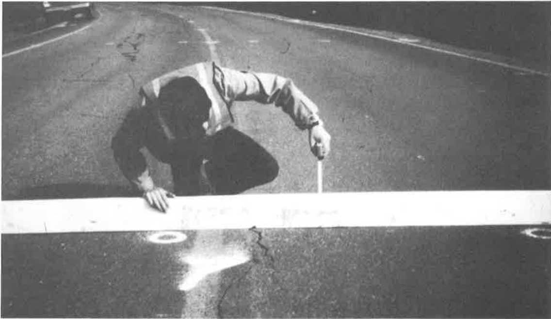
Photograph 8 - Cracks in Reinforced Section
