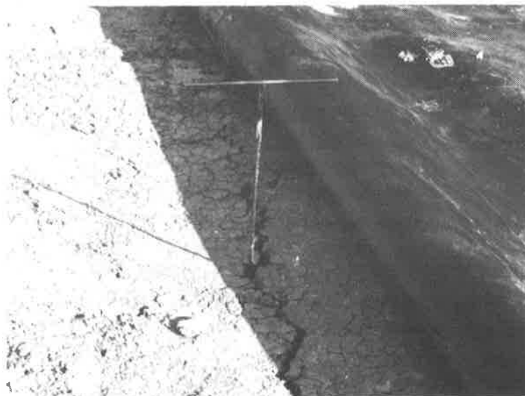
Figure 3. Cracking under the Existing Geomembrane Panels
