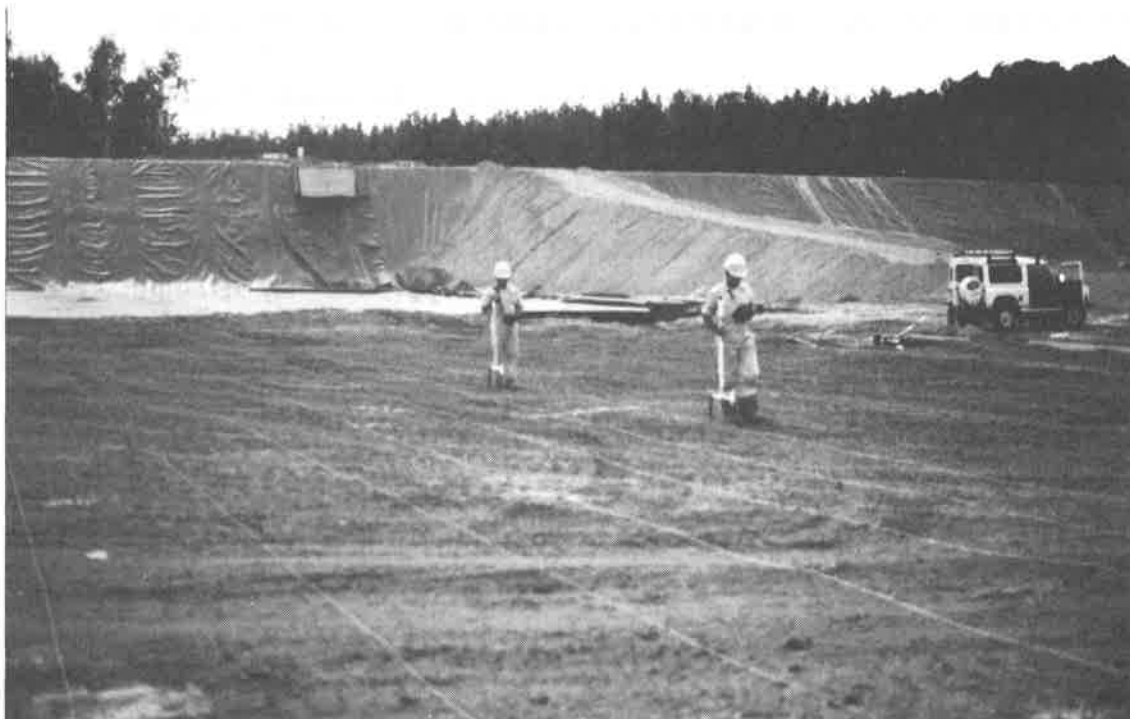
FIGURE 3. LEAK LOCATION SURVEY WITH SOIL COVER
