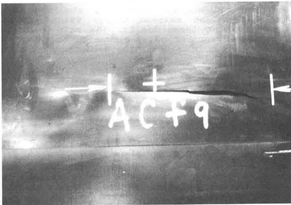
Figure 5 - Photograph of a ruptured seam
