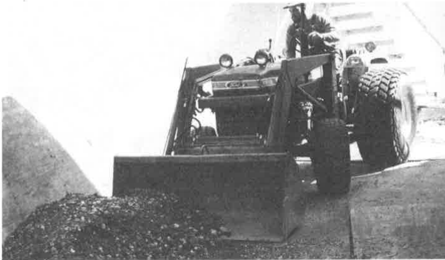
Figure 8. Soil cover placement. A minimum protection layer of 8" of soil or plywood boards were used.
