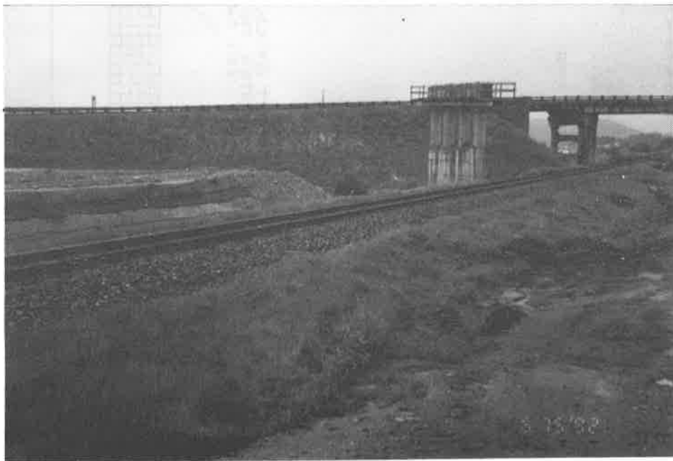
FIGURE NO. 9 - GEOGRID REINFORCED EMBANKMENT UNDER CONSTRUCTION AT BN RAILROAD OVERPASS - BOZEMAN, MONTANA
