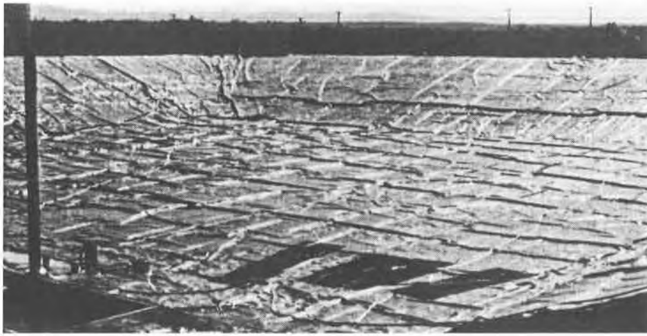
Figure 1. General view of primary liner. Note wrinkles.
