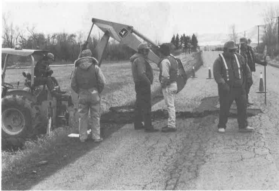
Figure 2. Pavement conditions prior to reconstruction.
