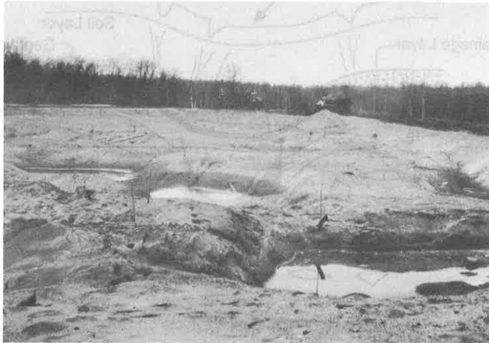
Figure 5. Results of Localized Subsidence of a Cap.
