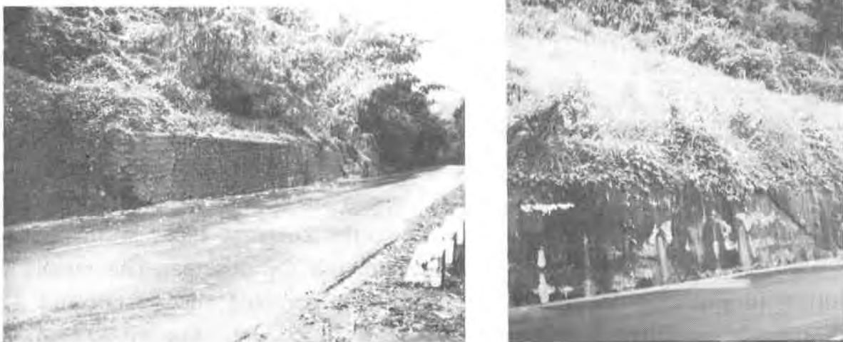
Fig. 1 Typical examples of retaining wall failure
