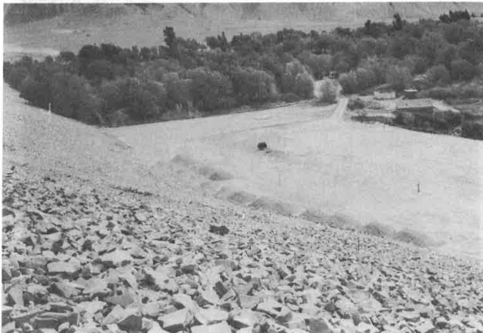
Picture 3. Placement of the overburden at the end of the construction period.
