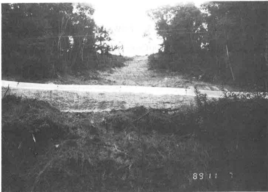
Photo 2. A view of the completed road traversing the old landslide path (November 1989).
