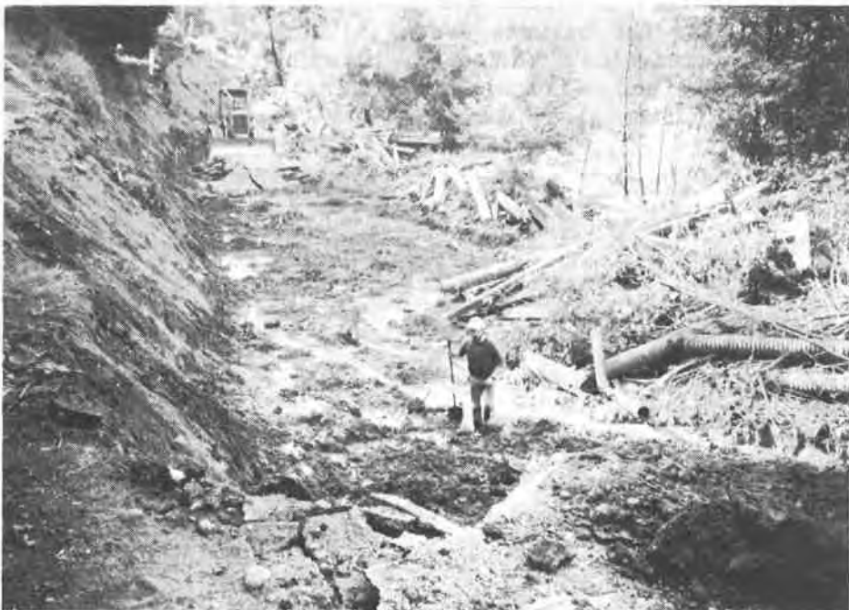
Figure 7. Saturated Soil Conditions at Elevation 50
