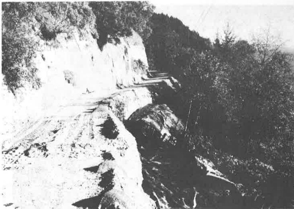
Photo 4. After excavating to the very dense underlying materials and preparing to place the first layer (September 1989).
