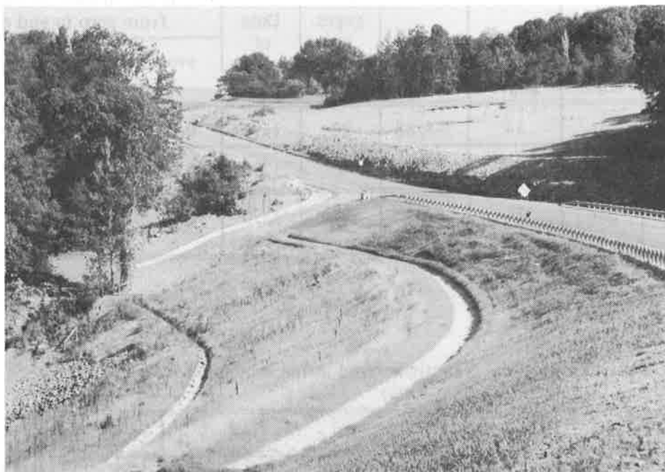
Photo 1: Completed Embankment (Note sloughing cut slopes in background).
