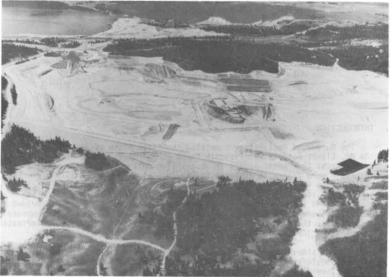
Figure 1. Aerial view taken June 1980, looking south across the Mt. Elbert Forebay Reservoir. The first portion of placed geomembrane is visible in the near right side of the reservoir and the processing plant is located in the center of the reservoir area. Also, the inlet-outlet structure (upper left-hand corner), forebay dam (foreground), slopes protection material around the perimeter of the reservoir, and subgrade areas being prepared by the contractor are visible.
