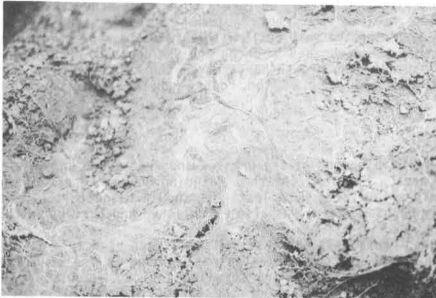
Figure 2. Root Mass at Edge of Tank
