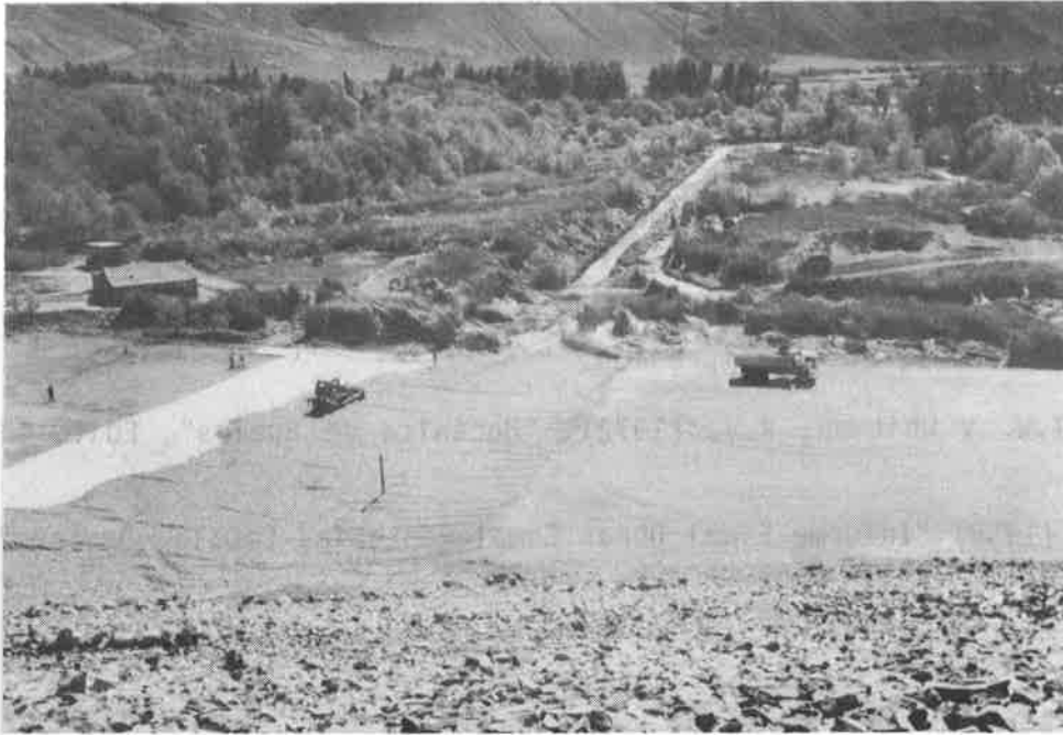
Picture 2. Placement of the drain over the geotextile during the constructive stage.
