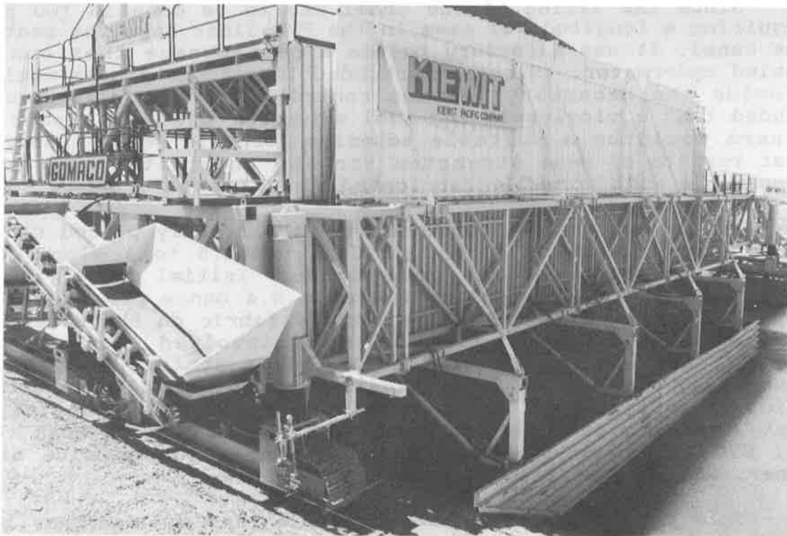
FIGURE 2. Paving Machine PVC Geomembrane was deployed and field welding performed on the top deck.
