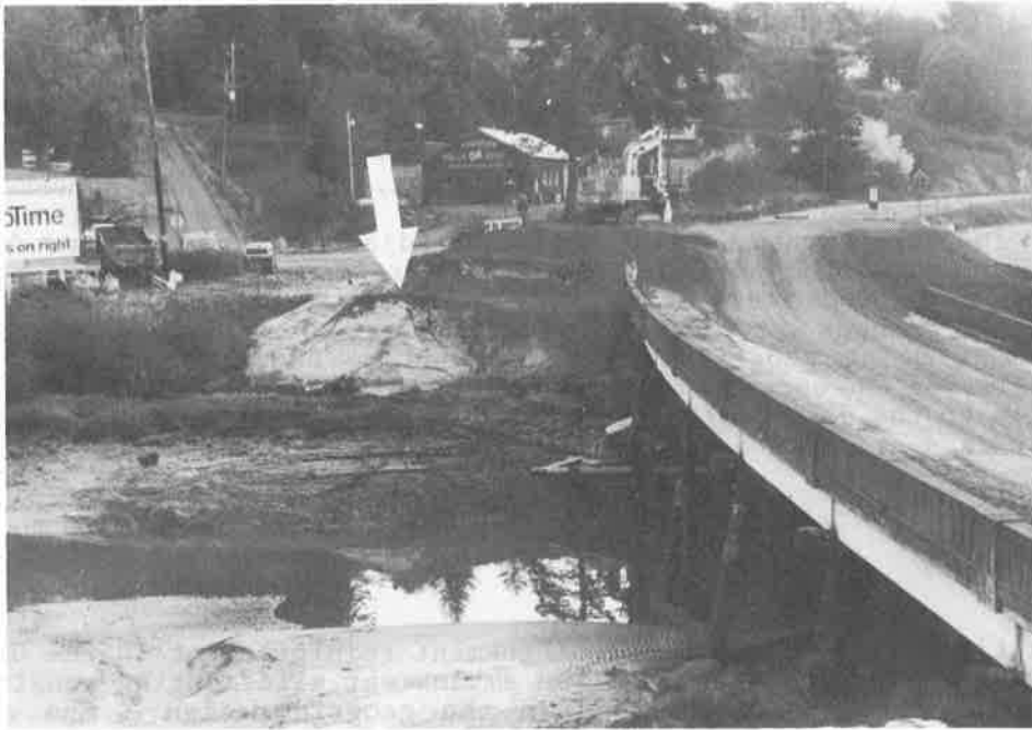
Figure 2. South Bound Approach Photo (Arrow Marks Dropped Portion of Embankment).
