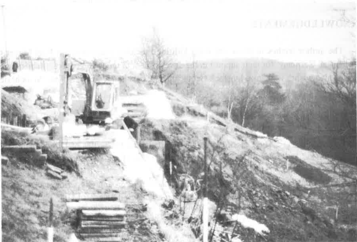
Fig.14. View of the Upper Bank Being Constructed to Re-Build the Original Crest.
