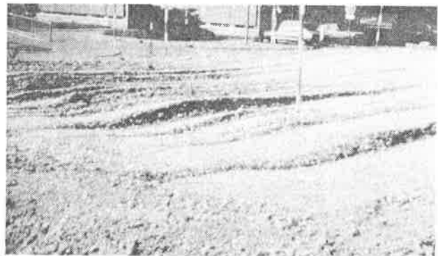
Photo 6: Deformations of the first fill layer in test field 1 with (right) and without (left) geotextile
