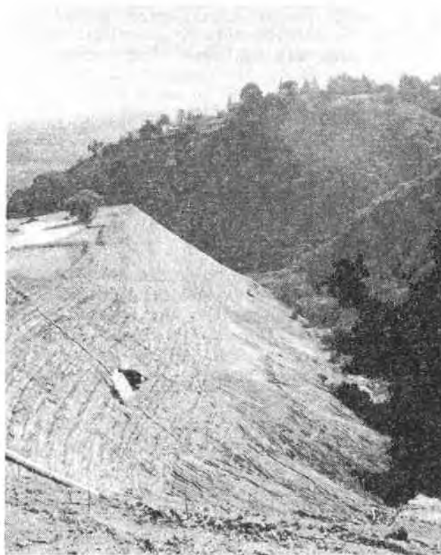
Figure 4b - A portion of completed slope. Note the instrumentation station at the foreground
