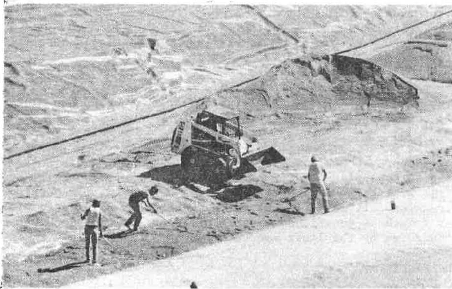
Figure 7. Front-end loader used to transport drain material to secondary leak detection pipe trenches.
