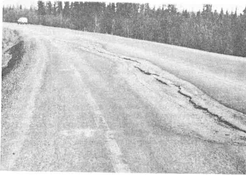
Photograph 1. Longitudinal cracks in Farmers Loop Road, Fairbanks, Alaska.
