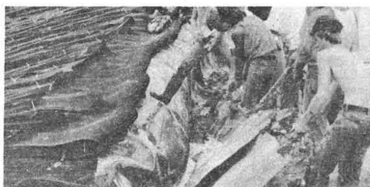
Figure 6. Pulling liner out of anchor trench to weld primary and secondary liners together.
