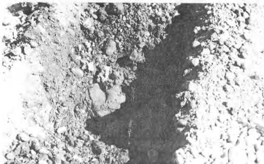
Figure 6: Severe rutting with the geotextile exposed subsequent to spring thaw.
