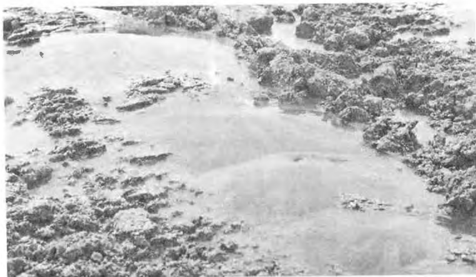
Figure 2: Piping due to excavation and construction
