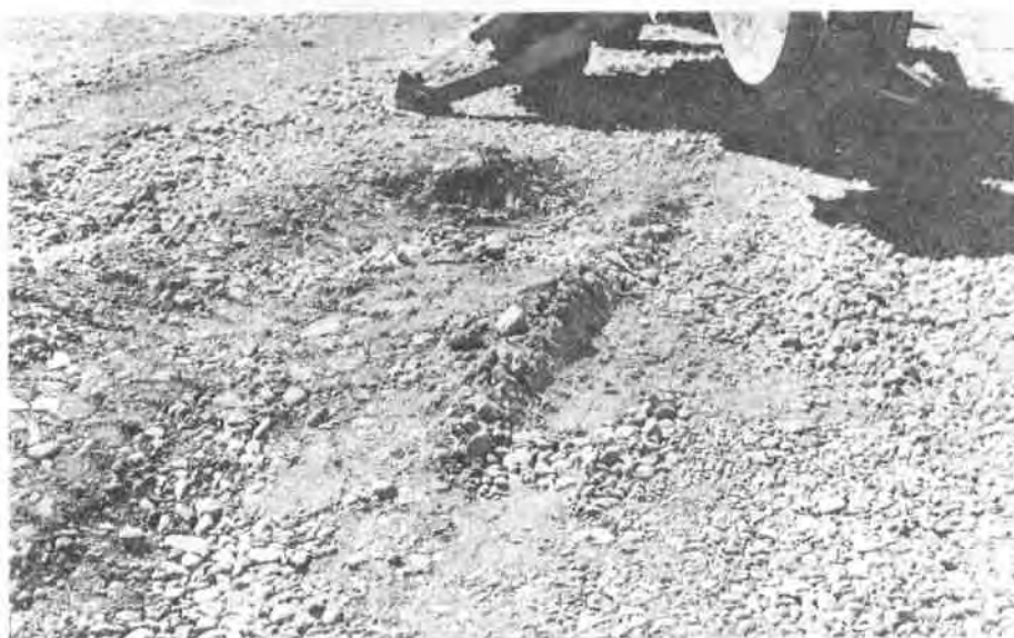
Figure 7: Minor rutting was noted primarily at corners
