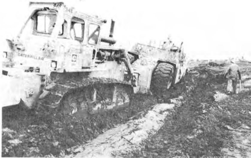
Figure 1: Example of softened subgrade during subcutting operations after precipitation
