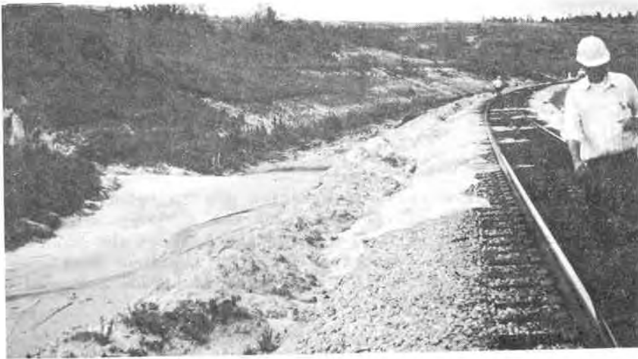
Figure 2 Condition of track structure in May, 1983, showing fouled ballast and clogged ditches.
