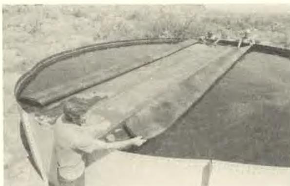
Fig. 4. Floating cover being lifted and slid across the water surface (top). Once on the water, the cover is unfolded (bottom). Folding helps prevent puncturing of the cover during installation.
