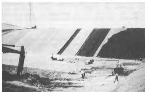
Fig. 3 Use of a plastic net over a geomembrane for leachate collection in a hazardous solid waste landfill.
