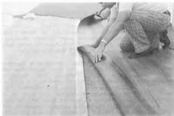
Fig. 2. Lapjointing sheet stock during the fabrication of a floating cover. Sheets must be carefully aligned.
