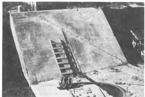
Figure 3. Side wall and bottom of the concrete pad on which the Fabridam rests showing bolts to hold the fabric and make the water tight seal to the pad.
