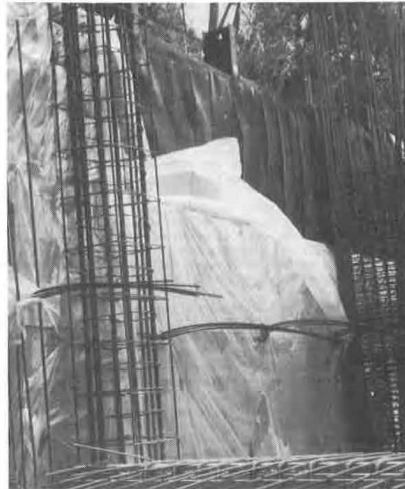
Fig. 2 Use of a plastic net drainage system with a soldier pile lagging/geomembrane system in the excavation for an underground garage.
