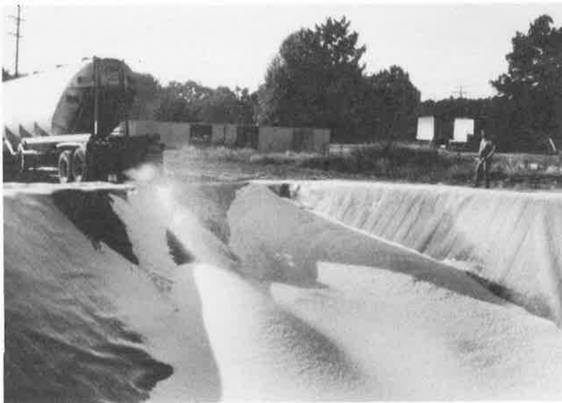
FIGURE 4 - This pond design required 140 tons of salt (NaCl) shown here being placed in the pond.
