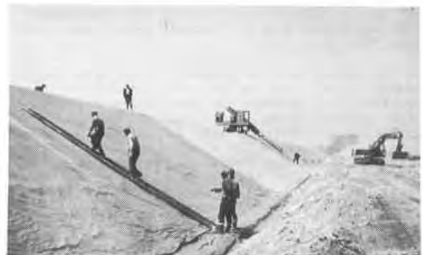
Fig.4: Foils on the slope: along the ladder a construction joint is being made; trimming in background
