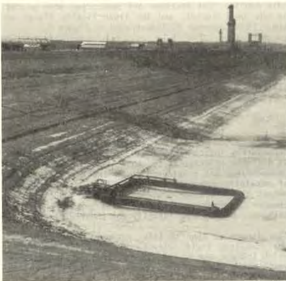
Figure 3: View of south side of pond. Note darker area in southwest corner of remedial clay liner, untrafficked brine sludge on base of pond.
