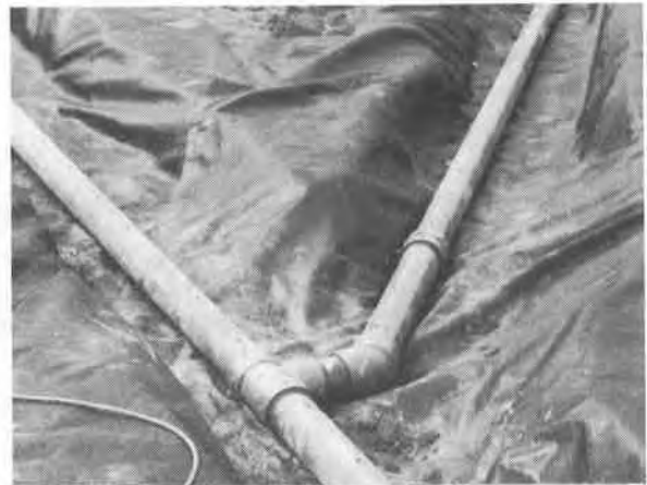
FIGURE 7: LEACHATE COLLECTION DRAIN PIPE
