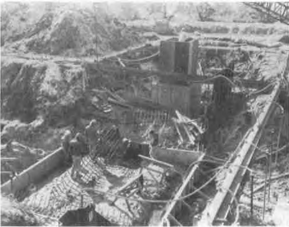
Figure 2. Early construction phase of the Fabridam showing the by-pass channel in background, the interlocking sheet piling, the well point system for dewatering and the third pour conditions for the vault building.
