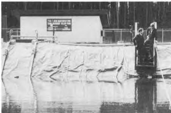
Biogas Collection Cover
