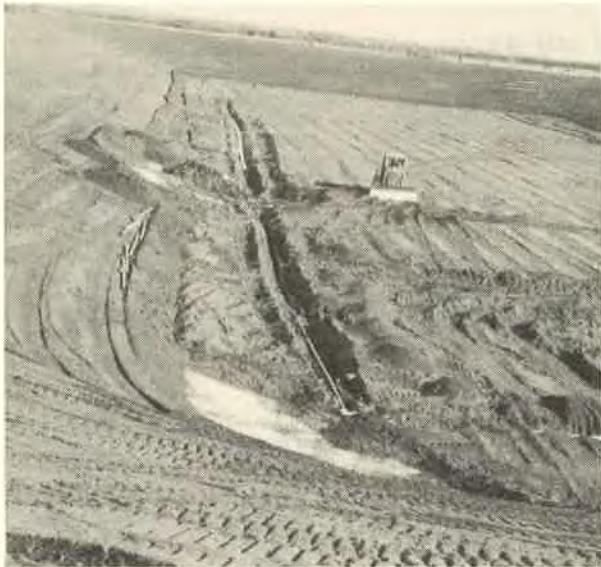
Figure 5: Placement of sand bed onto geotextile, and installation of ventilation and collection piping.
