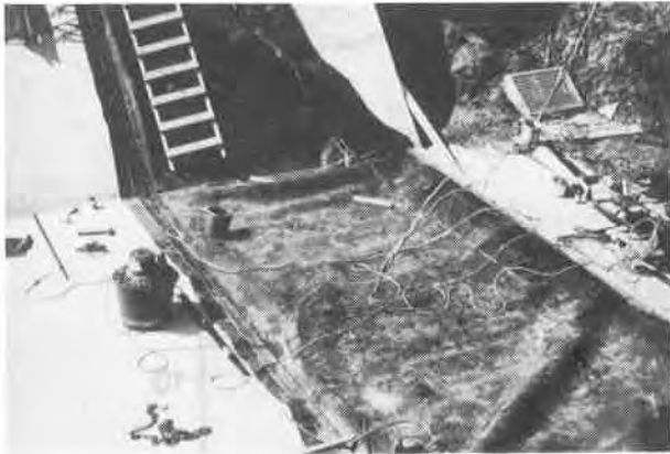
Figure 4. The excess fabric of the Fabridam was folded to form a smooth surface for the dam to rest on when deflated.
