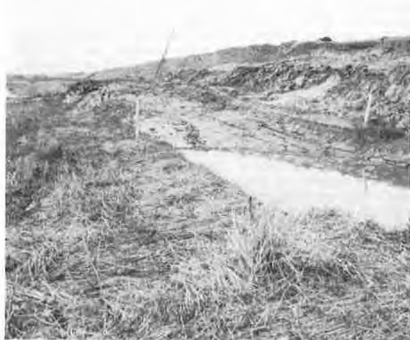
Photo 3 Failure of retaining bank due to sliding along a circular surface, north-south, at 11.00 a.m., at reference line I. Note the start of this surface of sliding at the crest of the retaining bank. The hydraulic placing pipeline had now suddenly come into view.
