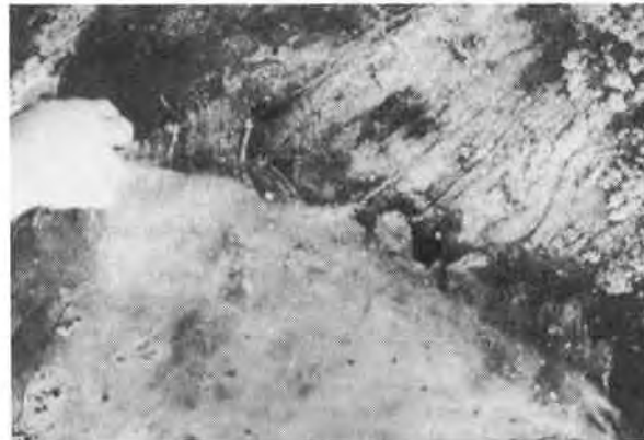
Fig. 7. Fabric failure in Holland highway embankment
