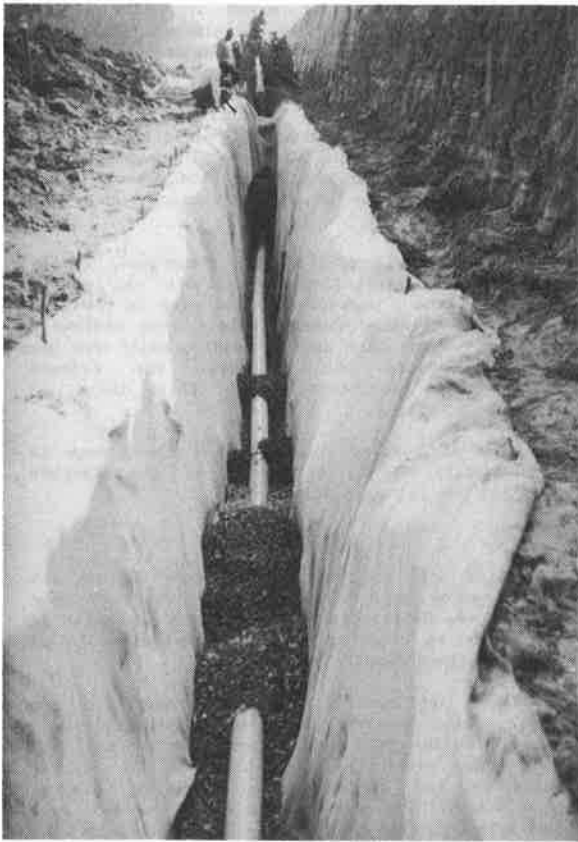
Photo 5 : Toe drain under construction - Fabric laid in excavated trench, slotted pipe inserted and stone filling started.
