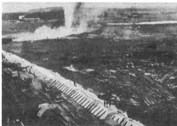
Phot.1 Constructed embankment of reservoir I, in background from east, to the right side from south along the highway from Karlino to Koszalin.
