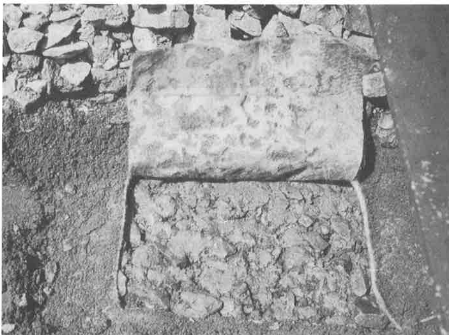
Fig. 9 Non-woven fabric uncover- ed after 7 years under railway - running (a pro- tective layer of 7 cm sand had been laid bet- ween geotextile and sharp-edged stonyballast).
