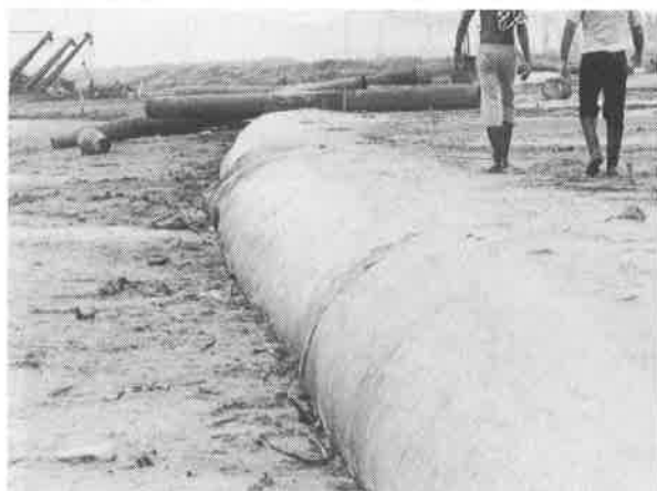
Figure 8 - Finished dike and landfill; the filled area to the right and site of the future lake to the left.
