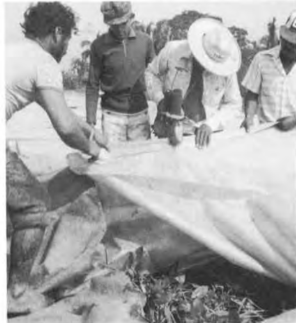
Photo 1 Aspect of Geotextile sewn on-site with electric portable bag closing machines and 1050 denier polypropylene thread.
