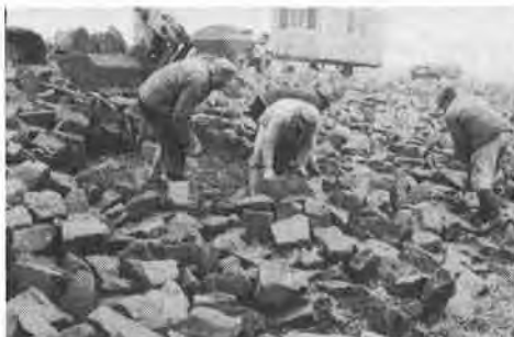
Fig. 2 Digging out a fabric at a seadike revetment at the Northfrisian coast
