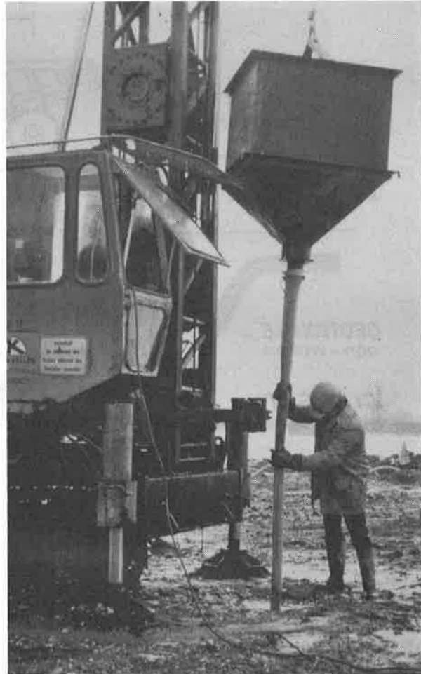
Fig. 4 Lowering of a vertical non-woven drain (filled with 2/7 mm - sand) into the borehole.
