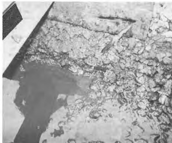
FIGURE 4 TRACK AT FIG. 3 GEOTEXTILE LEVEL
