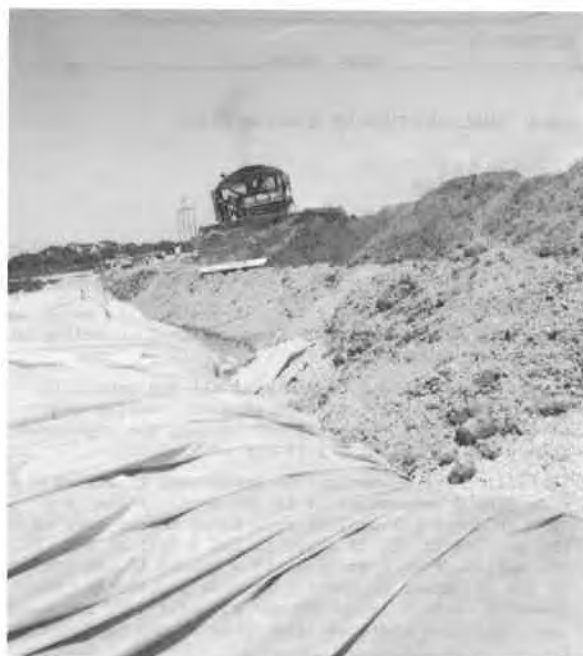
Photo 3 Material is spread out from the center to the sides following an arrow attack type of loading. Displacement of the peat can be seen.
