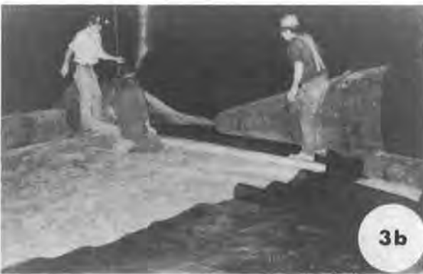
Fig. 3 Use of geotextiles in drainage systems associated with geomembranes: (a) geotextile being sewn to form a sleeve acting as a filter around a flexible perforated pipe used for draining gases; (b) plastic net (black, on the right of the photograph) acting as a drain, placed on a nonwoven filter (grey, on the left) and eventually covered by a geomembrane (roll in the background).
