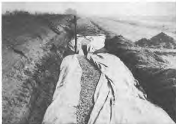
Photo 4 : Crown Sand Slimes Disposal - Filter drain under construction with fabric turned back to expose the stone.
