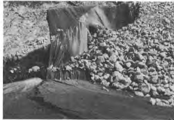
Fig. 5 Typical Slope Protection Failure Related to Tears in Filter Fabric
