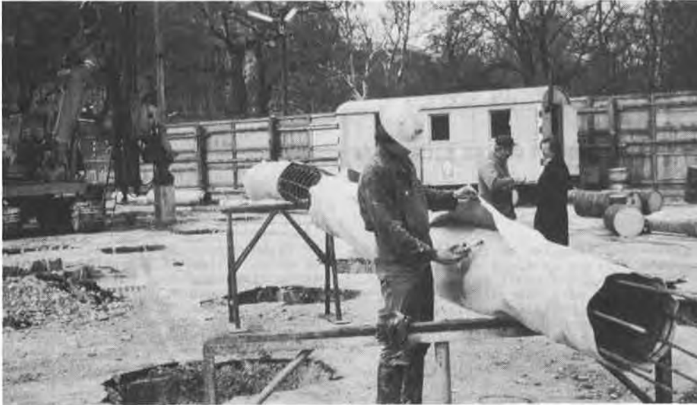
Fig. 1 Encasement of the reinforcement cage of a bored pile with a non-woven geotextile; welding of the longitudinal overlap with a blow torch.
