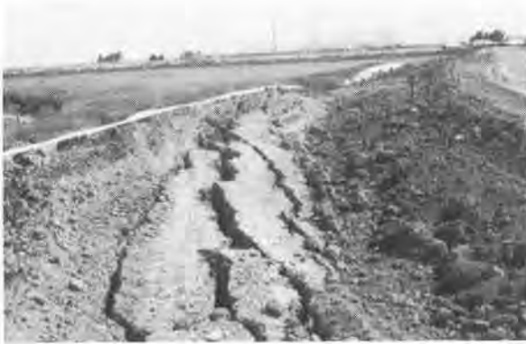
Photo 4 View showing pushup beyond slope toe of containment dike.
