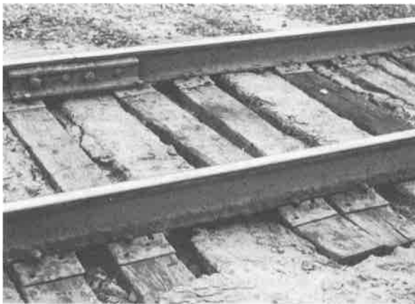
Figure 1. Typical Pumping Track Ballast Completely Fouled
