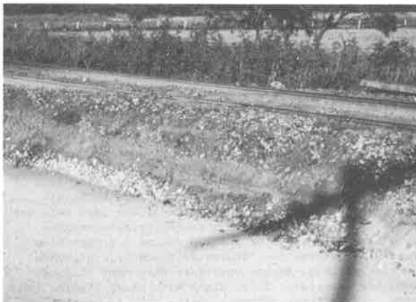
Figure 2. Side View of Mud Migrated Into Ballast
