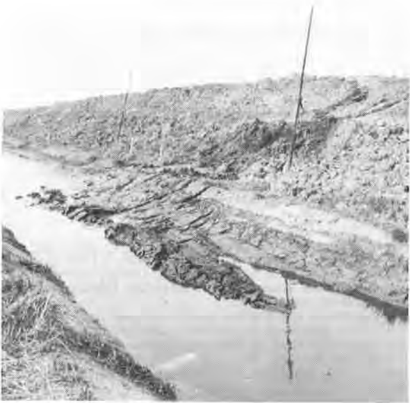
Photo 2 Bottom of ditch heaves forcibly at reference line I, north-south, at 09.45 a.m.
