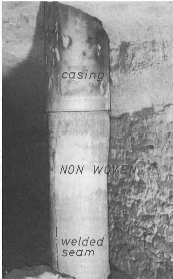
Fig. 3 Bored pile ( \varnothing 90 cm) with the reinforcement encased with a non-woven geotextile, during the tensioning of the pipe encasing in an old cellar passage (loess-subsoil).
