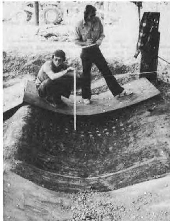
Fig. 4 Catenary sag and bulges of geotextile beneath rutted aggregate surface.
