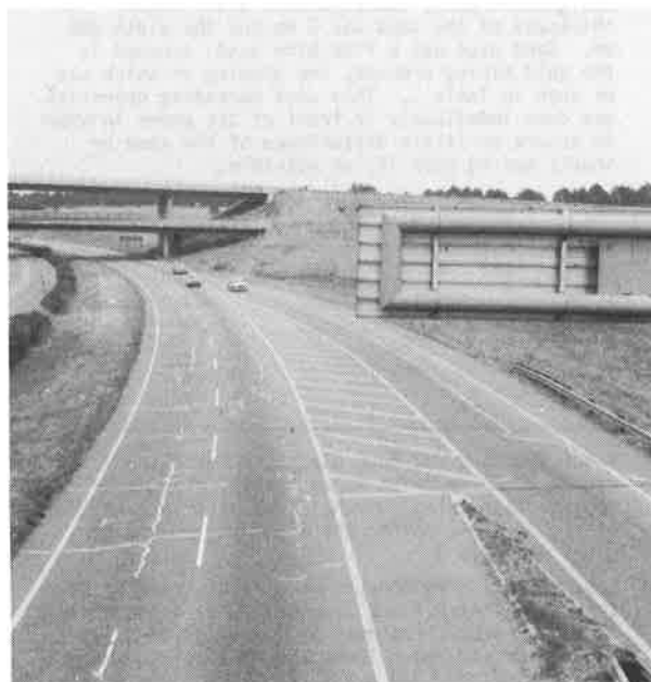
Fig. 5 Cracks demarcated with Lime during a Survey February 1982
