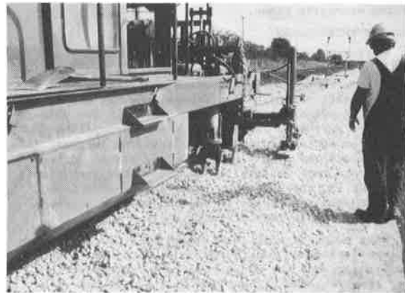
Figure 8. Ballast Tamper Compacting Ballast with Tamper Feet Being Closely Observed for Geotextile Damage.
