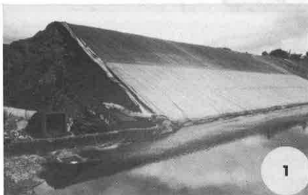
Fig. 1 Dike failure due a sinkhole caused by water leaking from the pond.
