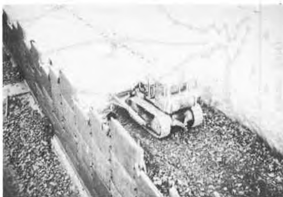
Fig. 1 Jersey wall under construction. Rock fill being placed over Paraweb and Terram
