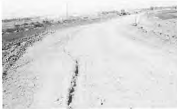
Photo 5 View showing longitudinal crack near centerline of containment dike.
