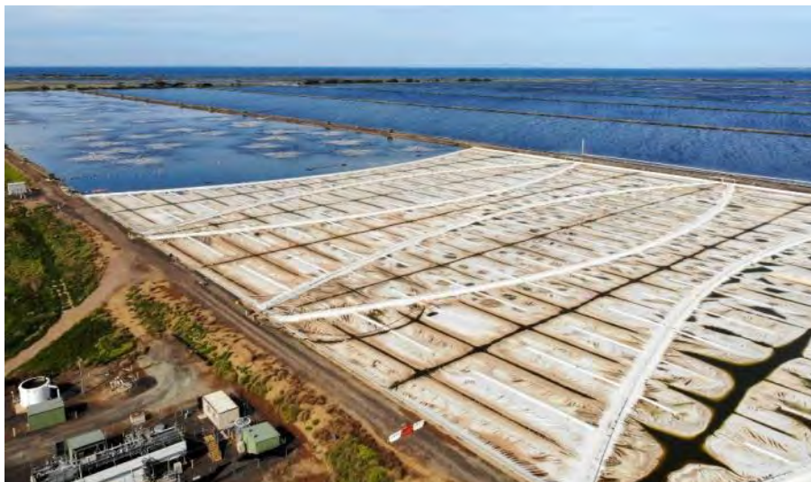
Figure 2. HDPE Floating cover on the anaerobic section of a wastewater treatment lagoon capturing biogas and eliminating odors. An energy company has an offtake agreement with the municipal water authority to use the gas to generate electricity. Victoria, Australia. (Image: Melbourne Water, 2021)
