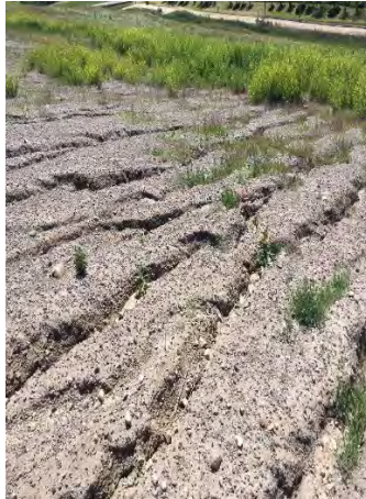
Figure 2 – Erosion Rills In Need Of Grading For An EGC Subgrade Preparation
