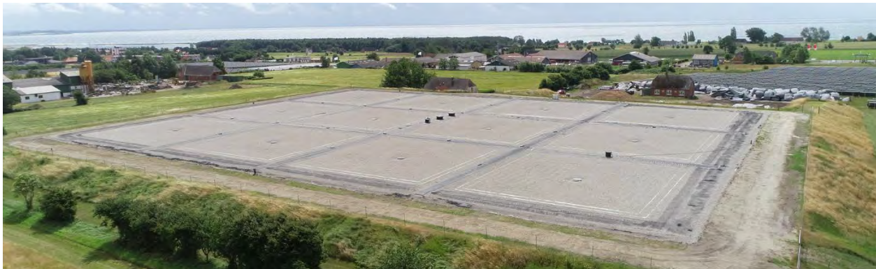
Figure 10. Insulated floating cover on a hot water thermal pit. Marstal, Denmark. (Image: AalborgCSP, 2019).
