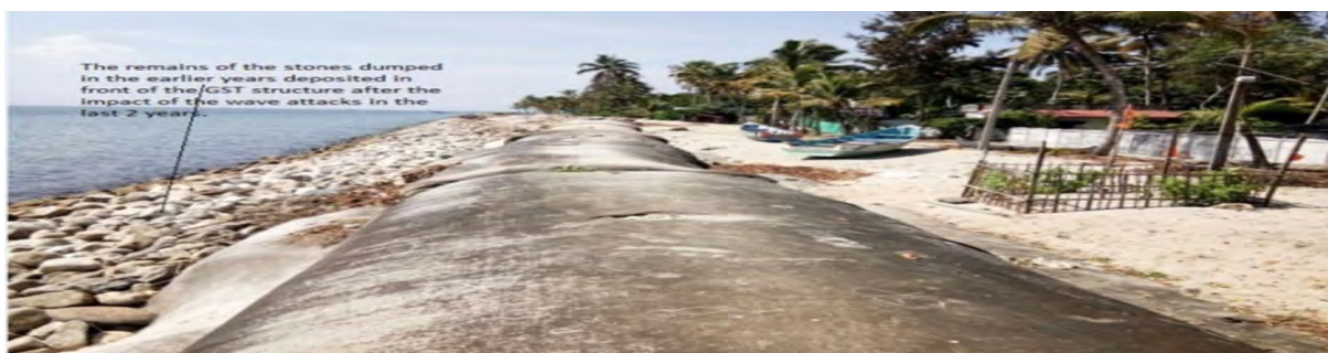
Figure 9. Geosynthetic Tubes as Seawalls for Coastal Protection, at Vypeen Reach. (Source: KID)
