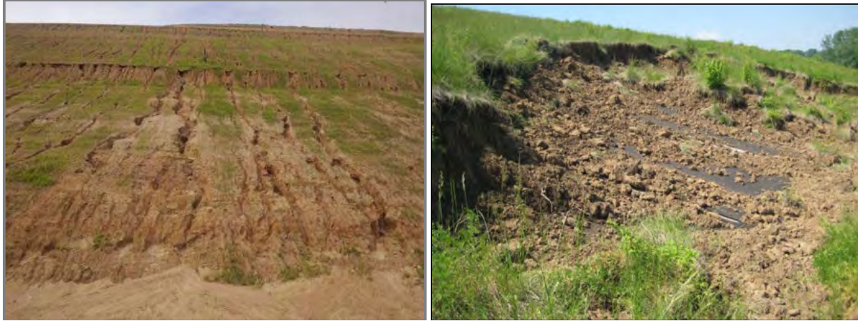
Figure 7. (a) Poor vegetation and erosion gullies on traditional soil cover (b) Veneer slope failure of traditional soil cover (Maier, 2012).
