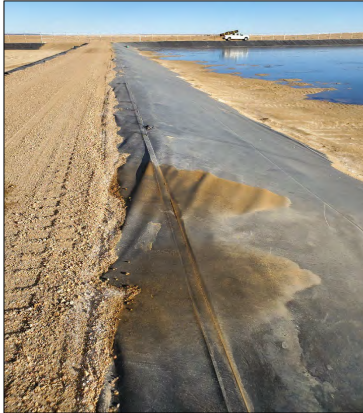
Figure 1. Hydrocarbon spills on geosynthetics for a water reservoir, which indicates driving too close to the geosynthetics.
