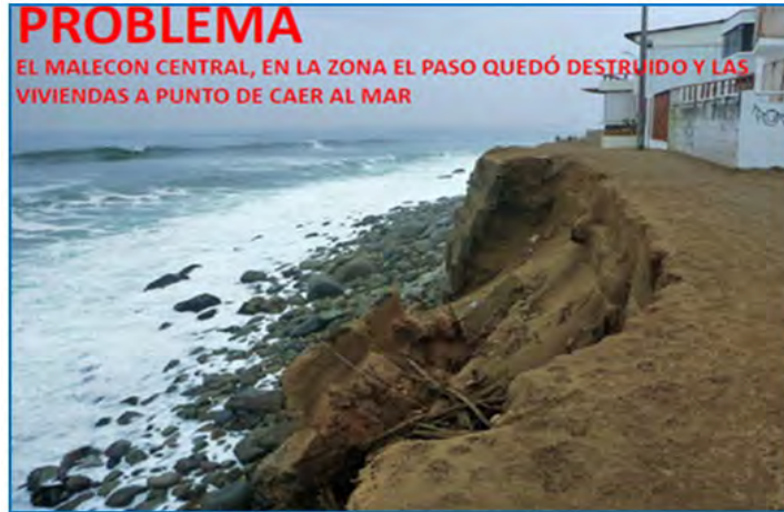
Figure 21. Collapsing shoreline required immediate protection
