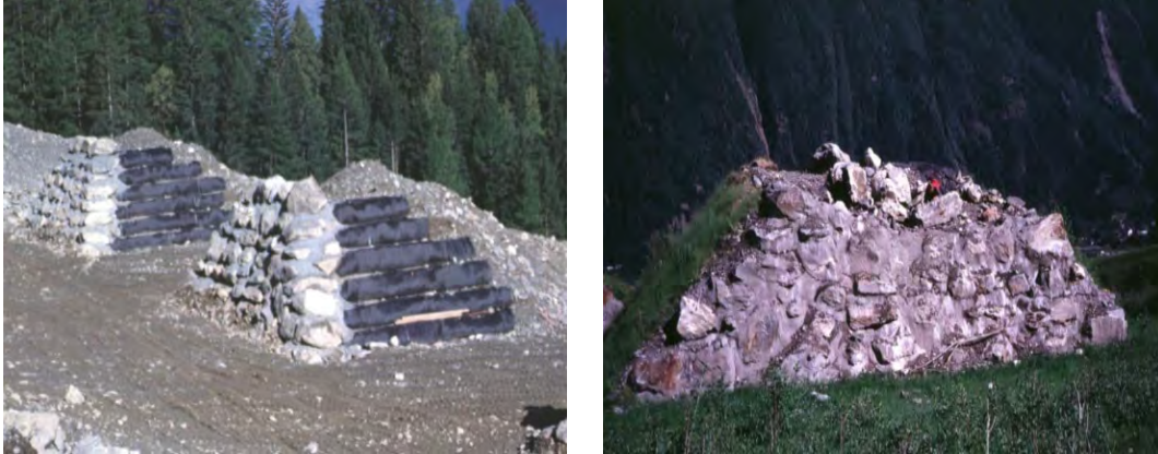
Figure 7. Avalanche breaking mound after completion (left) and after partial destruction (right). Location: Taconnaz, France. (J.M. Tacnet, INRAE).
