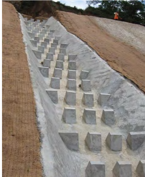
Figure 1. Energy dissipaters incorporated as part of a concrete-filled geocell mine channel, Peru
