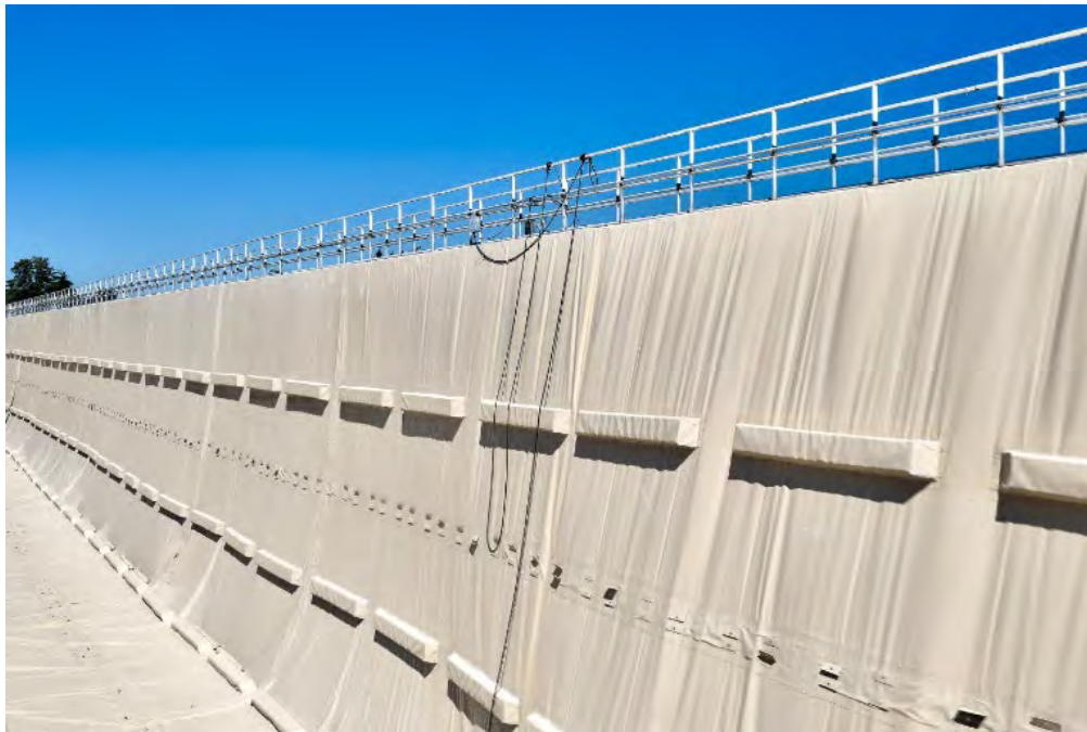
Figure 2. Installation underway of double trough system on 28-foot divider wall on west cell
