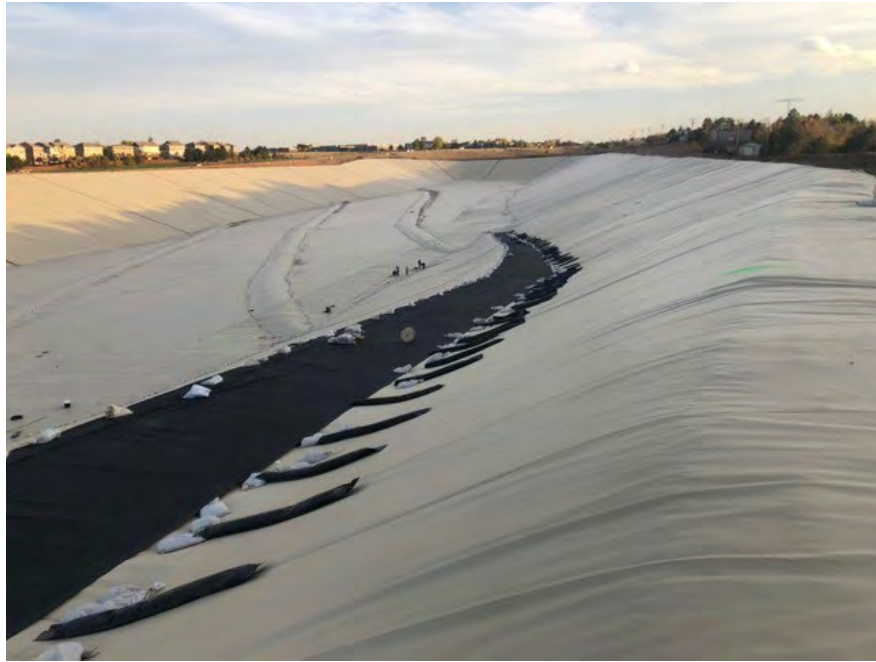
Figure 3. Typical black safety ladder for reservoir ingress and egress
