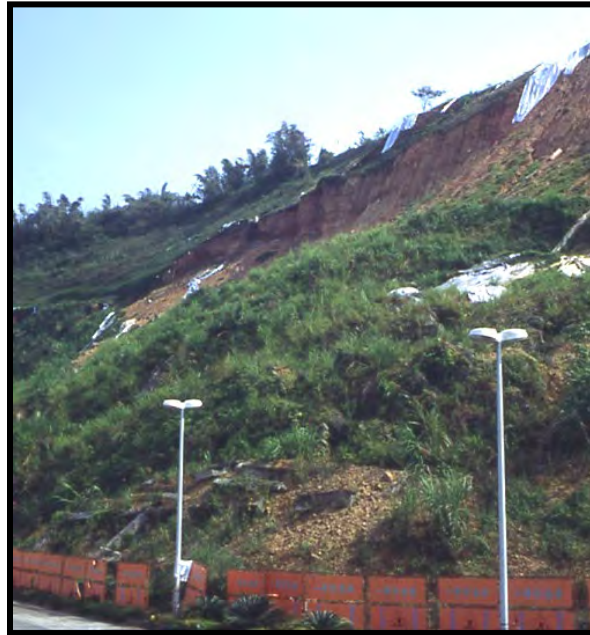
Figure 1. Photo of the failed slope.
