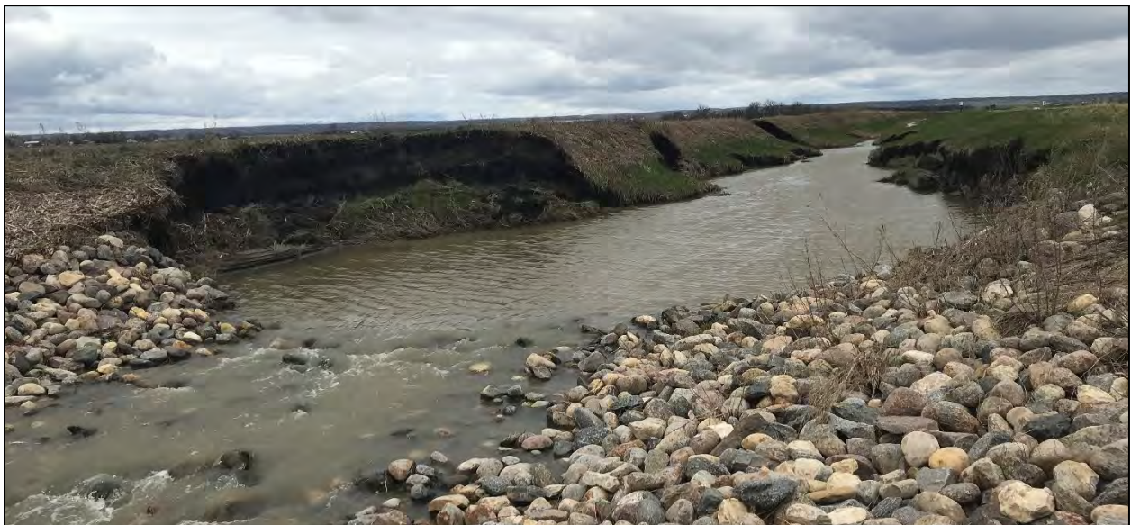
Figure 12. Unreinforced Section showing erosion and geotechnical failures after storm event - Upstream Section (05/2022)
