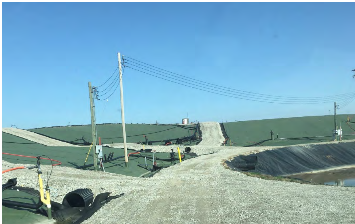
Figure 7 – Roads Overlying an EGC Used for Anchorage and O & M Access Activities
