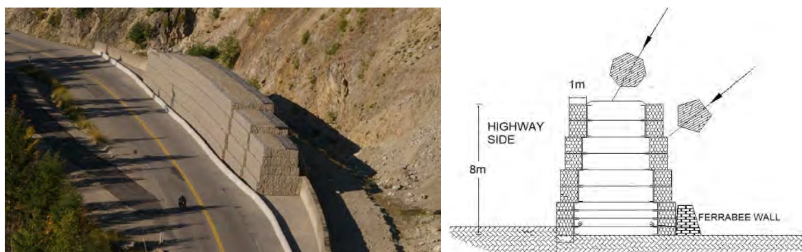
Figure 2. Rockfall protection embankment along the Trans-Canada highway. General view and cross-section (adapted from Simons et al., 2010).
