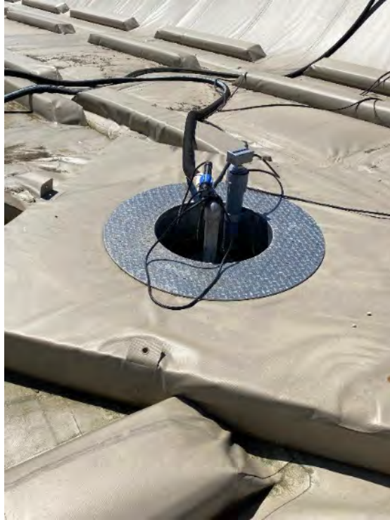
Figure 4 – Rainwater Removal System
