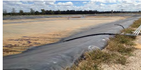
Figure 6. 1.00mm proprietary polyolefin floating cover on syngas process water to eliminate odors and rainfall ingress. Qld, Australia. (Image: A. Gersch, 2015)
