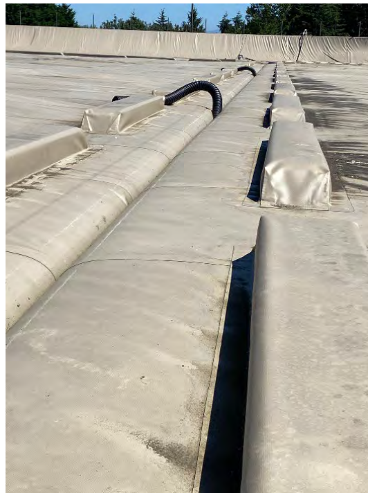
Figure 9. East cell trough & floats in service
