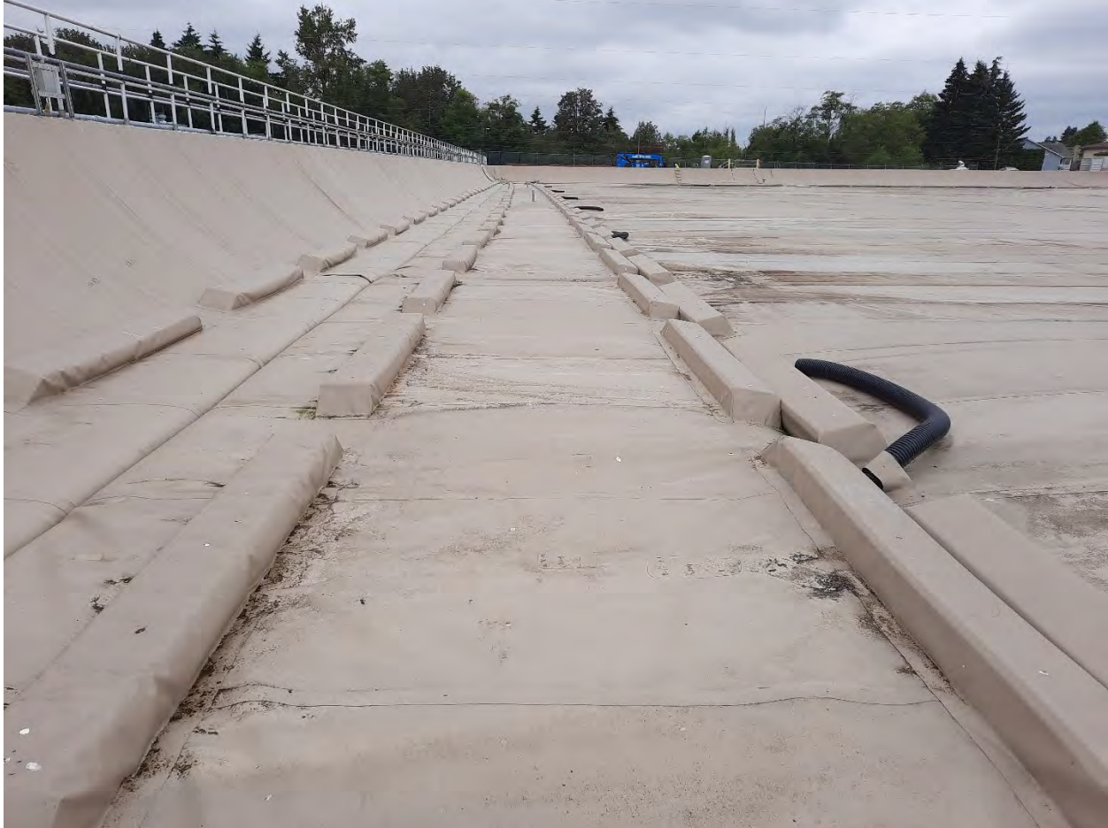
Figure 3. East Cell divider wall trough in full service
