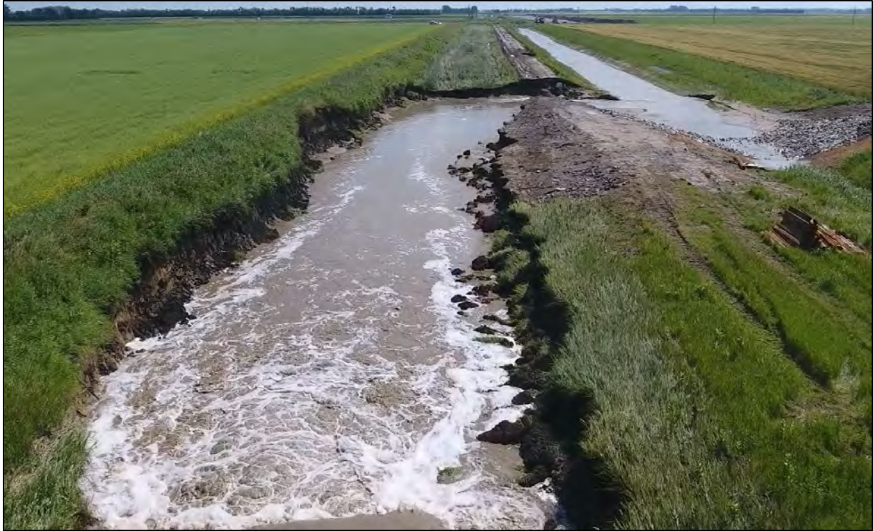
Figure 1. Channel Erosion prior to remediation.
