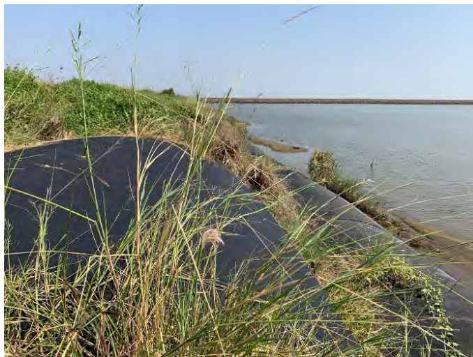
Figure 16. Vegetation growth over the sand filled mattress and geotextile tube.
