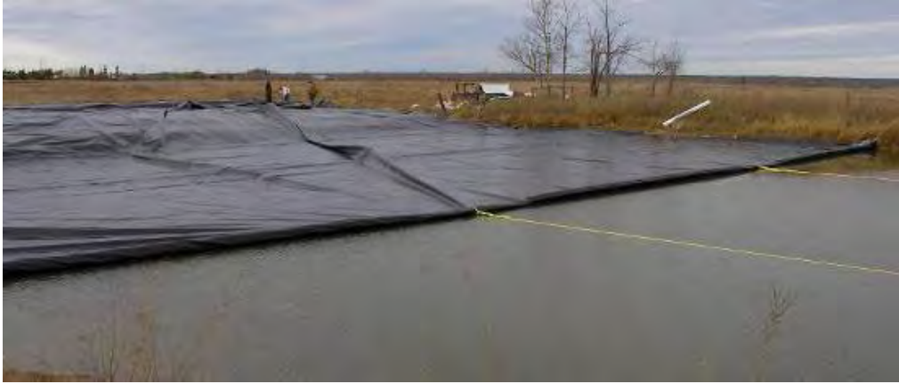
Figure 8. Floating cover being pulled into place with rope and reinforced leading edge.
