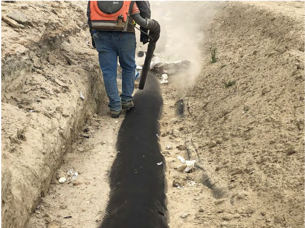
Figure 3. Backpack Leaf Blower Used to Dry out the Geocomposite in the Perimeter Isolation Gap.
