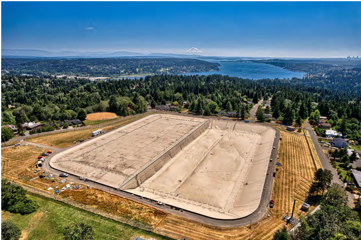
Figure 1. Aerial view of the completed east cell (left side) completed in 2021 and west cell (right side) reservoir under construction in July 2022
