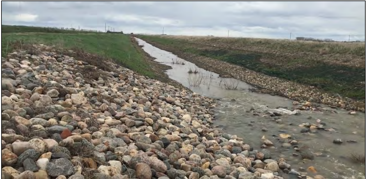
Figure 11. Gabion Mattress and EEAS Performing after storm event - Downstream Section (05/2022)
