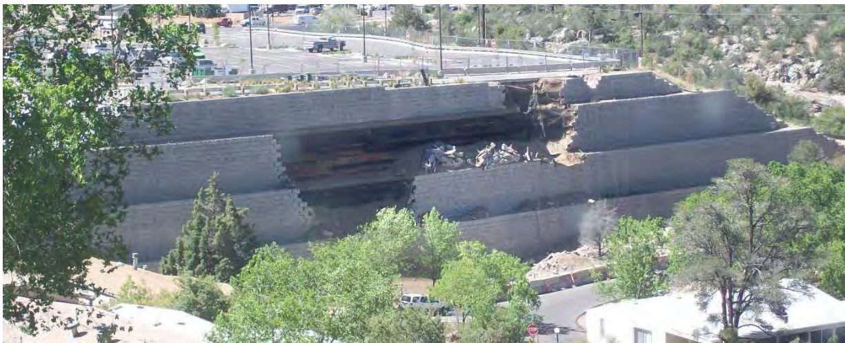
Figure 3. The failure shown several days later.
