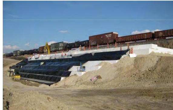
Figure 8. Geomembrane over Geofoam in Railway application. Salt Lake City UT USA. Source: University of Utah
