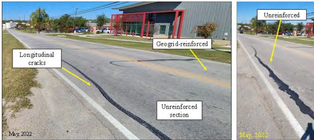
Figure 6. Road conditions during 2022 survey.
