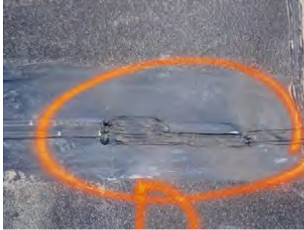
Photo 1. Untrained installation technician created “Gorilla bead”.
