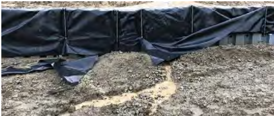
Figure 9. Seepage under the barrier wall.
