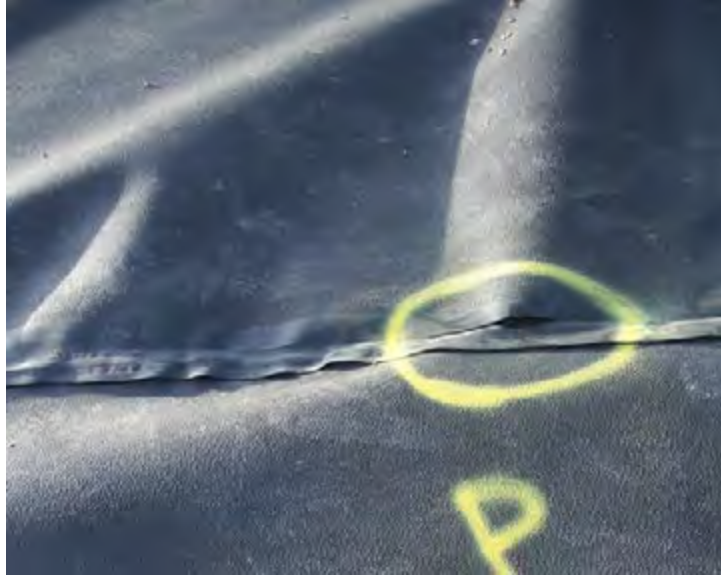
Photo 3. Improper pressure should have been observed by operator.
