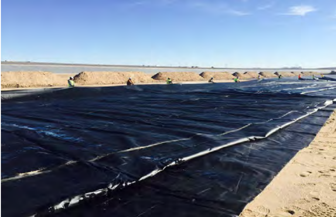
Figure 3. Photo showing large fPP-R panel unfolding and positioning on bottom. Note soil cover material staged for immediate placement after tie-in seaming
