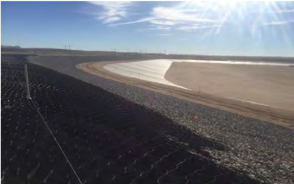
Figure 2. North End of reservoir showing from top to bottom – Geocell, 2 inch stone infill, soil covered bench, lower exposed section and finished bottom soil cover
