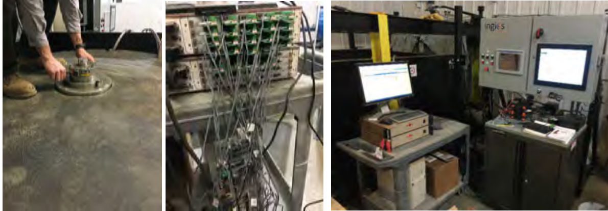
d) e) f) Figure 4. Illustration of the a) subgrade preparation, b) setting geogrids, c) base layer preparation and compaction, d) surface layers preparation, e and f) setting the data logger
