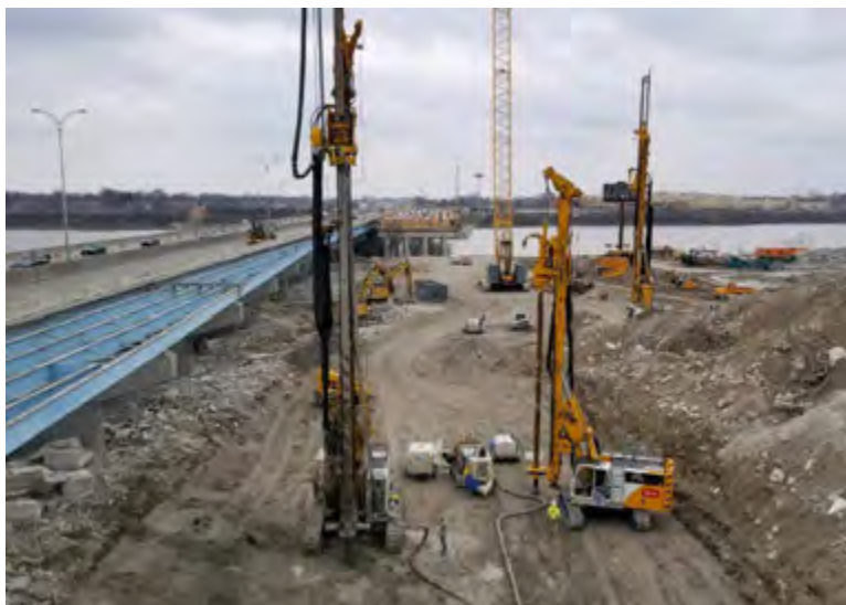
Figure 7. CMC rigid inclusion installation at the DiSalle Bridge Replacement Project. (source: Menard Group USA)
