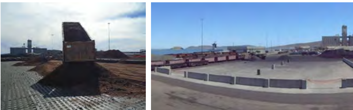
(a) (b) Figure 4. Laying down of fill material (a) and view of completed storage area (b).
