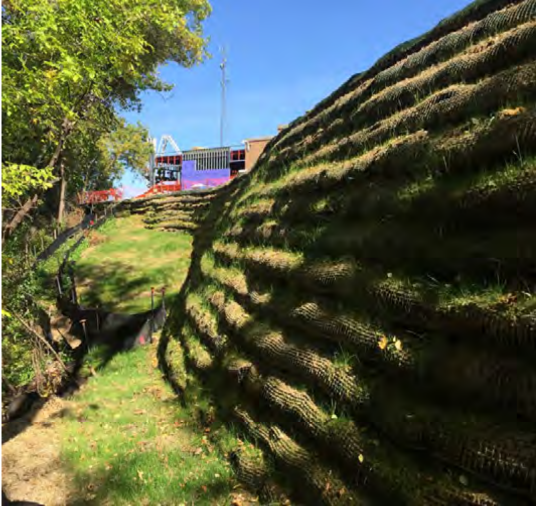
Figure 9. Portion of GRW wall at Mounds View HS a few weeks after hydroseeding.
