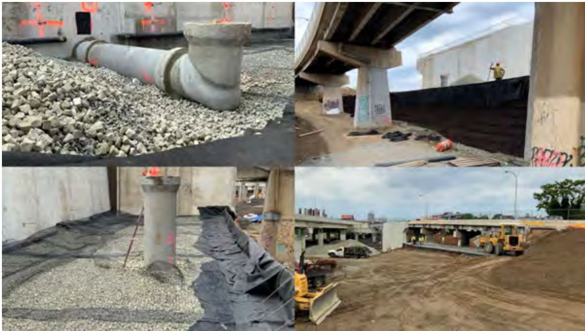
Figure 5. Photographs of MSE with UL-FGA backfill construction at Section GR4 of I-95 in Philadelphia, PA.
