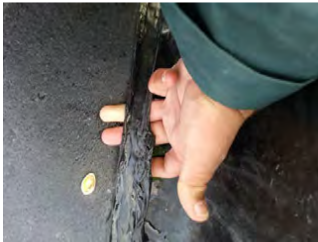
Photo 4. Tired crew did not abraird HDPE geomembrane prior to extrusion weld.
