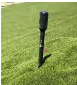
Figure 12. Pressure relief valve for engineered turf cover.
