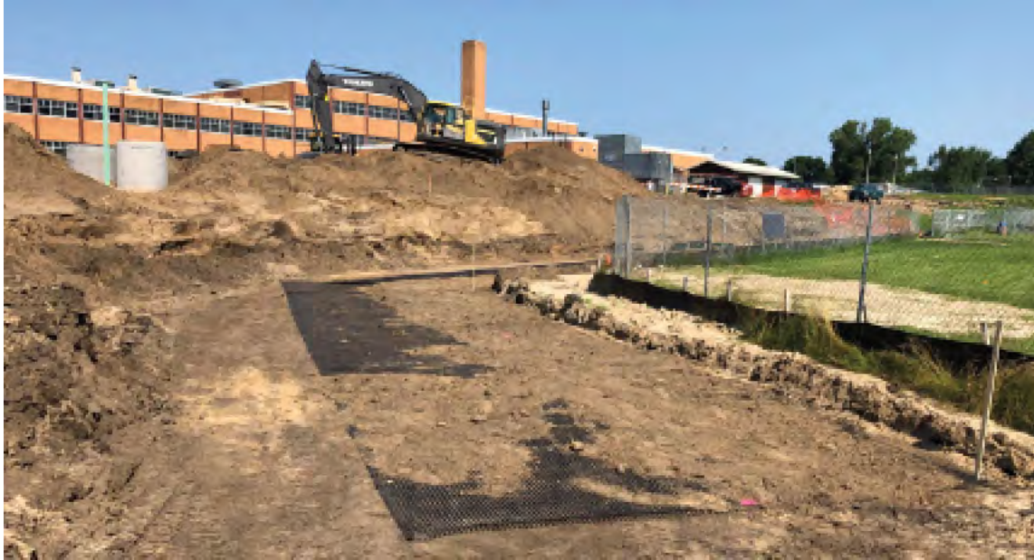
Figure 2. Subgrade pad and first layer of geogrid at Edgewood MS wall project.
