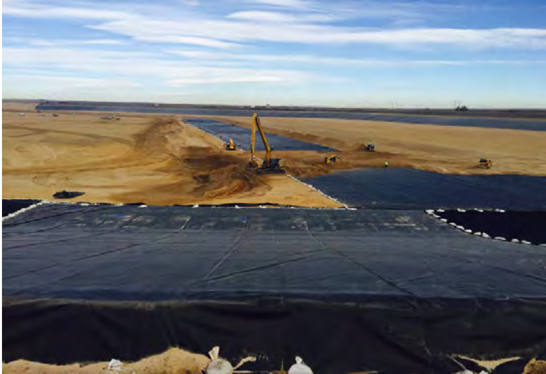
Figure 1. North End of reservoir showing slope panels transitioned into bottom panels and staged cover soils placement on bottom panels
