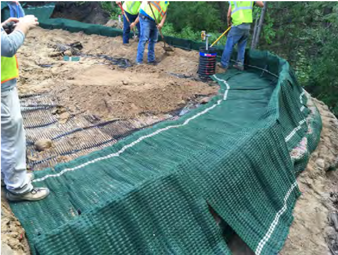
Figure 7. Backfilling a geosynthetic lift for a reinforced soil slope section at the Mounds View HS project.
