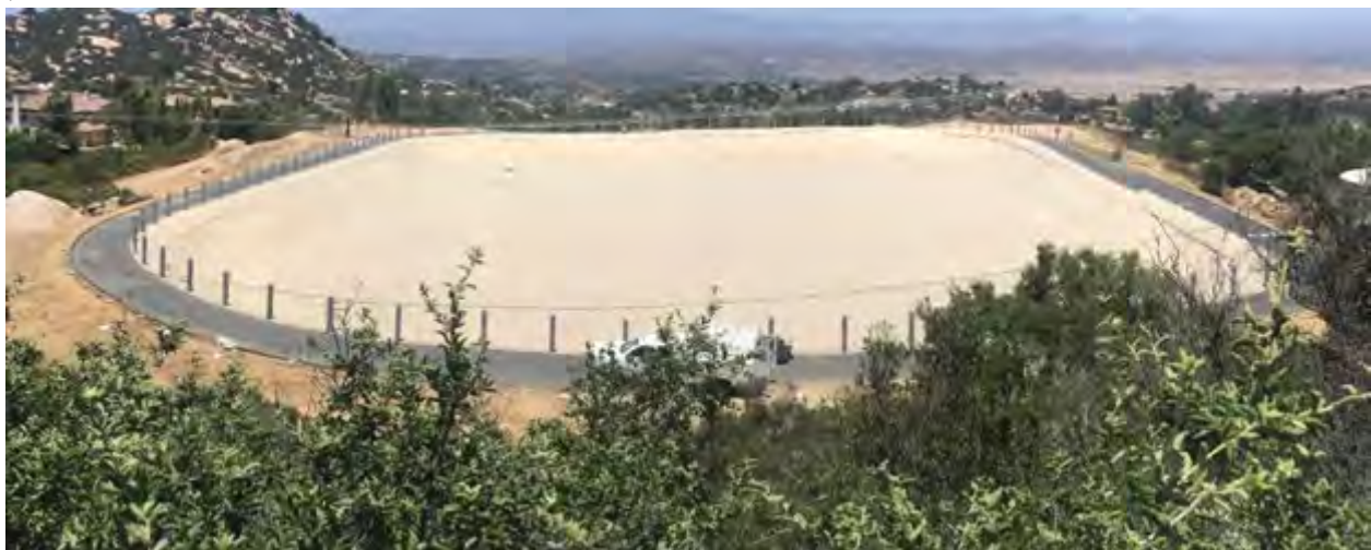
Figure 1. Ramona Water District. CSPE Tension Cable Systems installed in 2020
