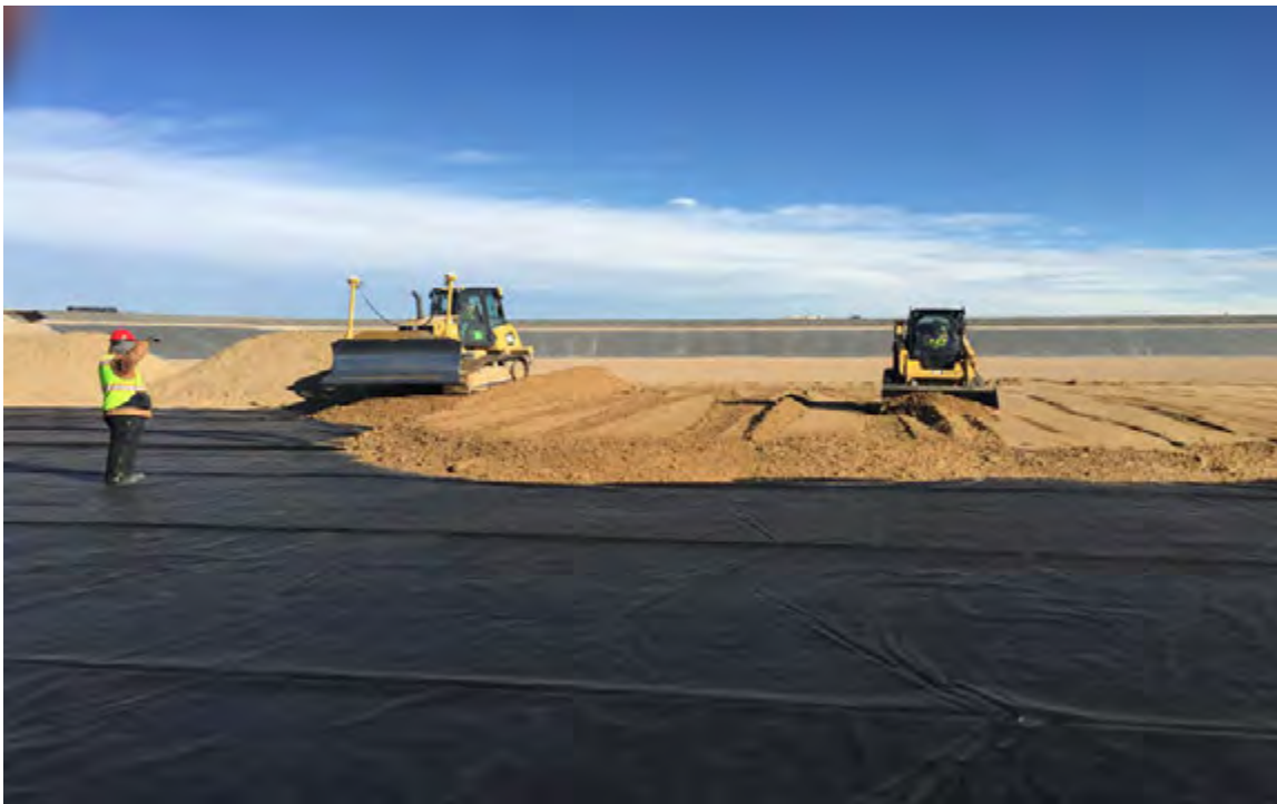
Figure 4. Photo showing cover soil placement by GPS guided LGP dozer and tracked skidsteer. Note minimal wrinkling or waves during placement
