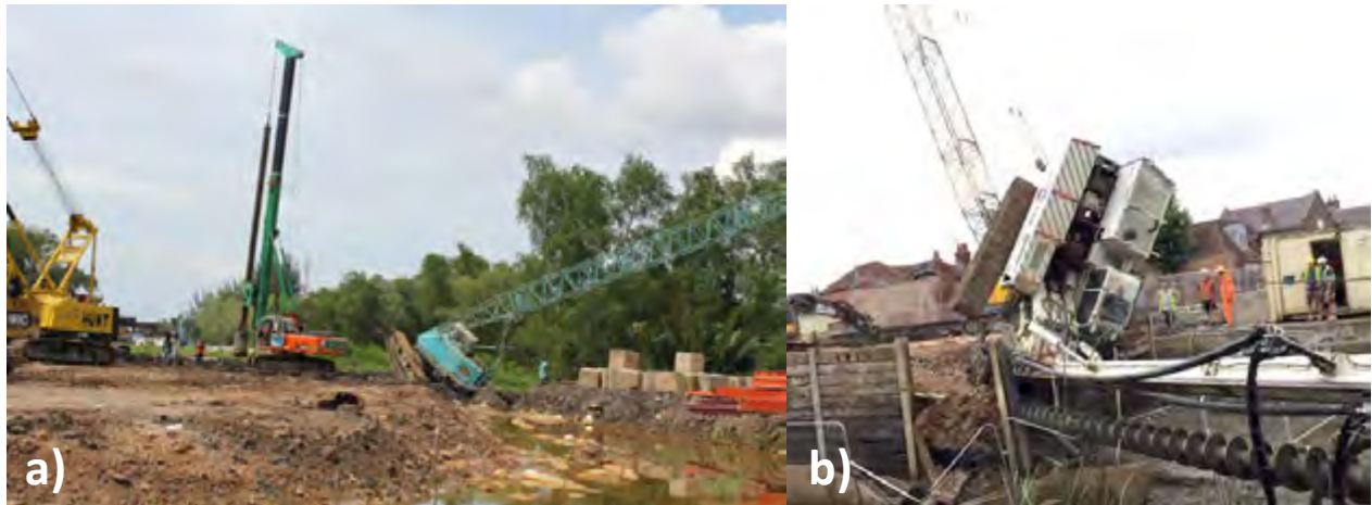
Figure 1. Examples of piling rig accidents: a) overturned due to soil low bearing capacity of working platform in Germany 2018; b) at quay in Emsworth, Australia at 30th July 2019
