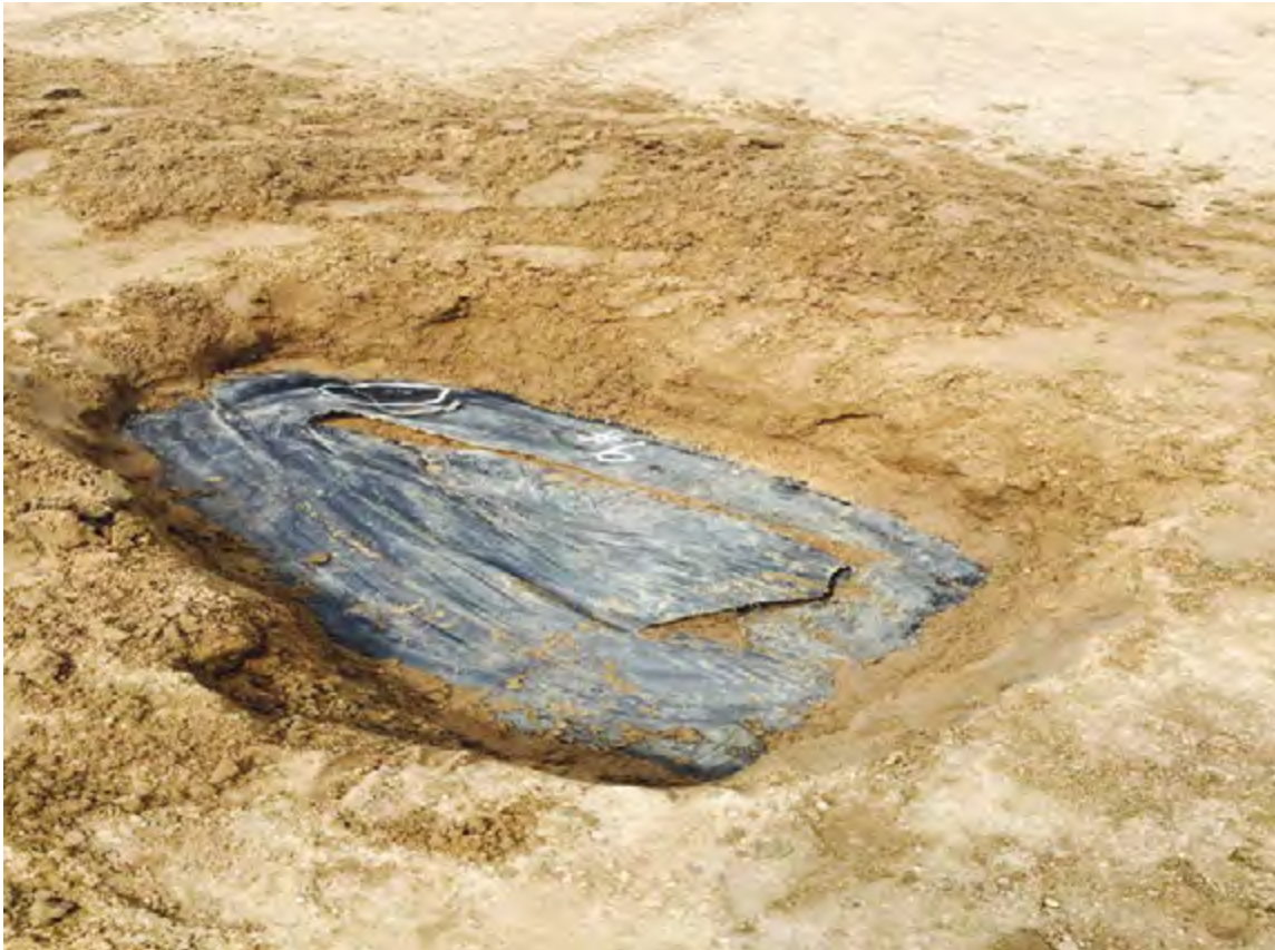
Figure 5. ELLS photo showing significant damage due to contractor equipment during cover soil placement on bottom lining system.
