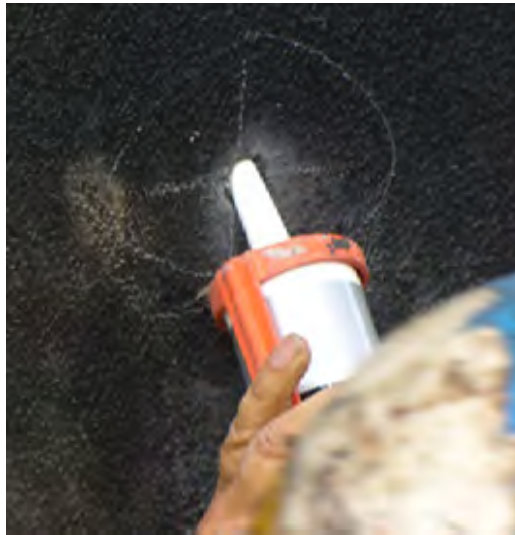
Photo 2. Untrained installation performing improper HDPE repair using caulk.
