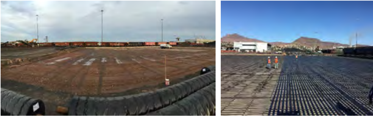
(a) (b) Figure 3. Preparation of the site (a) and geogrid installation (b).
