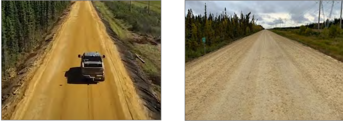
Figure 7. Final road structure immediately after construction (left) and after one freeze-thaw cycle (right).
