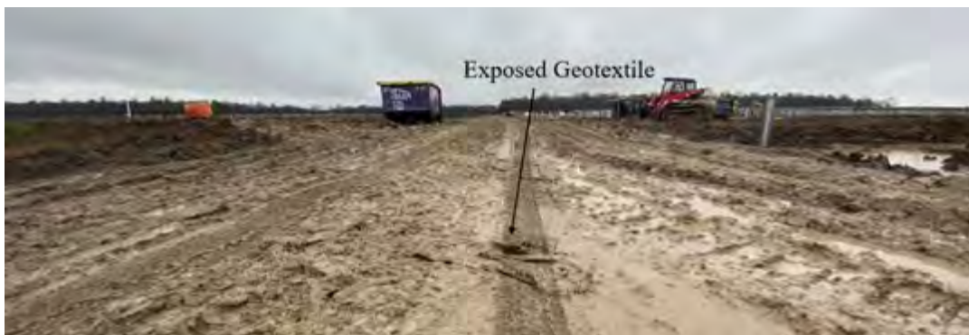
Figure 7. Exposed Geotextile Caused by Unanticipated Use of Access Road
