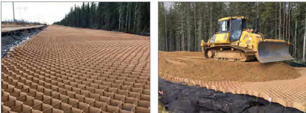
Figure 4. Stretched NPA geocell and non-woven geotextile separation layer (left) and placement of sand fill (right).
