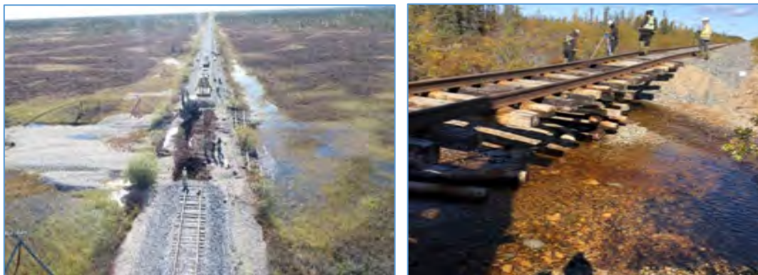
Figure 3. The condition of railway line after the flood event pictures from 2018.
