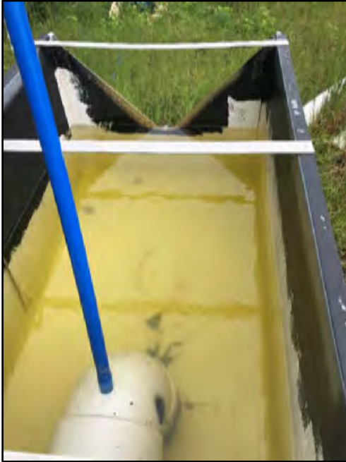
Figure 19. Effluent in Weir Tank
