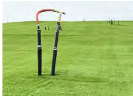
Figure 11. Landfill gas extraction wells integrated with engineered turf cover.
