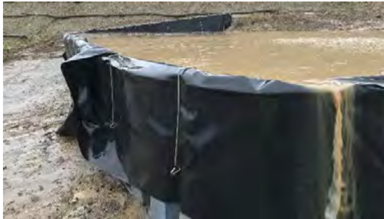
Figure 12: Basin MW-9 overtopping during a storm event.
