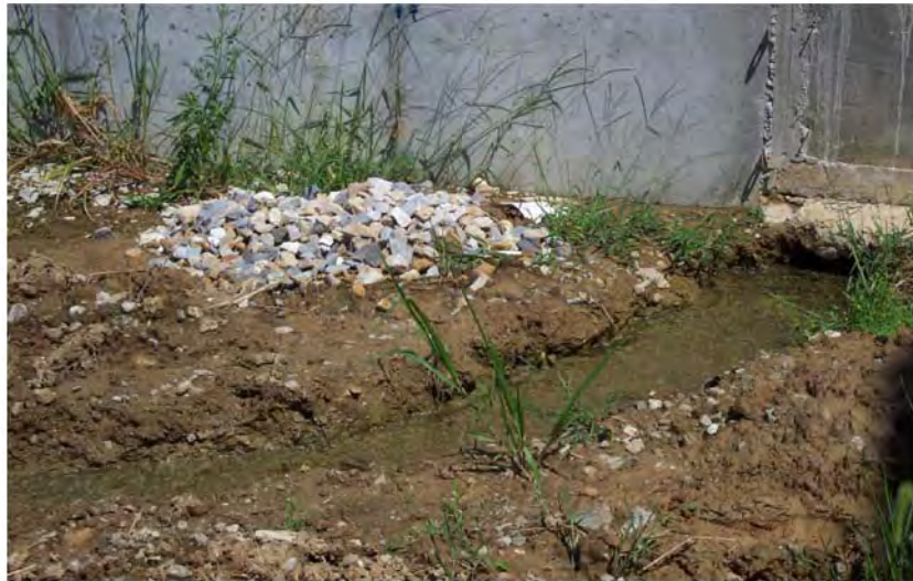
Figure 9 – Example of water in drainage excavation beneath footing
