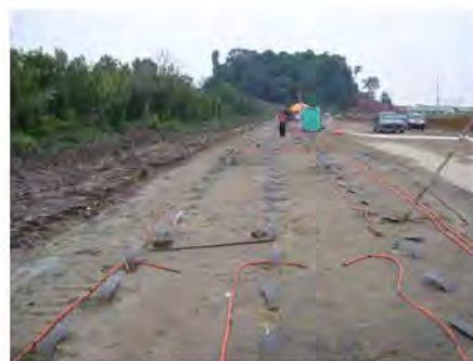
Figure 7: View of EVD with cables attached
