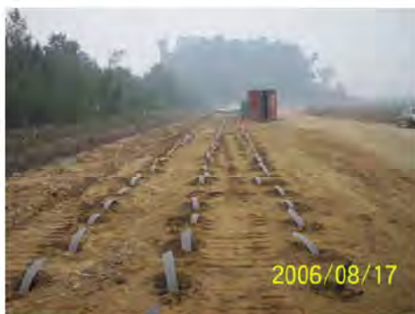
Figure 6: View of EVD installed
