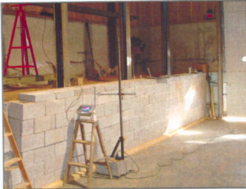
Figure 6 Completed segmental wall and fence posts prior to full-scale testing of the proprietary fence system. Instrumentation, hydraulic ram and the reaction frame can also be seen.
