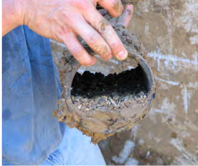
Figure 5 – Clogged existing perforated pipe drain along top of the concrete wall footing (July 17, 2006)
