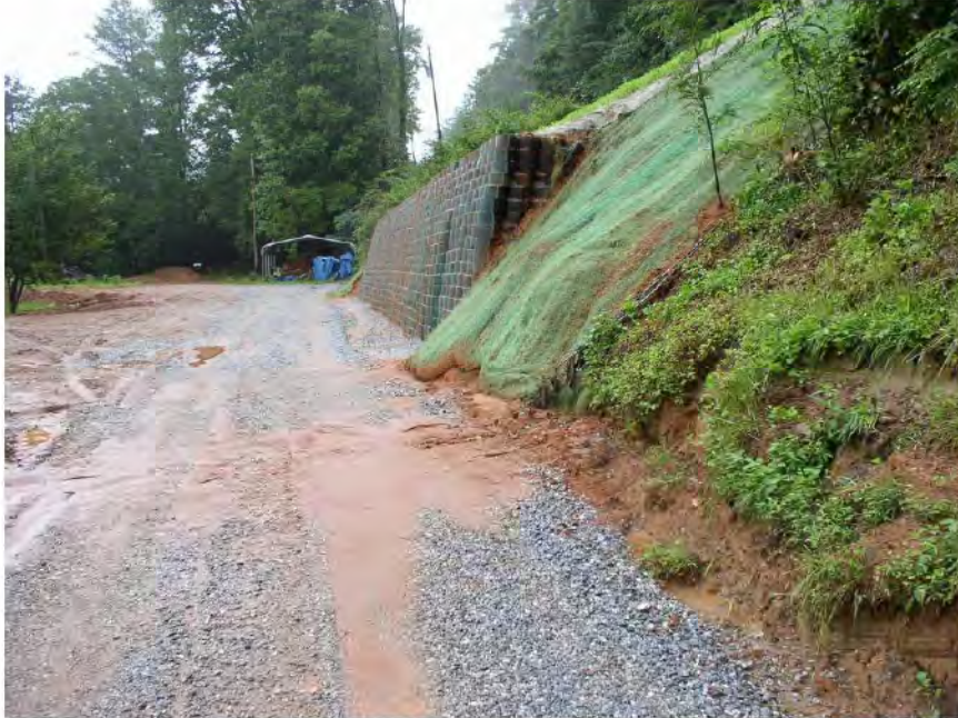
Figure 20 Slope Failure at the end of the Geocell Wall
