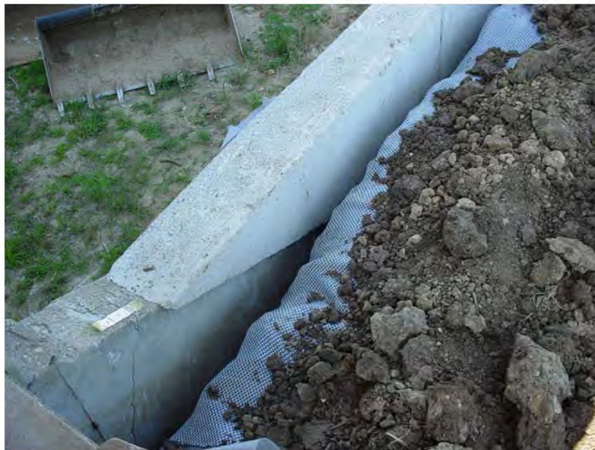
Figure 13 - Gap between concrete wall and geotextile wall in lift #9 (July 24, 2006)
