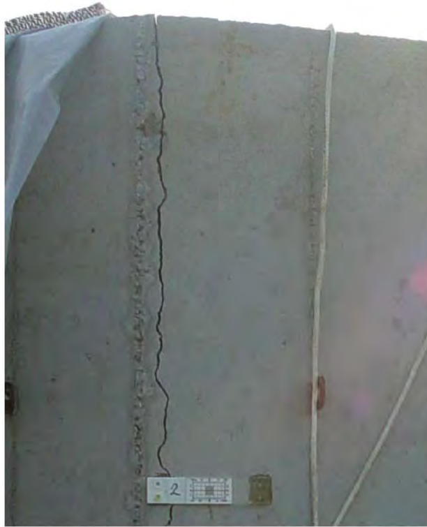
Figure 14 – Existing corner crack on concrete wall face with crack gauge (July 24, 2006)
