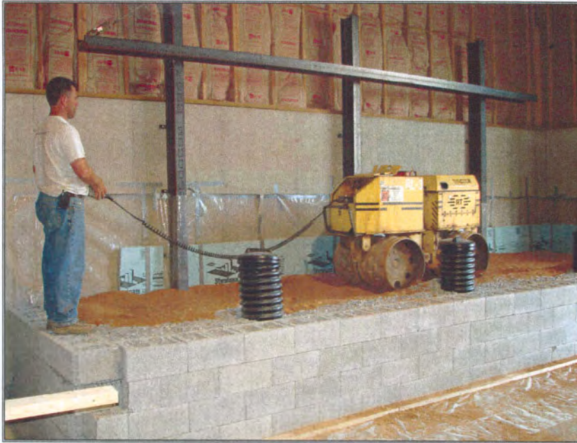
Figure 5 Compaction of soil backfill during full-scale testing of the proprietary fence support system. The fence supports can be seen in the foreground, placed directly behind the segmental blocks.
