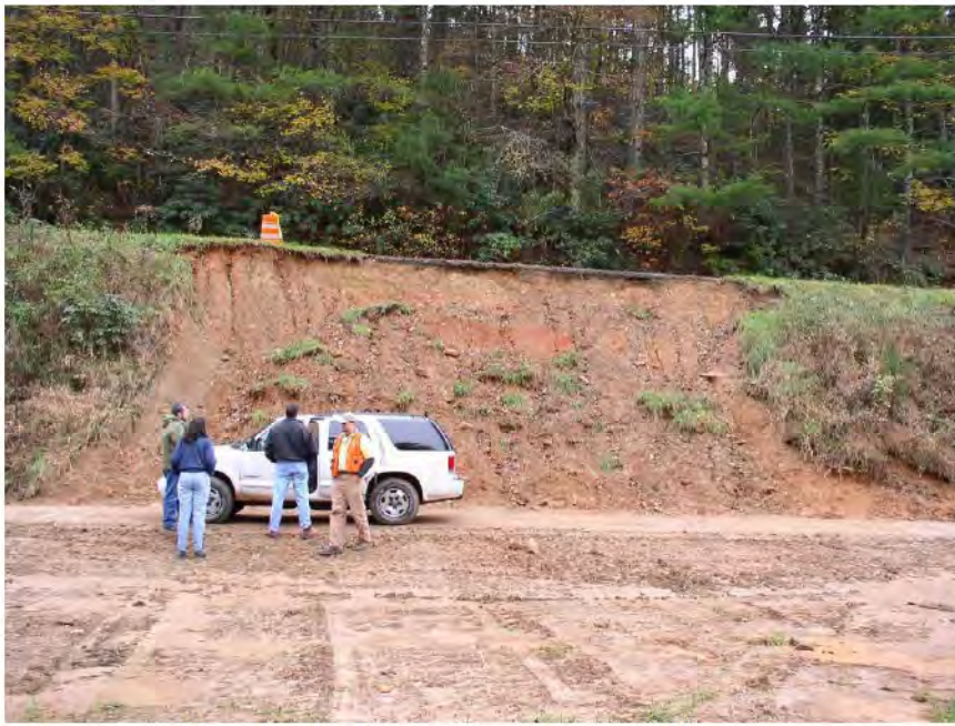
Figure 11 Rabun County EWP Site 3 Slope Failure
