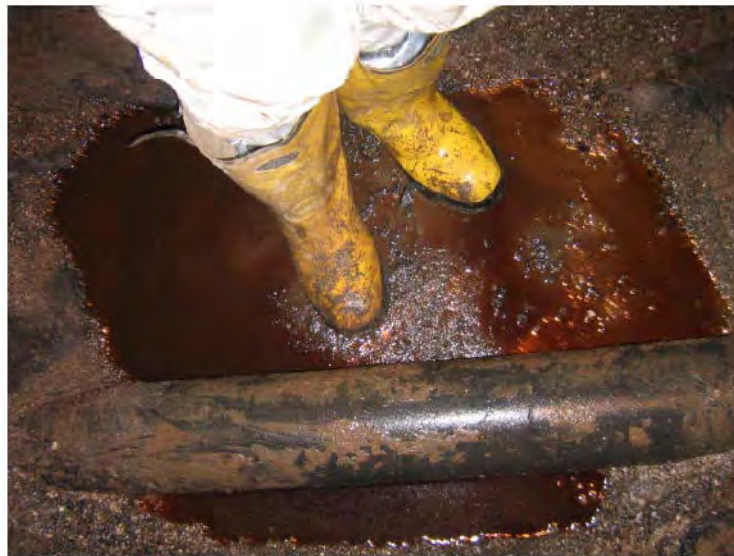
Figure 10. – Leachate collection pipe within shaft at D-14
