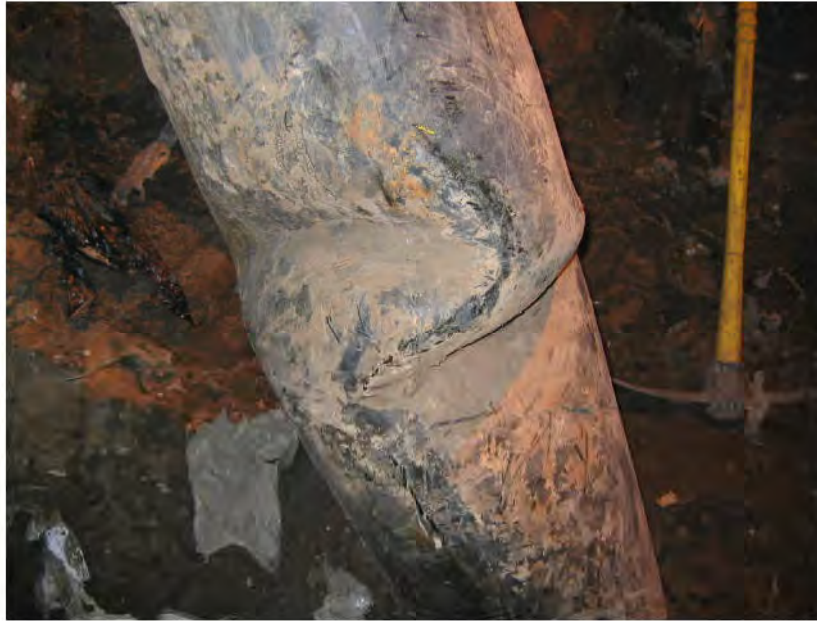
Figure 13 –Hand excavation around sub-cell A-North collapsed riser pipe
