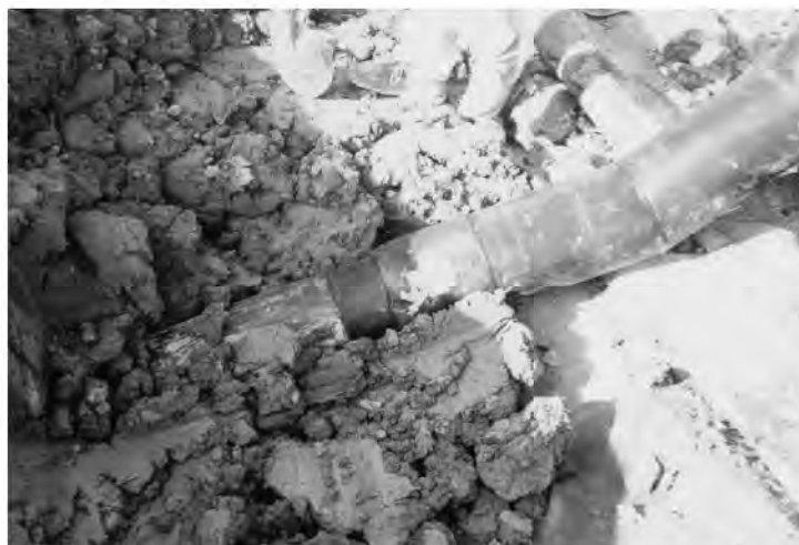
Figure 6. - Condition of bedding soil around elbow
