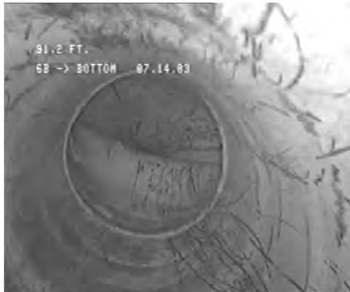
Figure 3. - Distressed elbow in Subcell B riser
